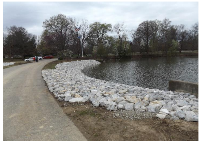
The beginning phases of the Grounds project included installing riprap rock around the main lake.
