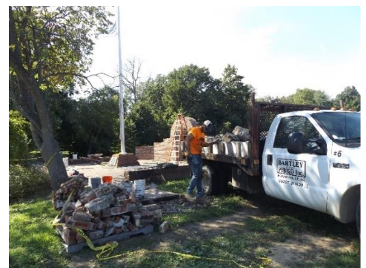
Contractor Christopher Schmitt is seen working on the Veterans’ Memorial near the campus lakes.
