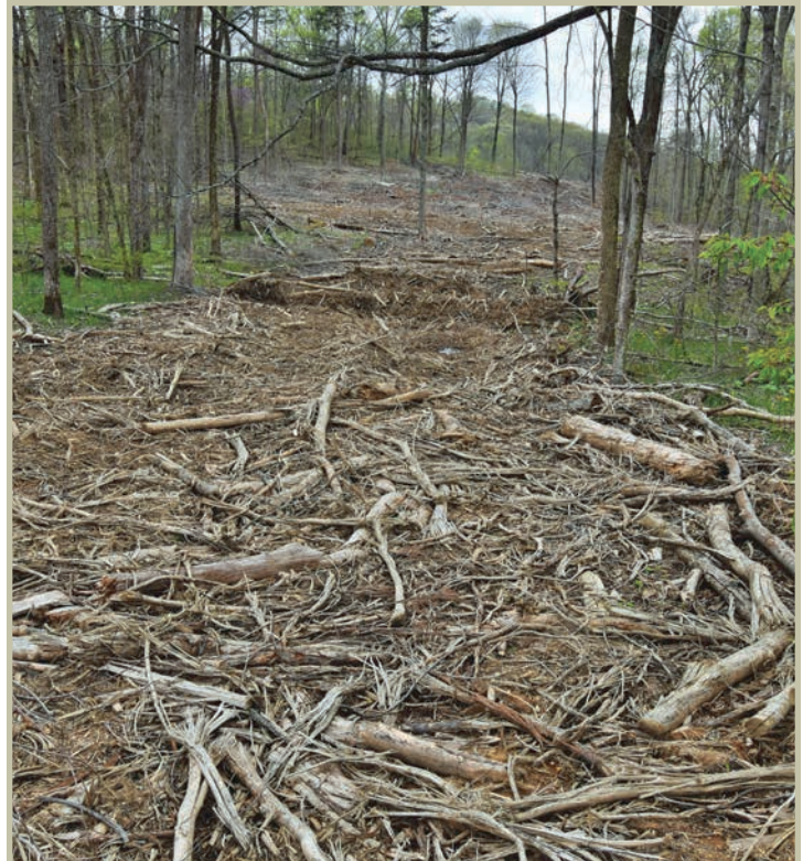
Use of debris to armor skid trails is a great practice to reduce erosion and close out skid trails.
