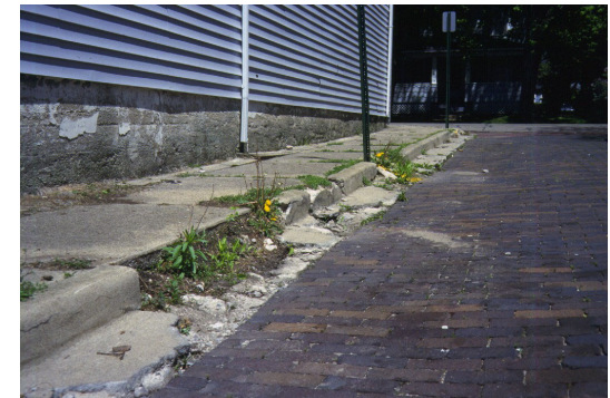
The curbs and sidewalks are deteriorating throughout the Town of Culver.
