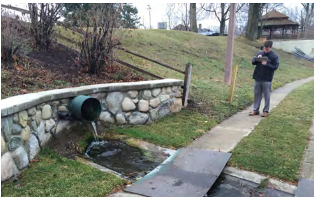
This drainage obstruction cuts across the path adjacent to the lake
