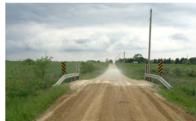
Bridge over a ditch on 20 A Road that will need to be widened to include a trail
