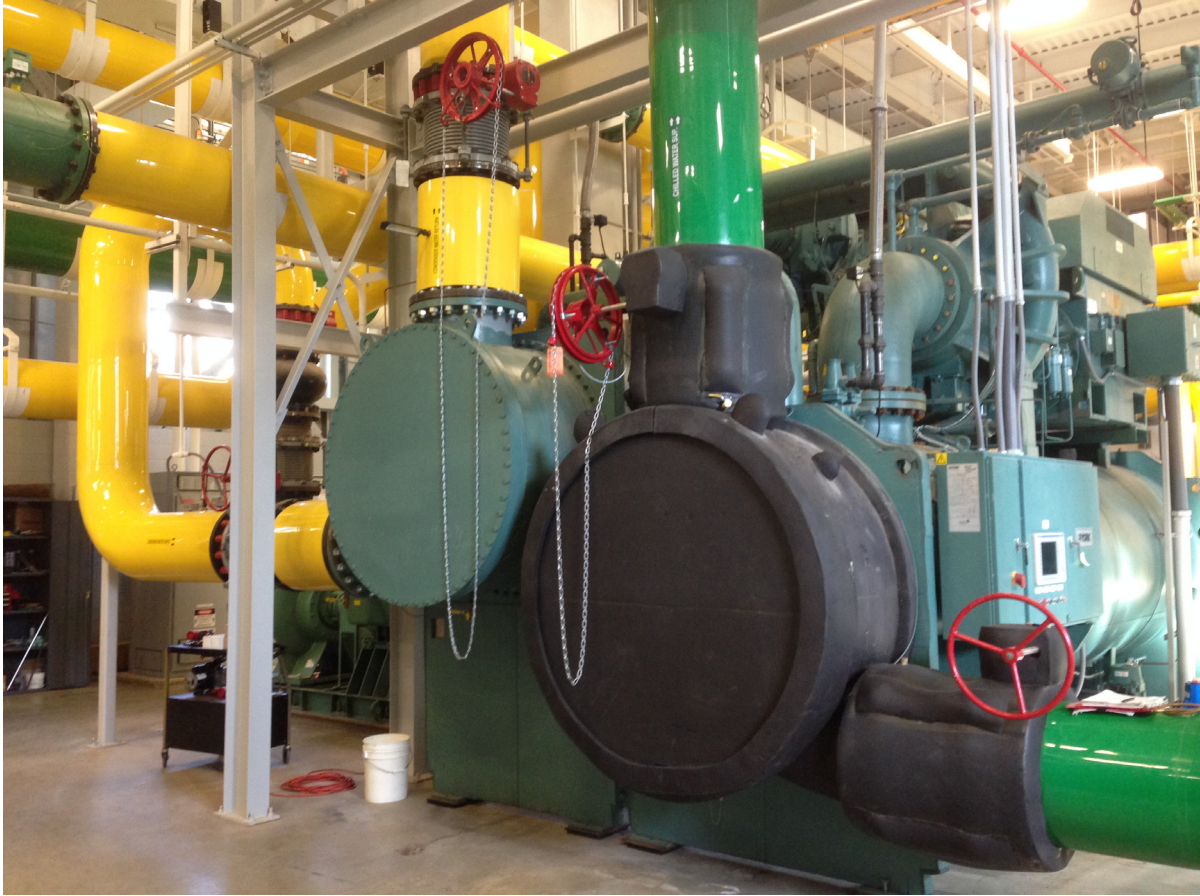
Geothermal heat pump chillers
