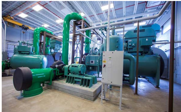
North District Energy Station
