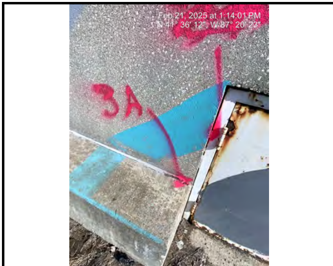
Sample #3 Exterior Caulk - Gray, flexible, at base of decorative concrete and exterior footings
