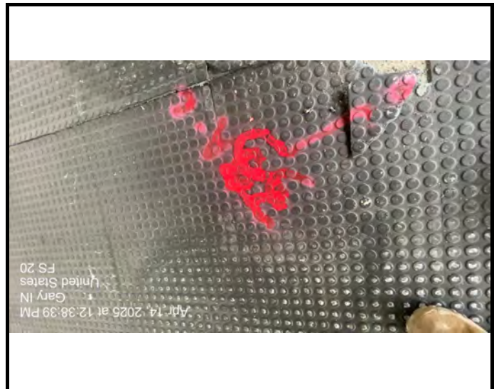
Sample #33 Rubber - Matting on SkyBridge flooring
