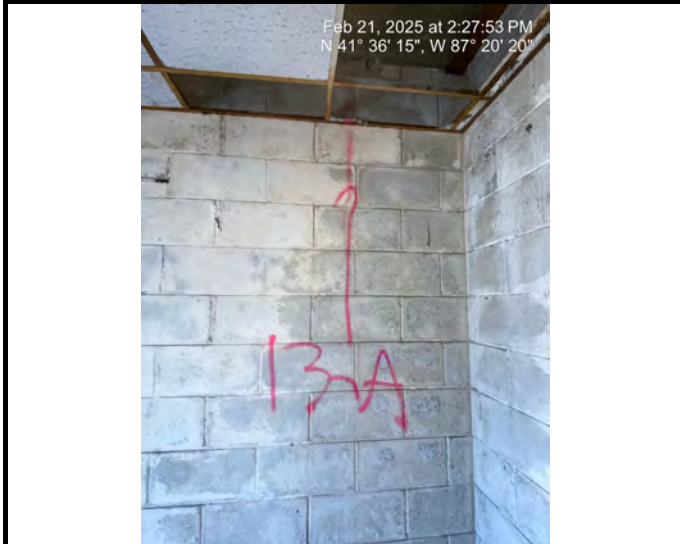
Sample #13 Ceiling Panel - 2X2, white, pinholes & fissures
