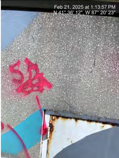
Sample #5 Exterior Caulk - Gray, brittle, at short metal doors
