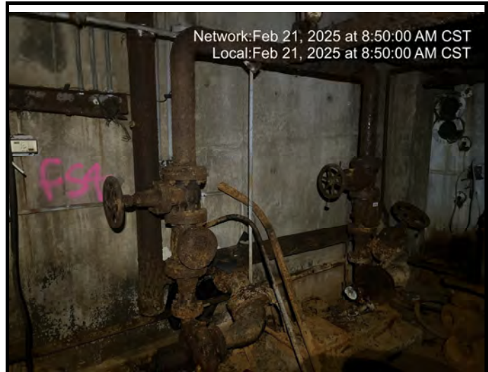
Assumed Material # A-6 Valve Packings - Various size valve packings
