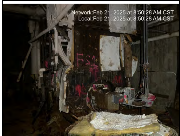
Assumed Material # A-4 Boiler Insulation - Internal boiler components including but not limited to; fire brick, gaskets, insulation, etc.
