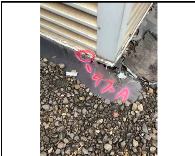
Sample # 47 Exterior Caulk-Light Gray - Around an Air Handling Unit perimeter and used as patching seams, Window
