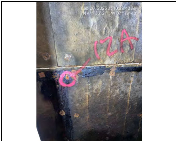
Sample # 12 Construction Adhesive - Black, on fiberglass insulation inside air handler
