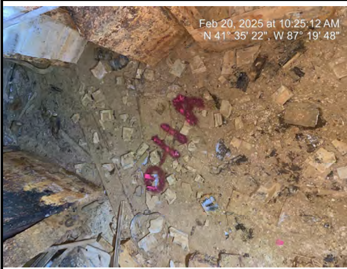
Sample # 11 Insulator - Transite debris, from electrical panels
