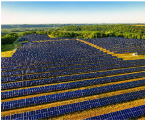
Figure 1. Solar Farm at Red Wing Minnesota
