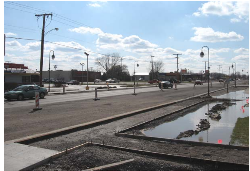
Pavement Rehabilitation and Repair: 133 rd Street from Wicker to Parish, Cedar Lake
