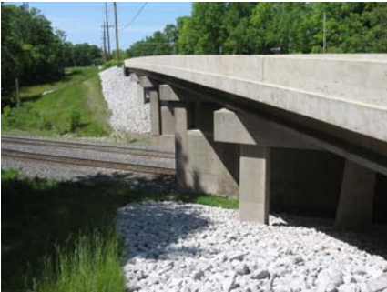
Bridge Rehabilitation or Repair: Calumet Avenue bridge over CSX railroad, South of Chesterton
