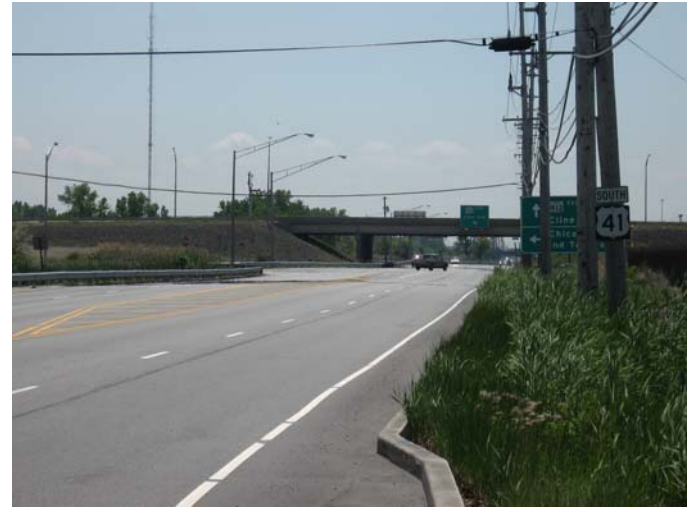
HMA Overlay: US 41 from 0.9 miles south of I-90 to 0.15 miles north of Sheffield, Hammond
