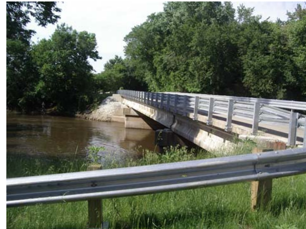
Bridge Rehabilitation or Repair: CR 50W bridge over Kankakee River, Porter County
