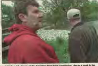
Bob Coiffman, left, director of the Kankakee River Basin Commission, checks a break in the river's levee just west of County Road 425 West in Porter County with John Law of the St. Joseph County drainage board Friday while crews work to fix the break.
