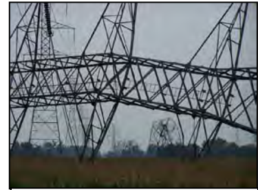
21 metal truss towers for power lines were toppled by 100-120 mph winds, Kouts, August 2007 Source: Weather Underground
