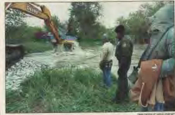
Bill Black saw a breach Friday in a levee in the Kankakee River levee when the Raylight Echon complex hit the river between Hobbs and DeKalb. Jim Hampton, left, Bob Coiffman, of the Indiana Department of Natural Resources, and Russell Perry visit the site.
