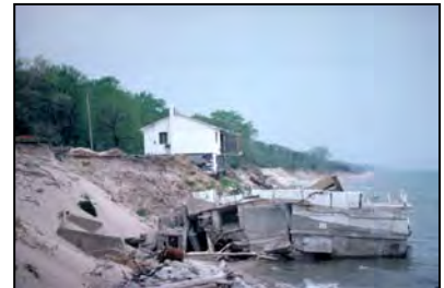
Shoreline erosion damages home in Ogden Dunes, Source: Michigan Sea Grant Extension , Carole Y. Swinehart
