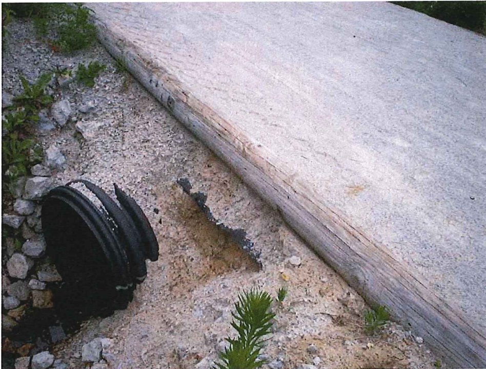
Photo 1 Stream crossing at sta: 18+75. Crossing needs extension
