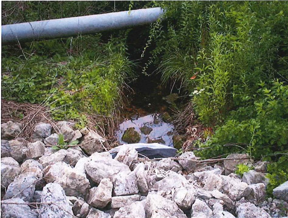
Photo 5 Stream crossing with exposed gas main.
