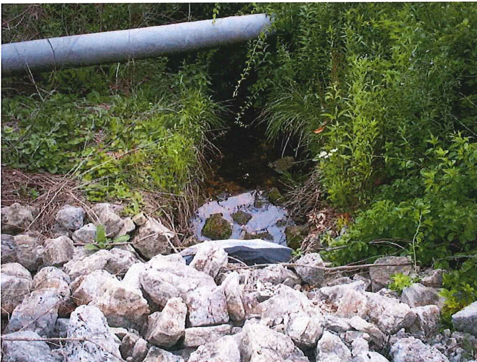
Photo 2 Stream crossing with exposed gas main.
