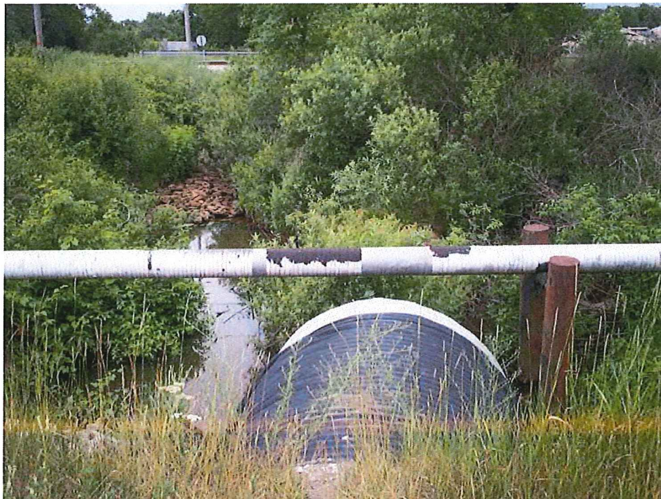
Photo 6 Culvert at sta: 524+20 needs erosion control, excess fabric should be removed. Exposed gas main.
