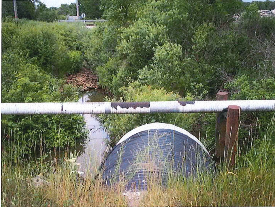
Photo 3 Culvert at sta: 524+20 needs erosion control, excess fabric should be removed. Exposed gas main.
