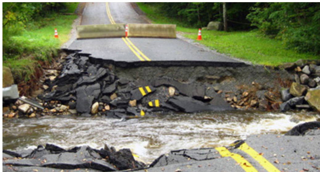
Culvert washout at Walker Brook in Becket, Massachusetts
