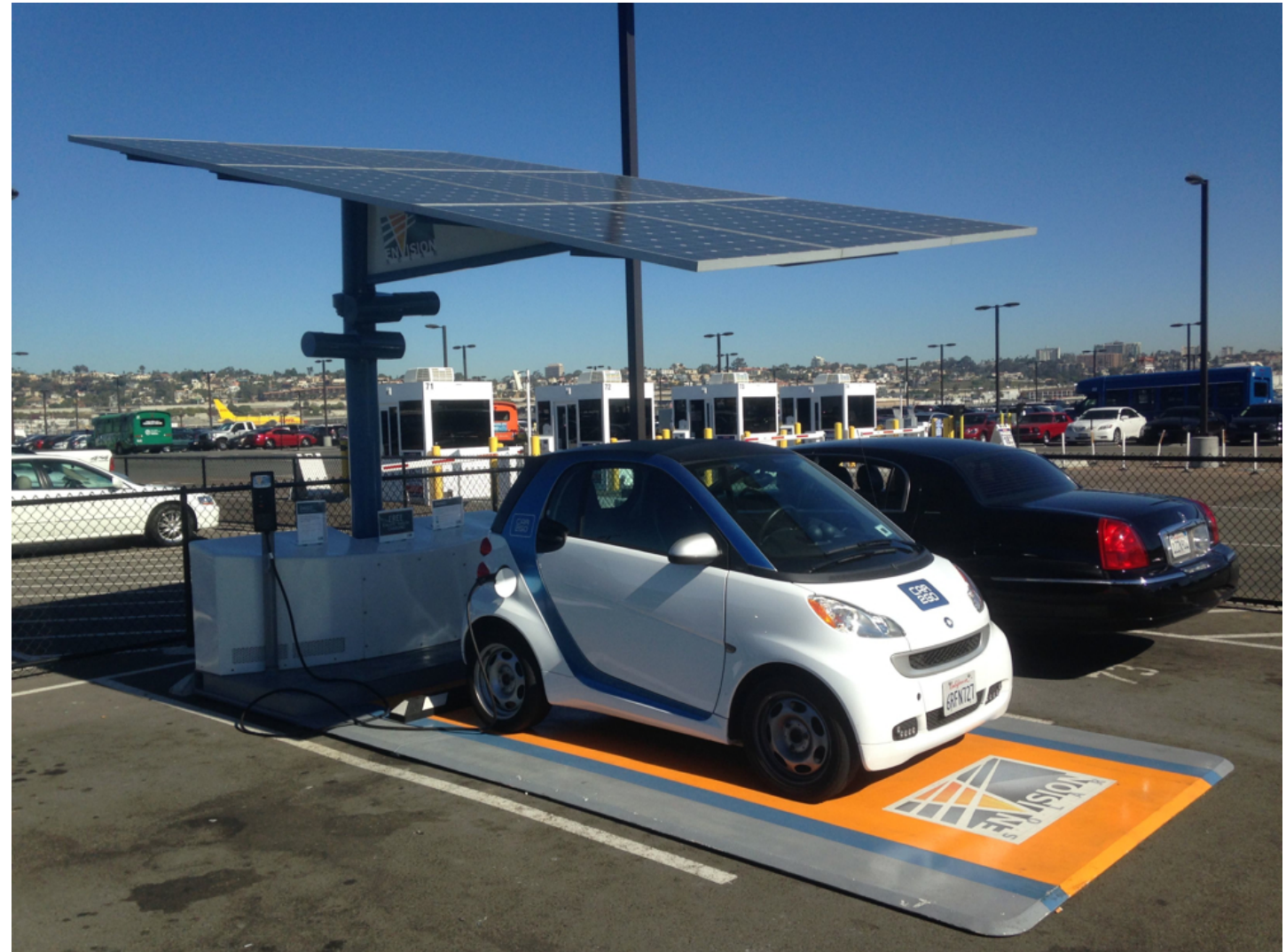
Envision Solar EV ARC solar powered charging
