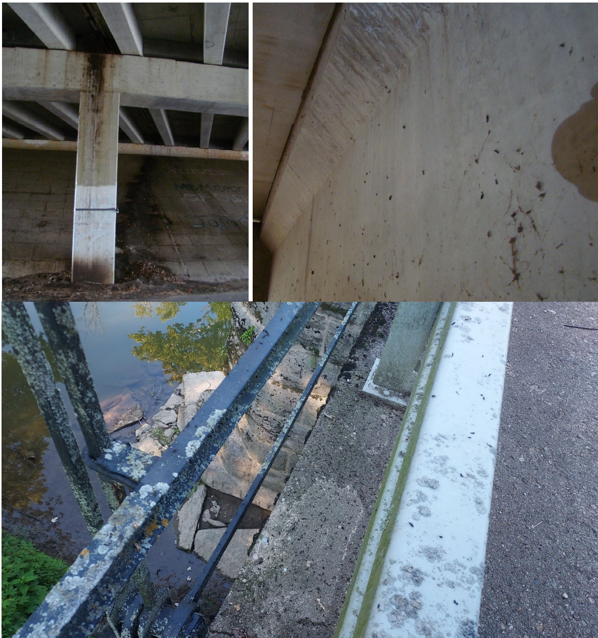
Figure 12. Examples of guano accumulations on bridges. (photos provided by Georgia Department of Natural Resources (top) and Indiana Department of Transportation (bottom)).
