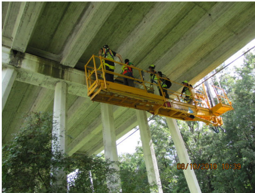
Figure 14. Biologists use a snooper truck to assess expansion joints and concrete caps over deep water (photo provided by Georgia Department of Transportation).
