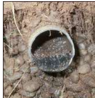
Lateral line clogged with solids (Photo from www.KingCounty.gov )
