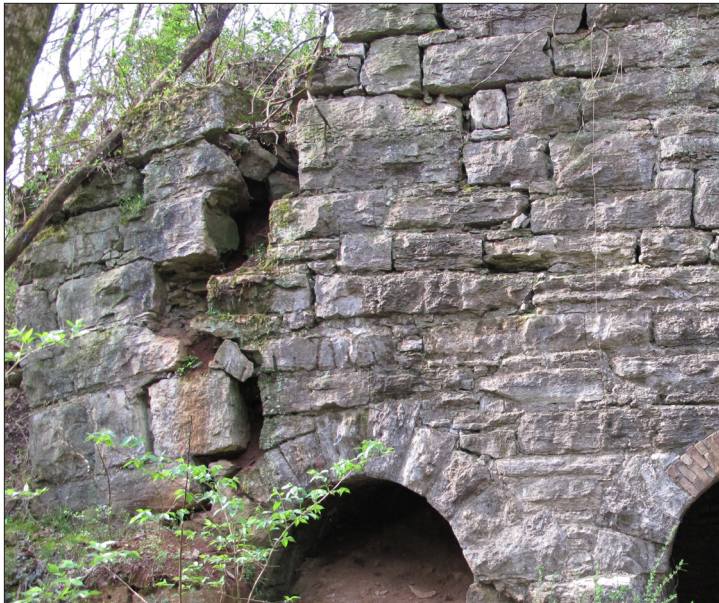
Damage to stone wall
