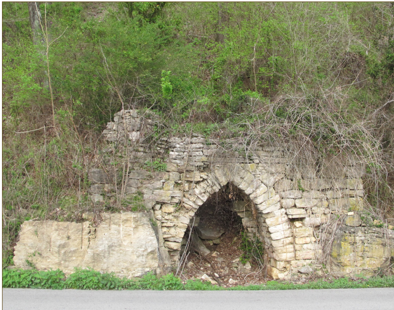
Current view showing extent to which the facade has been buried
