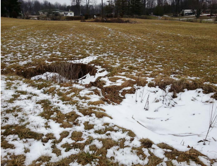
Photo 13: A-06, 2 small sinkholes, which swallow overflow from adjacent pond, both approximately 6' diameter, 3' deep.
