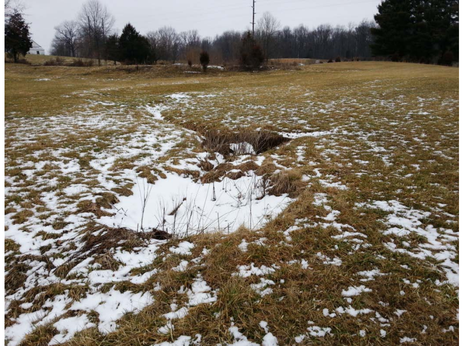
Photo 12: A-06, 2 small sinkholes, which swallow overflow from adjacent pond, both approximately 6' diameter, 3' deep.
