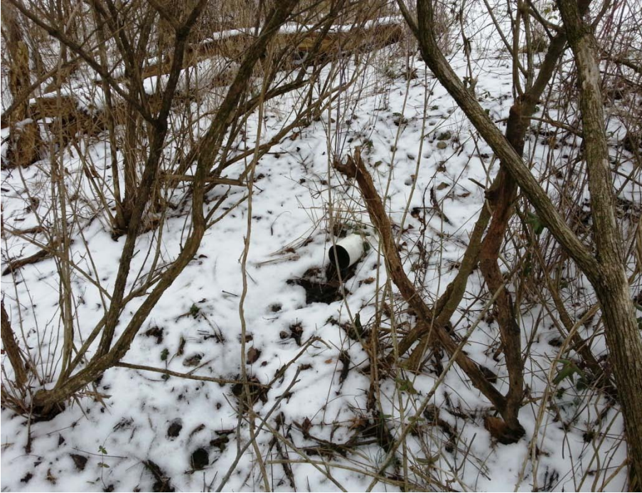
Photo 141: E-26, PVC draining into a large sink approximately 30' diameter, 6' deep.
