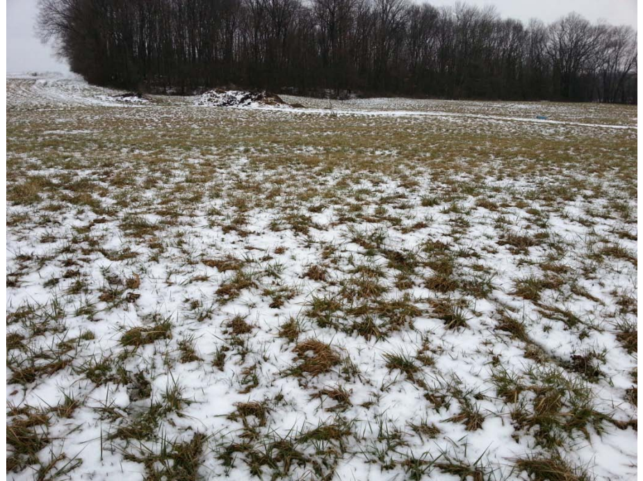
Photo 64: D-02 & D-03, Area surrounding 3" diameter open holes with no significant depression.
