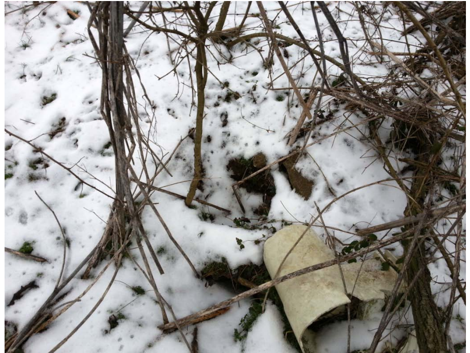
Photo 58: D-01, Swallow hole in a broad, shallow sinkhole, approximately 30' diameter, several feet deep. Debris is near swallow hole.
