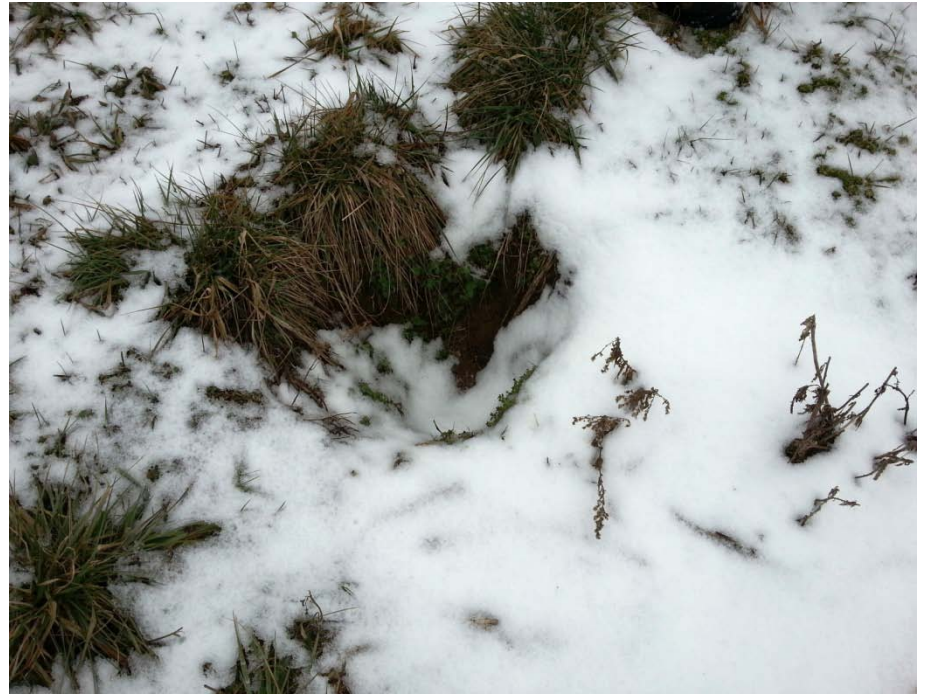
Photo 60: D-02 & D-03, open holes with no significant depression.
