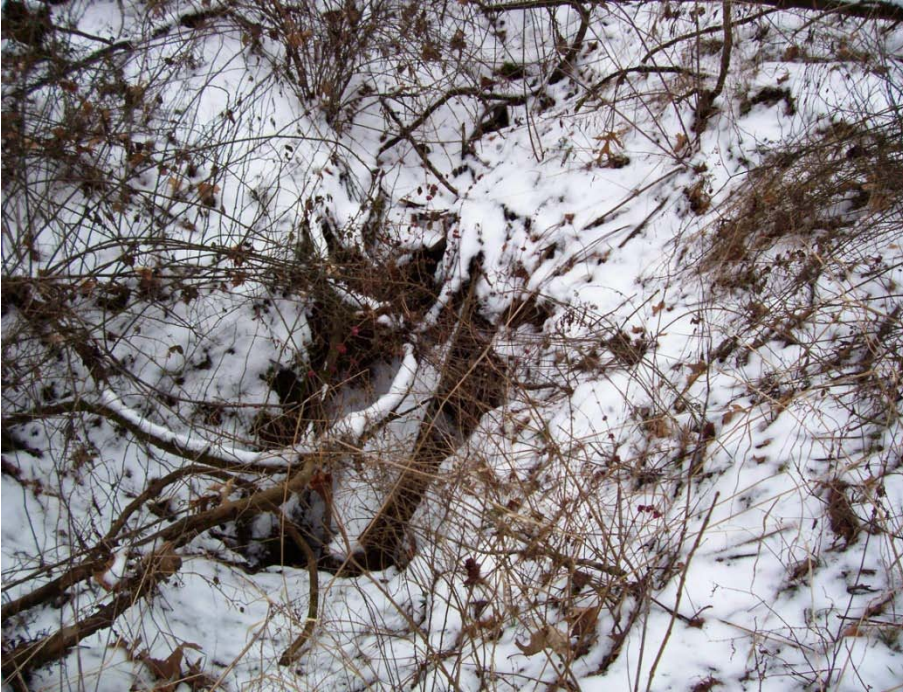
Photo 87: E-04, 15' x 25' sinkhole, approximately 5' deep. Corrugated (tin) roofing panels embedded in bottom.
