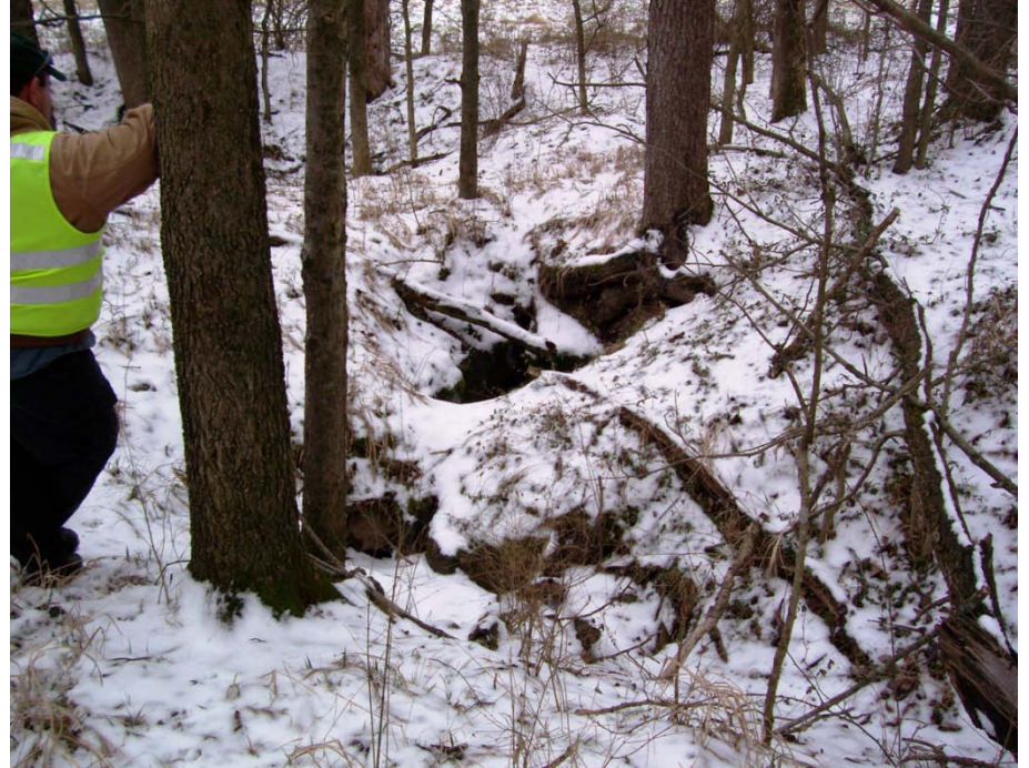
Photo 68: D-08, 20' x 10' sinkhole with 2 inlets.
