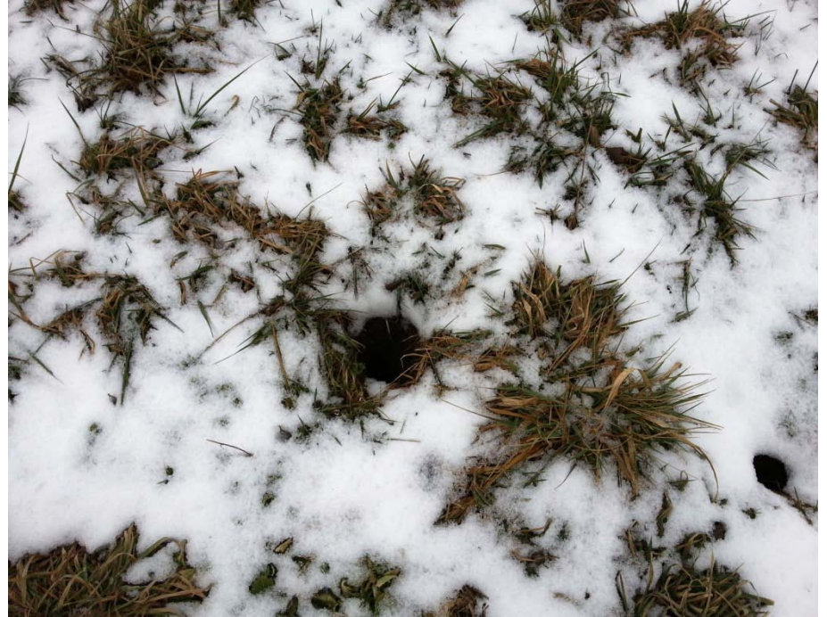
Photo 62: D-02 & D-03, 3" diameter open holes with no significant depression.
