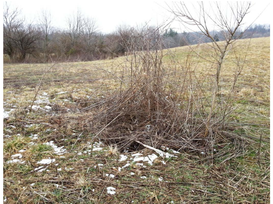
Photo 52: C-07, Distinct sinkhole approximately 10' x 15' x 4' deep with accumulation of sticks.
