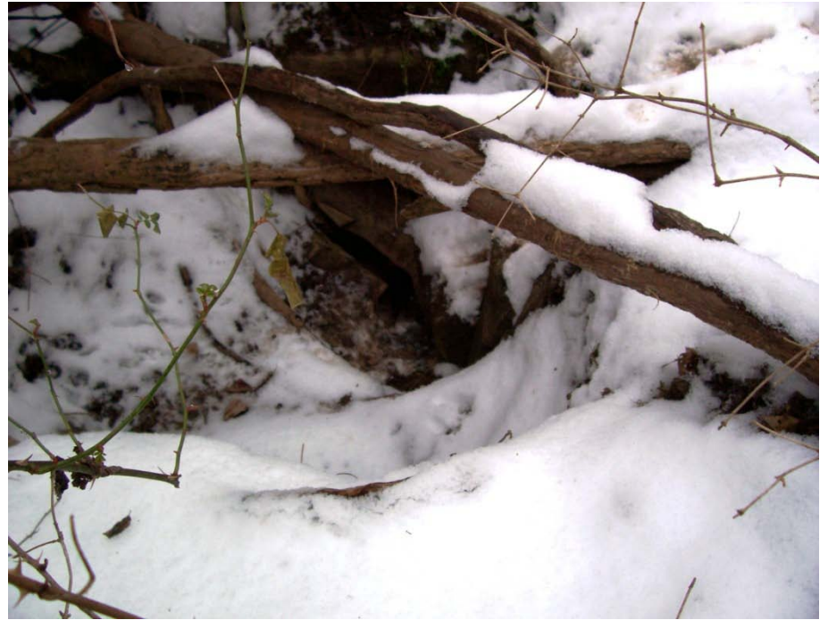
Photo 110: E-13, E-14, E-27, E-28, E-29 & E-30, Swallow hole in major sink with multiple openings. Basin is approximately 80' diameter, 10' deep.
