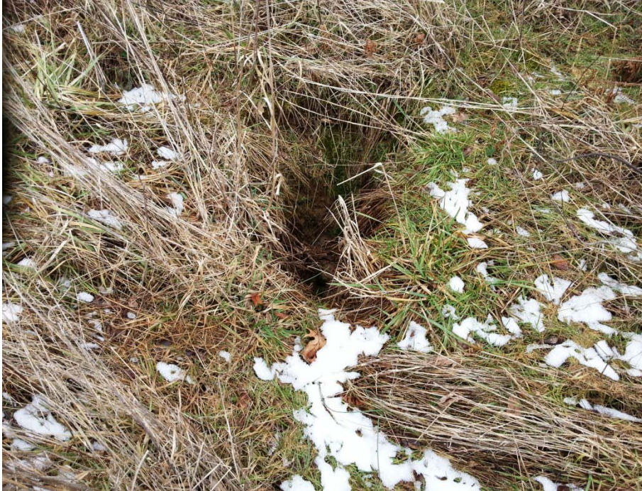
Photo 39: C-03 & C-T2, Swallow hole within large broad silt filled sinkhole with several distinct 2' diameter x 2' deep swallow holes approx 80 long x 40' wide with 5' total depth.
