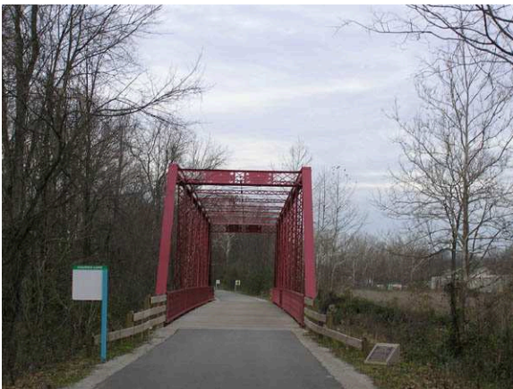
(35104) - Harris Ford Bridge and Interpretive Signage Looking North on Clear Creek Trail
