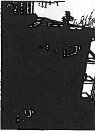
(11) Brick deterioration on the South Elevation. Outlines of the removed electrical conduit and meters are visible.
