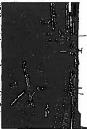
(17) View east showing south parapet of Ice Cooler area. Copings remain in poor condition.
