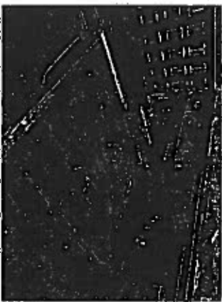
(18) View of roof over remaining South Dock office areas. Ponding water is visible.
