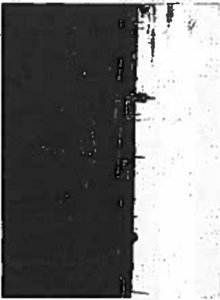
(15) Roof condition at north roof area looking northeast showing poor roofing condition and vegetation growth.
