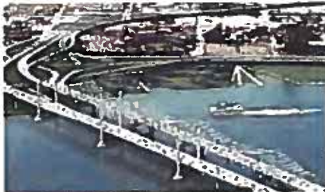
The new Downtown Bridge (left) is being constructed next to the existing Kennedy Bridge to alleviate traffic congestion and make travel safer.
