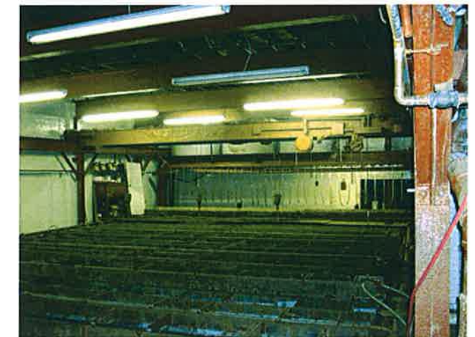
Ice Tank Room (View looking South)
