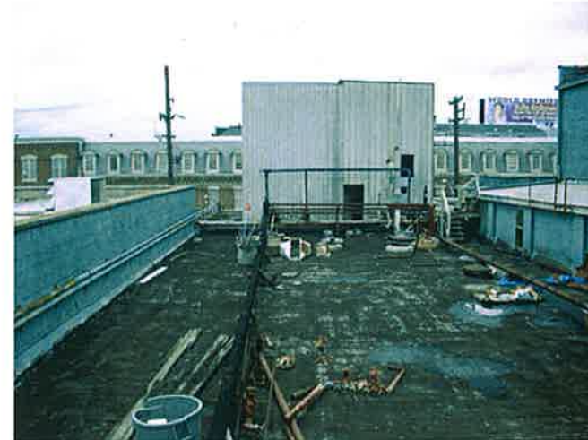
Debris on Ice Tank Room Roof looking South
