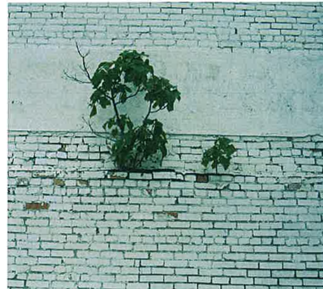
Deferred Masonry Repair -- Tree Growing from Brick Ledge
