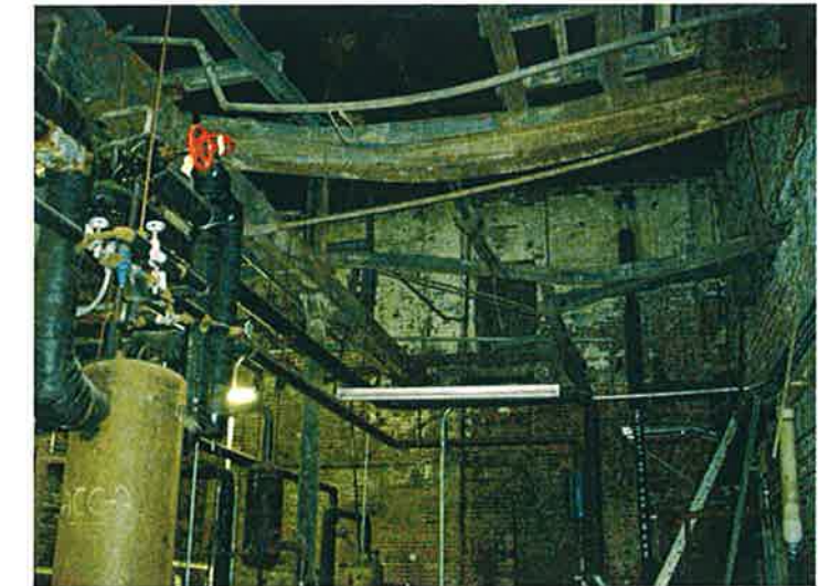
Mechanical Room A
