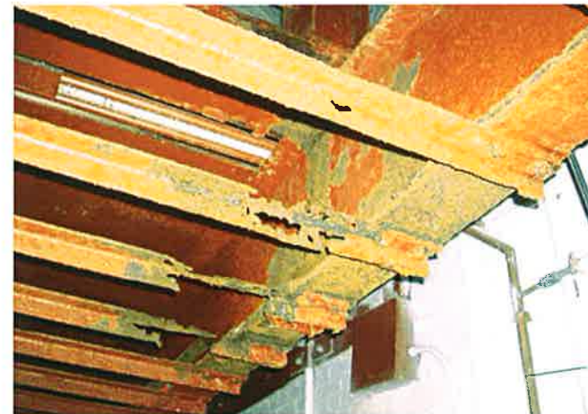
Deteriorating Steel at Ice Tank Room
