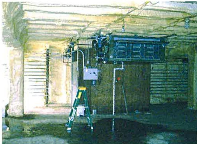
Newer Ceiling-Hung Mechanical Unit at Cooler E, Third Floor (Elevator and Former Refrigeration Piping Beyond)
