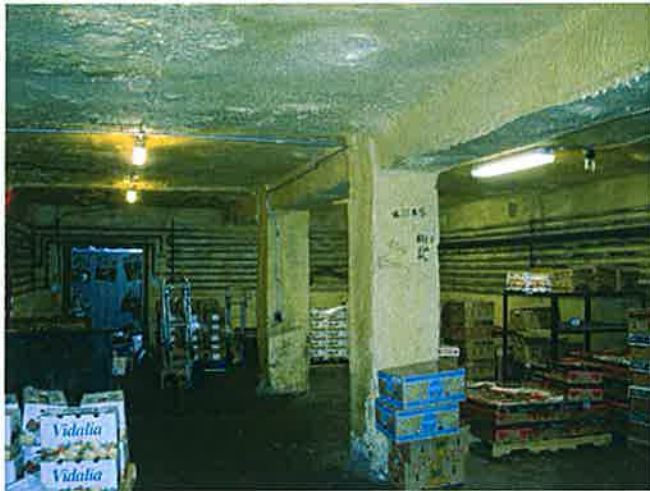
Cooler F looking North
