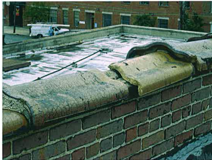
Clay Tile Coping Deterioration
