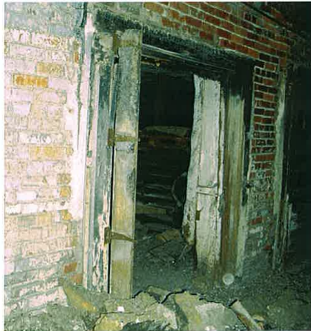
Fire Damage at Cooler G, Third Floor
