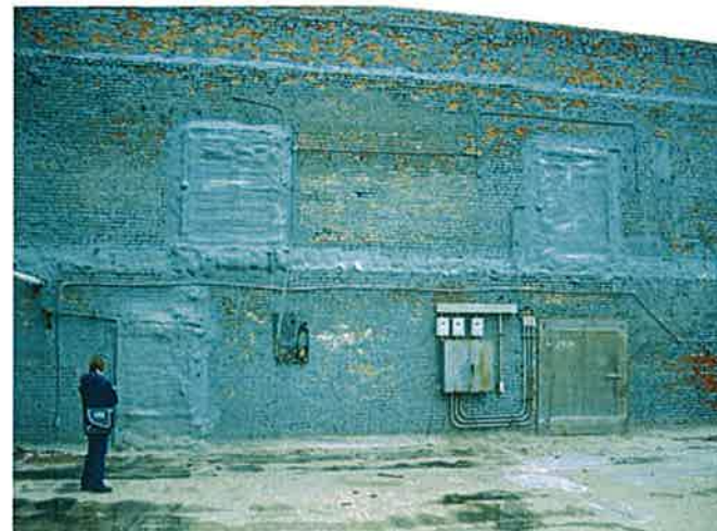
West Elevation of Cooler E at Roof Level of Former Tank Room
