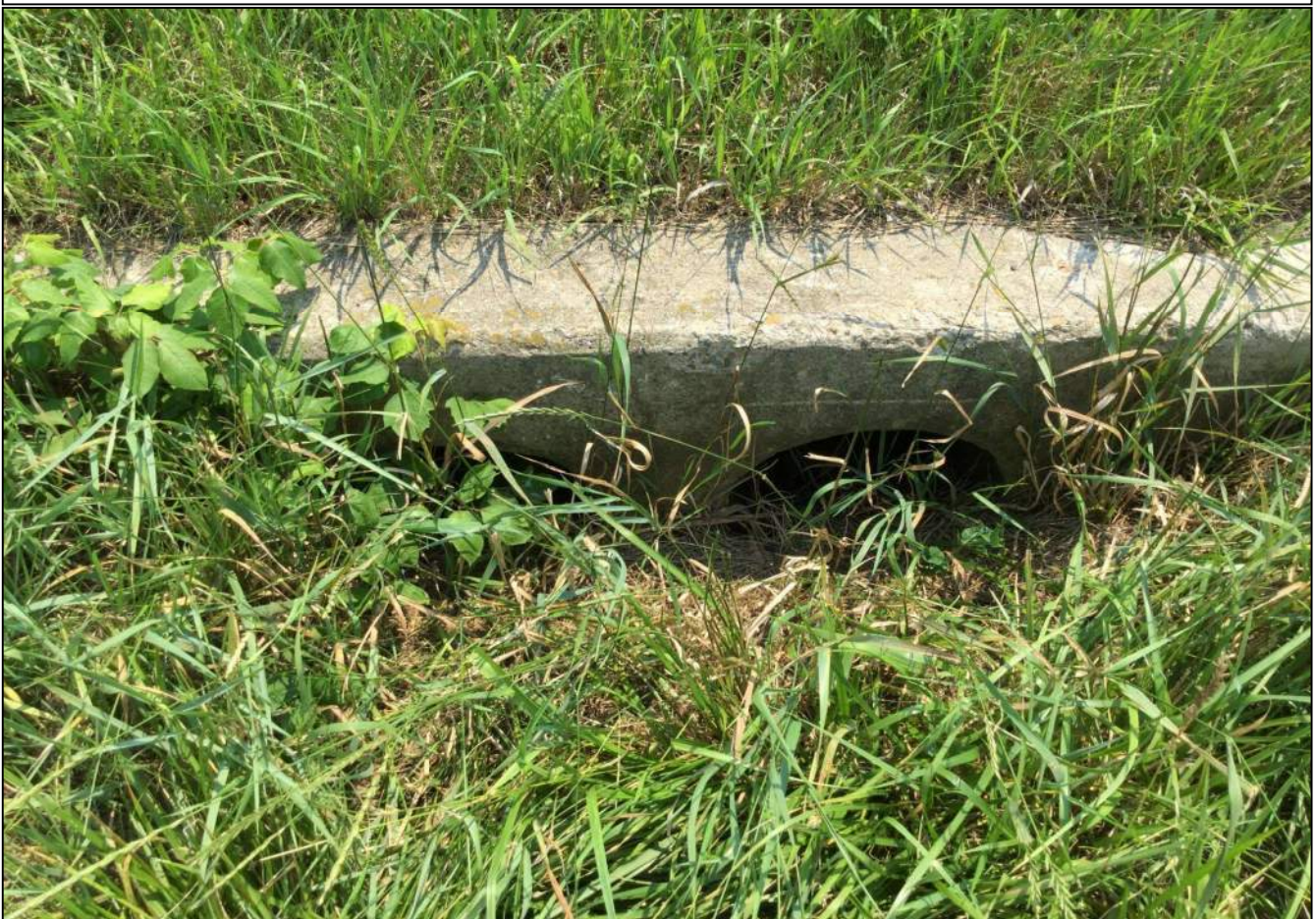
150. Looking south at Structure No. 121 located along the north side of SR 32. No stream or wetland features were observed. Photo taken July 6, 2021.
