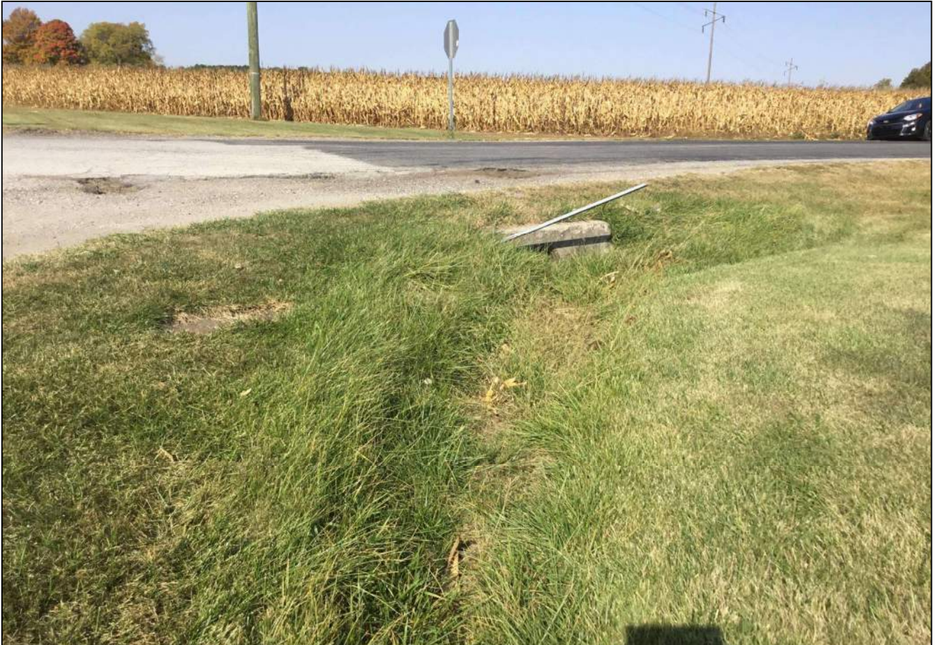
80. Looking northwest along the north side of SR 32 and at CR 500 W. Please note the concrete headwall for a small diameter culvert pipe that conveys drainage underneath CR 500 W. Photo taken October 7, 2020.
