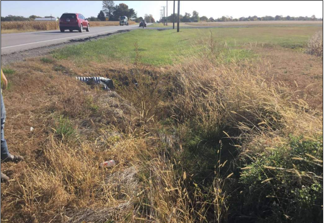
168. Looking east along the south side (EB lane) of SR 32 just southwest of Structure No. 111. No stream or wetlands were observed. This structure will be replaced as part of this project. Photo taken October 8, 2020.
