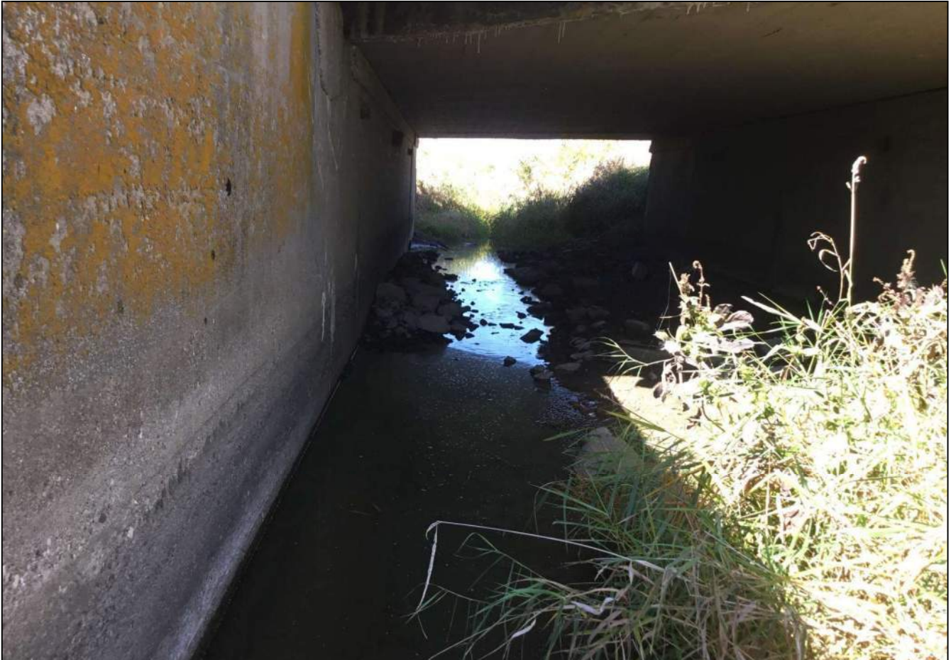
122. Looking northwest (downstream) Little Sugar Creek underneath structure CV 032-006-53.90. Photo taken October 8, 2020.
