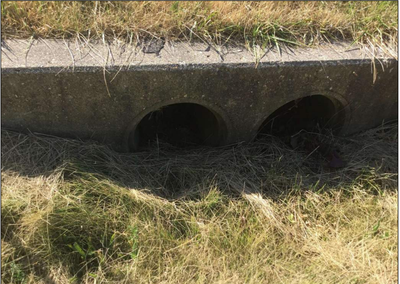
74. Looking south/southwest at a double barrel culvert located on the north side of SR 32. Photo taken October 7, 2020.
