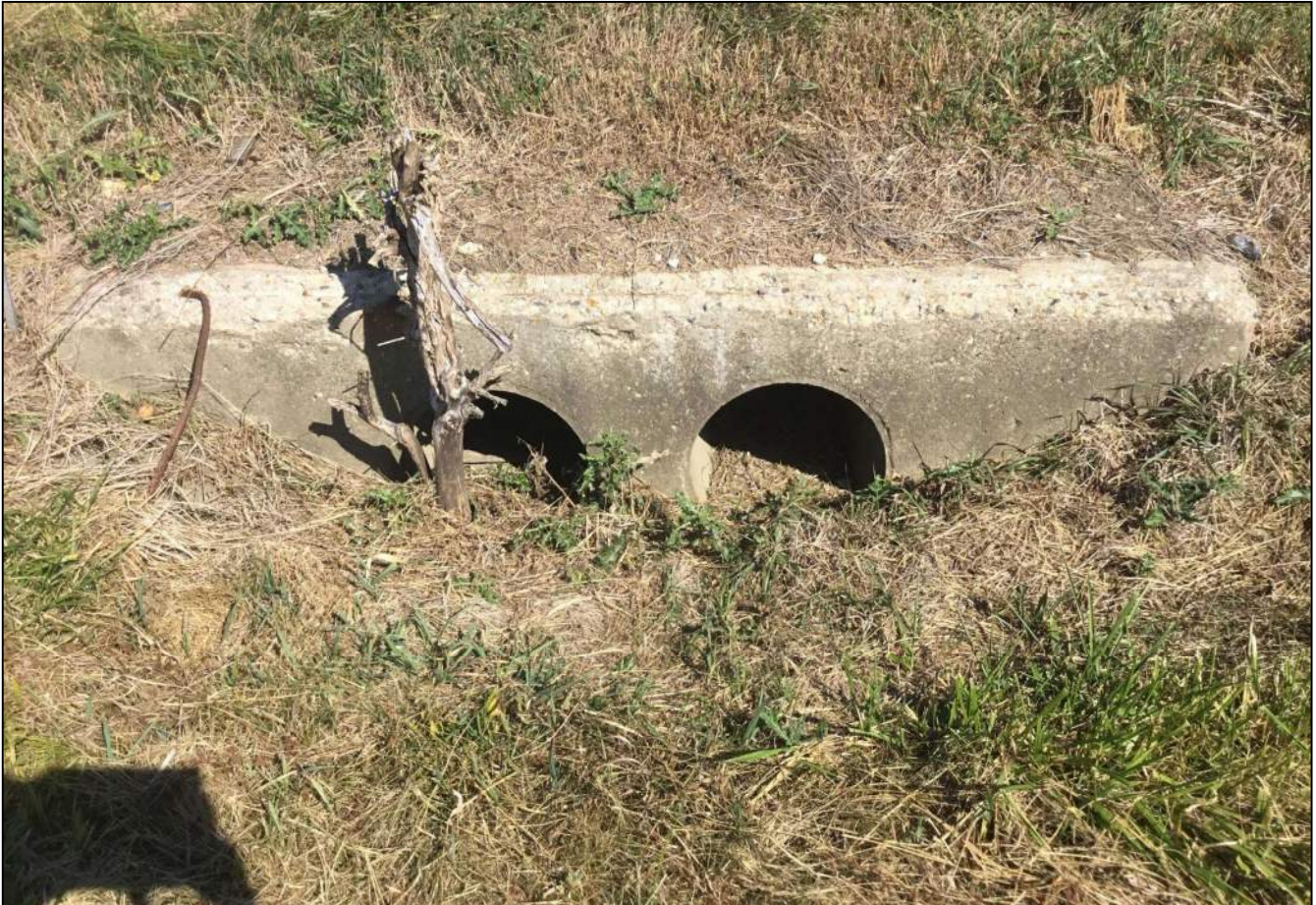
72. Looking north at a double barrel culvert located on the south side of SR 32. This structure will not be impacted as part of this project. Photo taken October 8, 2020.
