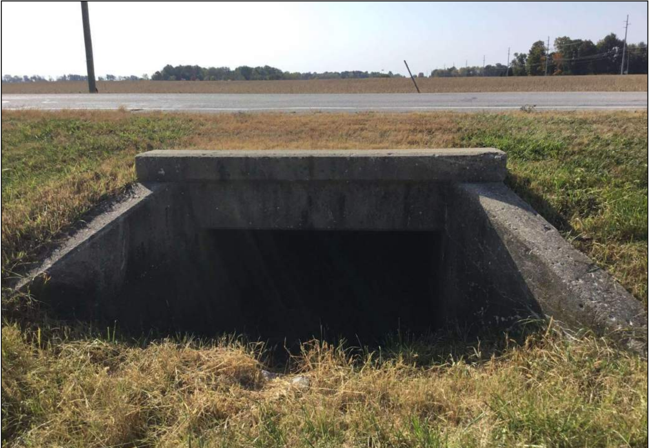
106. Looking south at CV 032-006-54.47 located on the north side of SR 32. No stream or wetland feature was found. This structure will not be impacted as part of this project. Photo taken October 7, 2020.
