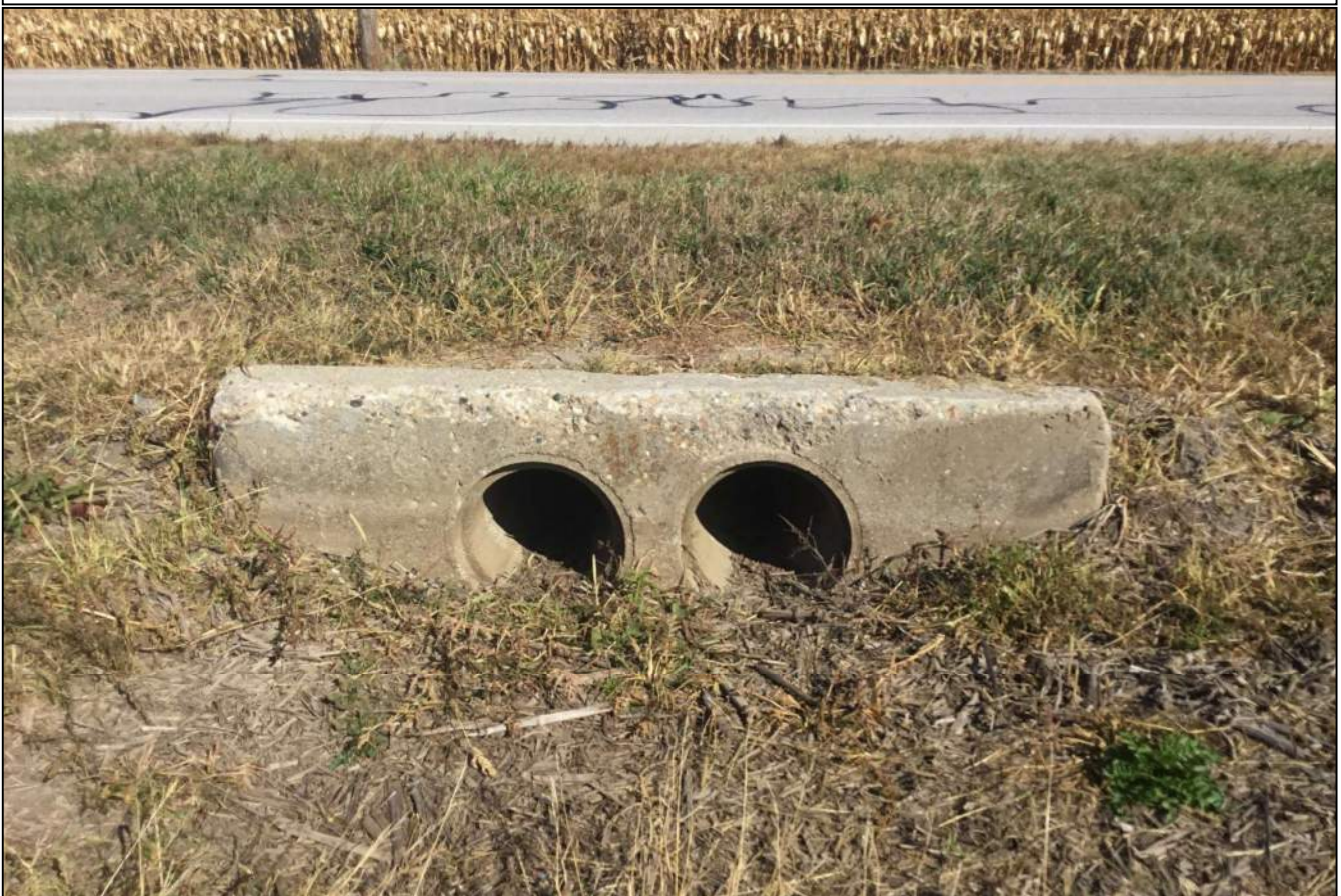
Looking north along the south side of SR 32 at Structure No. 123 that conveys drainage from the existing landscape underneath SR 32. No stream or wetland features were observed. This structure will be replaced as part of this project. Photo taken October 8, 2020.
