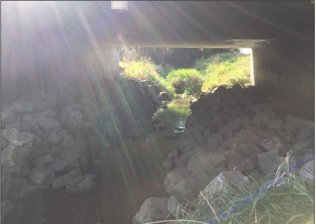
94. Looking south (upstream) of Wolf Creek and underneath Bridge No. 032-06-00583 D. Photo taken October 7, 2020.
