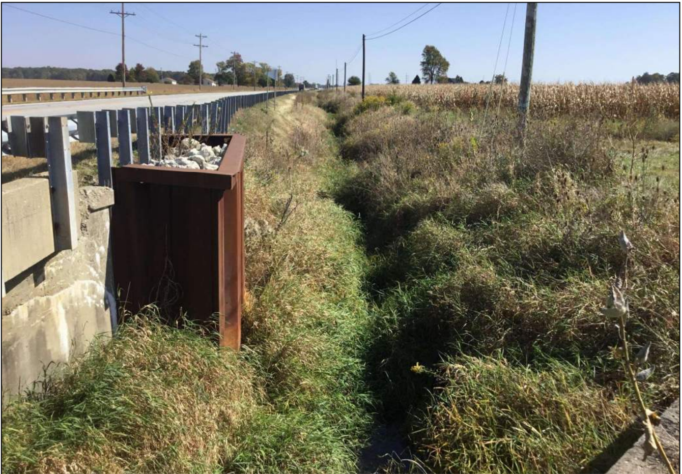
121. Looking east along the south side of SR 32 (upstream) Little Sugar Creek from the wingwall of CV 032-006-53.90. This structure will not be impacted as part of this project. Photo taken October 8, 2020.
