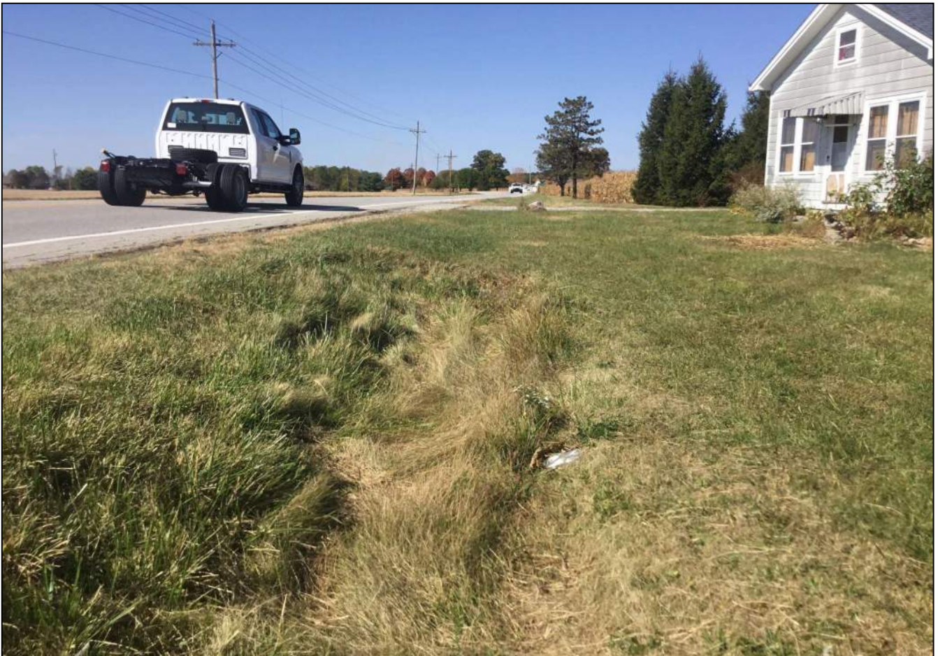
75. Looking northwest just west of the double barrel culvert pipe located on the north side of SR 32. Photo taken October 7, 2020.
