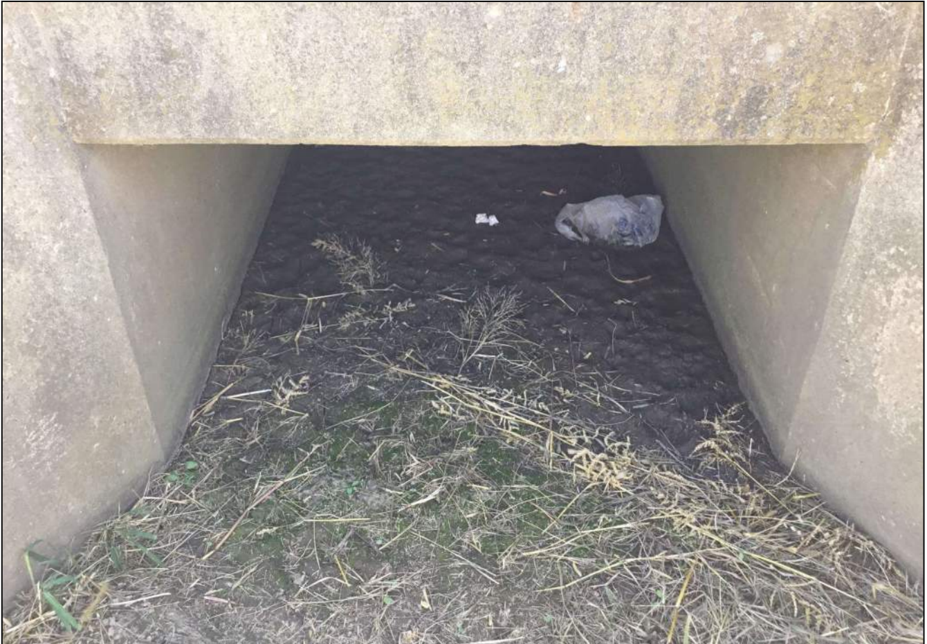
142. Looking south from the north side of SR 32 at Structure No. CV 032-006-53.38 (Structure No. 122) that conveys drainage underneath SR 32. Photo taken October 7, 2020.
