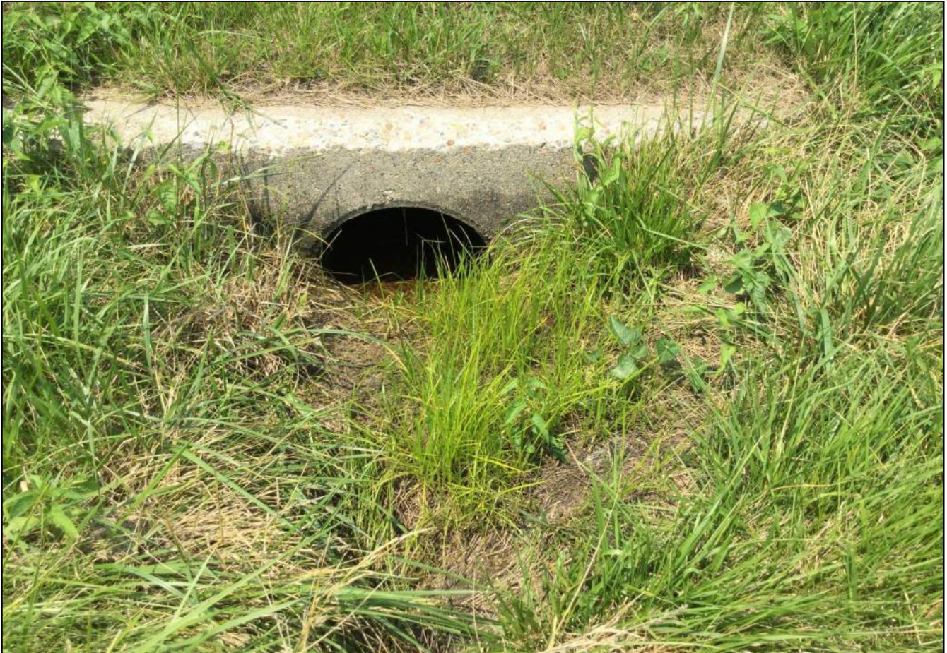
154. Looking north at Structure No. 120 located along the south side of SR 32. No stream or wetland feature was observed. This structure will be replaced as part of this project. Photo taken July 6, 2020.
