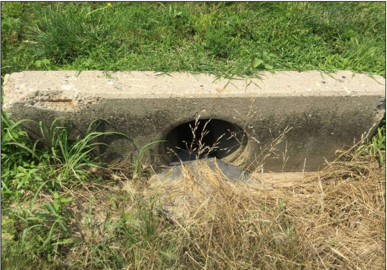
167. Looking north at Structure No. 112 located along the south side of SR 32. No stream or wetland features were observed. Photo taken July 6, 2021.
