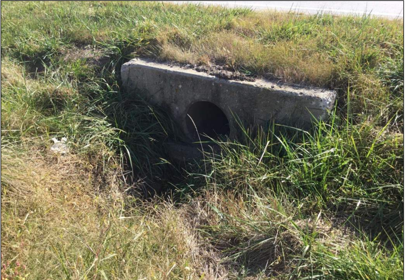
166. Looking southeast at Structure No. 112 located along the north side of SR 32. No stream or wetland features were observed. This structure will be replaced as part of this project. Photo taken October 7, 2020.
