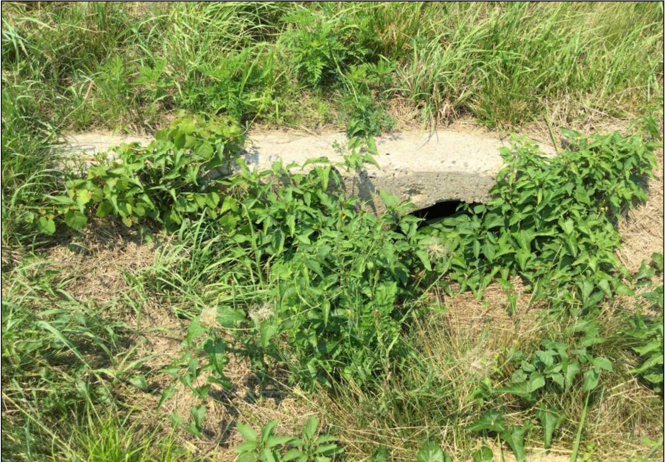
148. Looking north at Structure No. 121 located along the south side of SR 32. No stream or wetland features were observed. This structure will be replaced as part of this project. Photo taken July 6, 2021.
