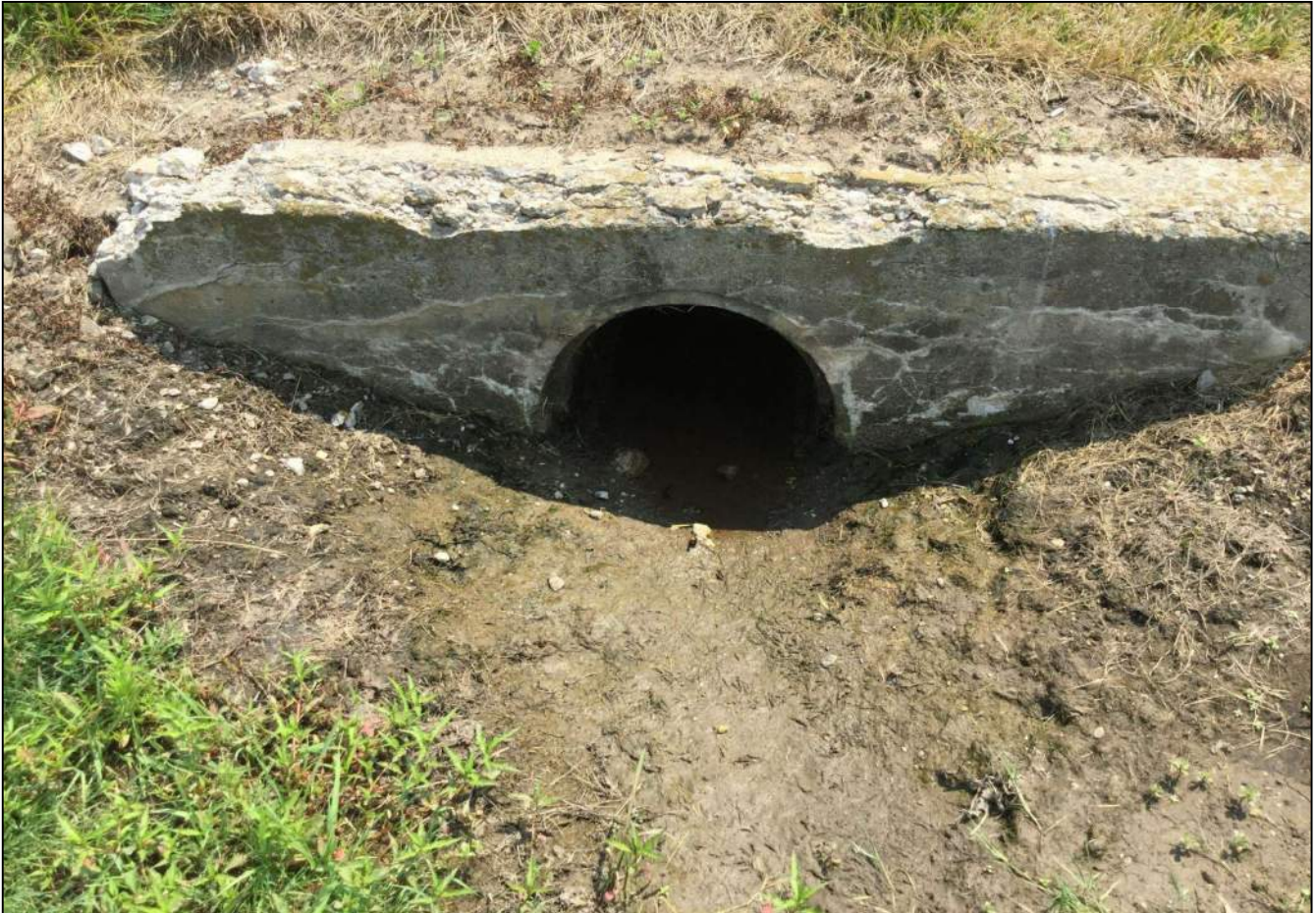
156. Looking south at Structure No. 120 located along the north side of SR 32 in front of the Western Boone High School. No stream or wetland features were observed. Photo taken July 6, 2021.
