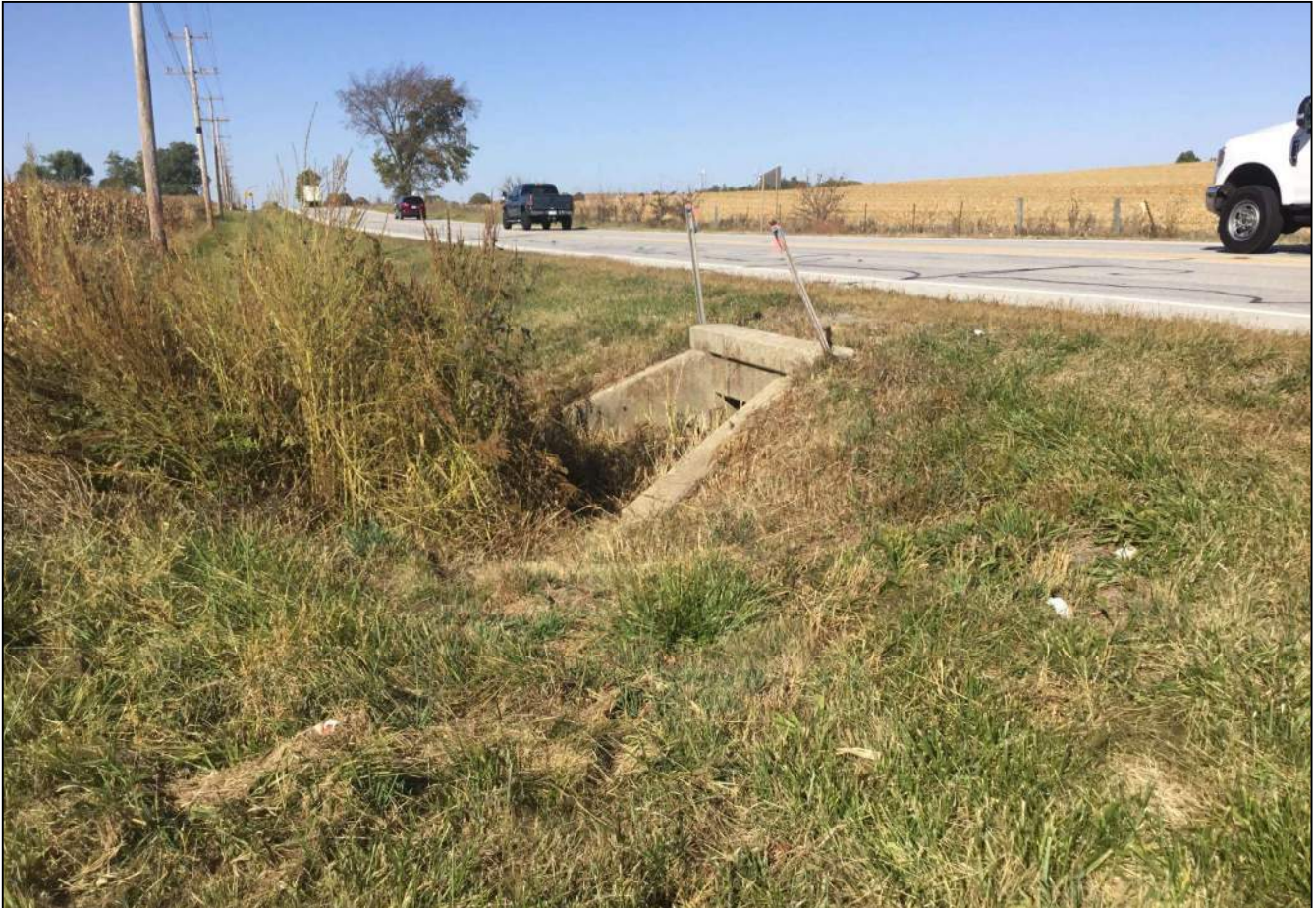
140. Looking northwest at a CV 032-006-53.38 (Structure No. 122) that conveys drainage underneath SR 32. This structure will be replaced as part of this project. No stream or wetlands were observed. Photo taken October 8, 2020.
