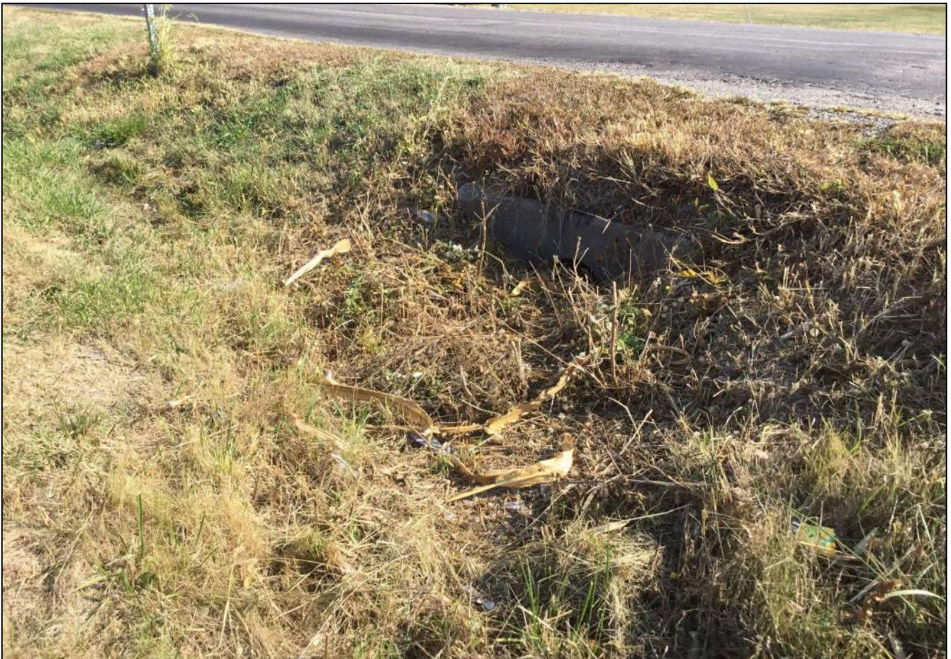
81. Looking northeast at a close up of the small diameter culvert pipe that conveys drainage underneath CR 500 W. on the west side of CR 500 W. Note that it is partially buried. Photo taken October 7, 2020.
