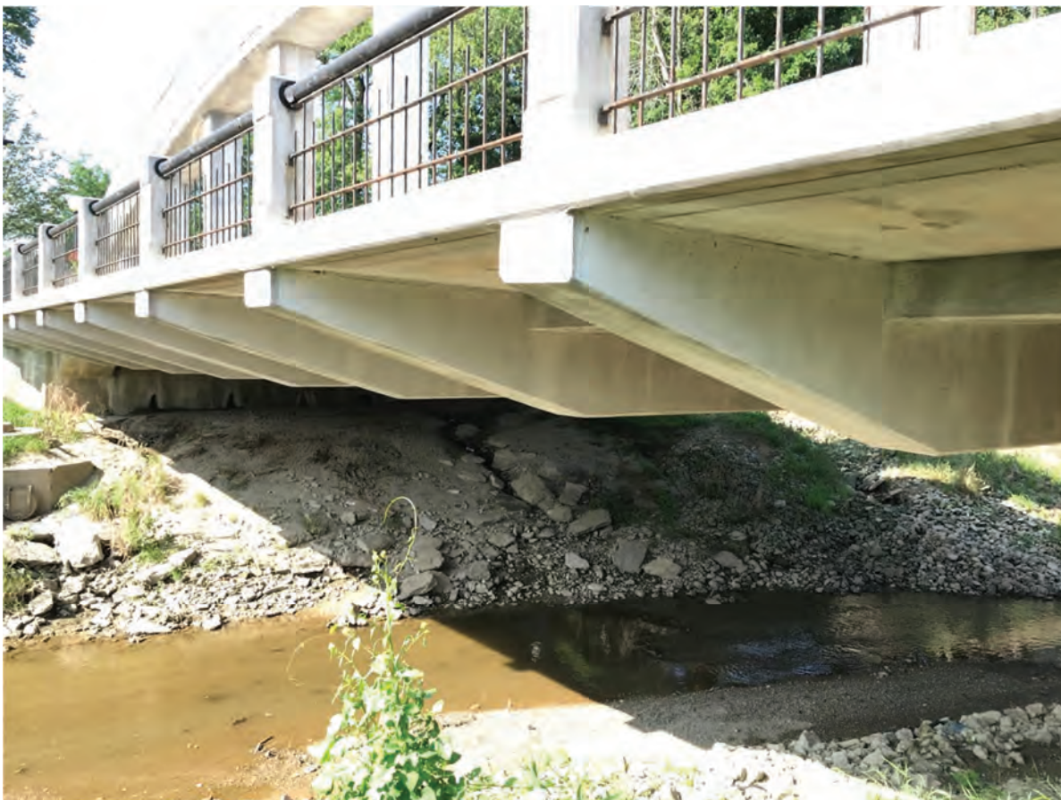
120. Looking SW in Portland Commercial Historic District (NR-1299) at IHSSI #075-521-33086, Meridian Street Bridge, Outstanding
