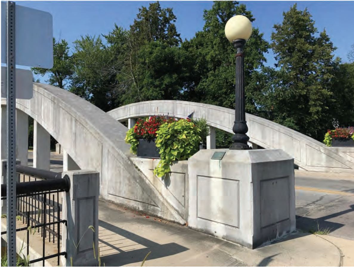
121. Looking SW in Portland Commercial Historic District (NR-1299) at lighting on IHSSI #075-521-33086, Meridian Street Bridge, Outstanding
