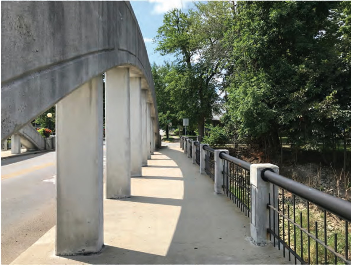
119. Looking S in Portland Commercial Historic District (NR-1299) on the S side of IHSSI #075-521-33086, Meridian Street Bridge, Outstanding
