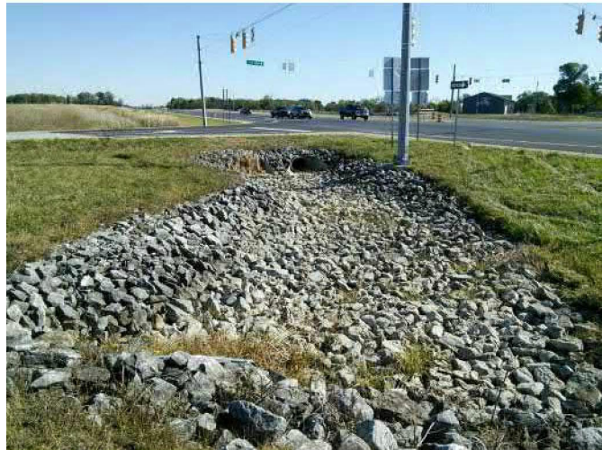
PP-7: Looking northeast at the riprap and culverts on the northwest side of the project area (2019-10-14)
