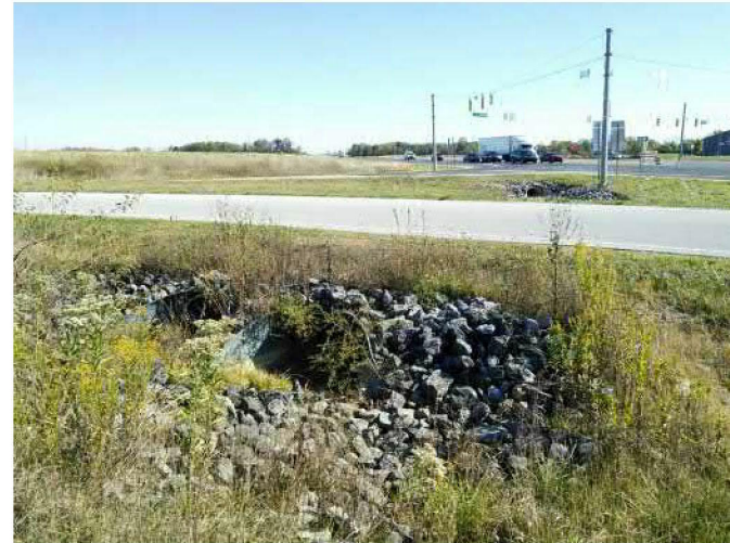
PP-6: Looking northeast at the culverts under the SR 46 junction to SR 3 on the northwest side of the project area (2019-10-14)
