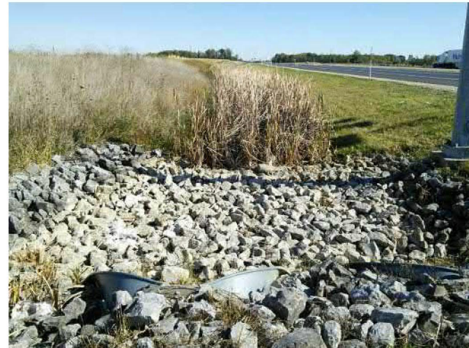
PP-8: Looking northeast at the culverts and riprap at the west side of the Wetland A (2019-10-14)
