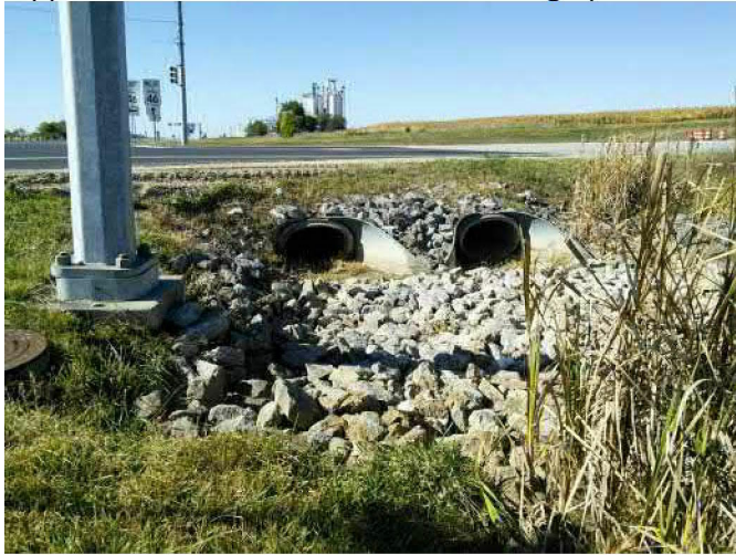
PP-8: Looking southwest at the culverts and riprap at the south end of Wetland A (2019-10-14)
