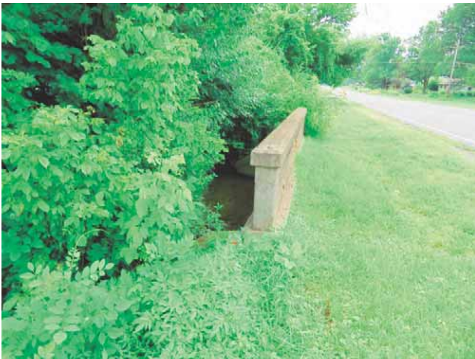
Photo 16: Investigation Area 2; looking south along the east side of US 31 towards the inlet of Camp Run
