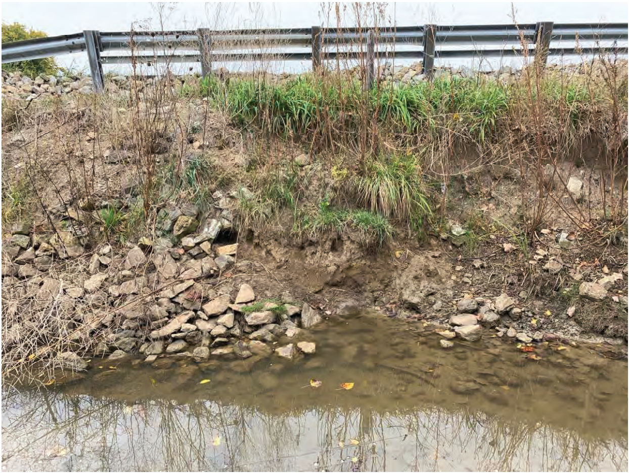
7. Looking north at slide to be corrected
