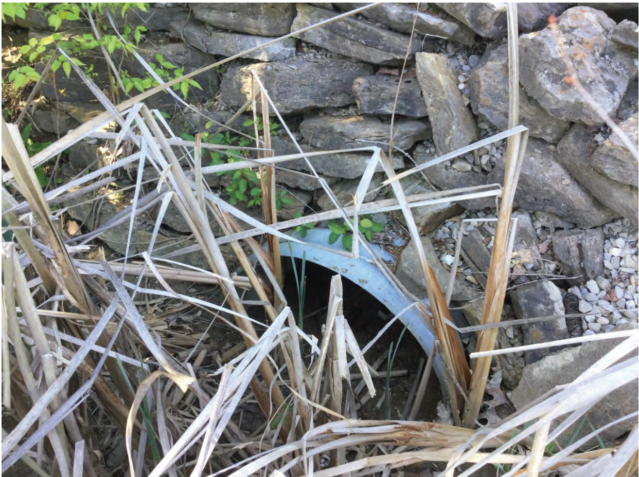
6. Looking west at culvert conveying drainage between Wetland A and Wetland B – 4/21/2020
