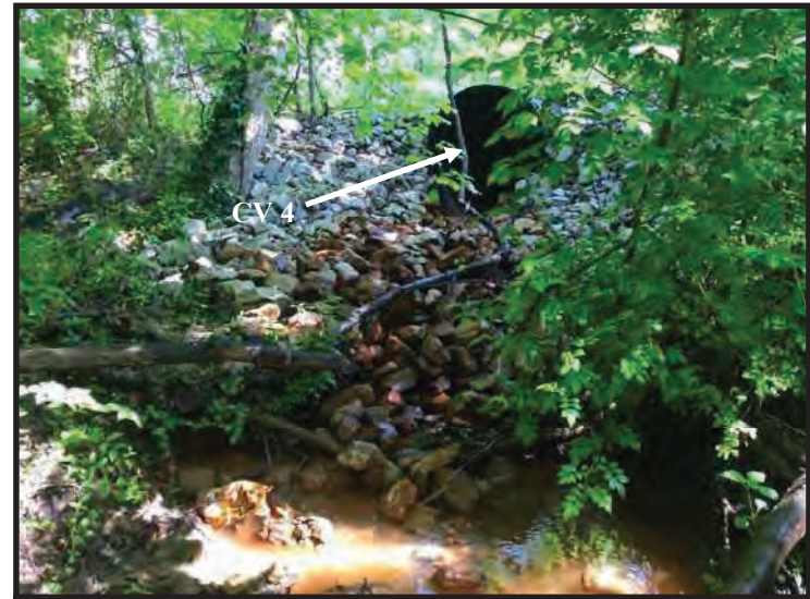
50. View of UNT 1 to Silver Creek and CV 4 at the northern PSL, looking north (upstream). (Taken 5/14/2020)
