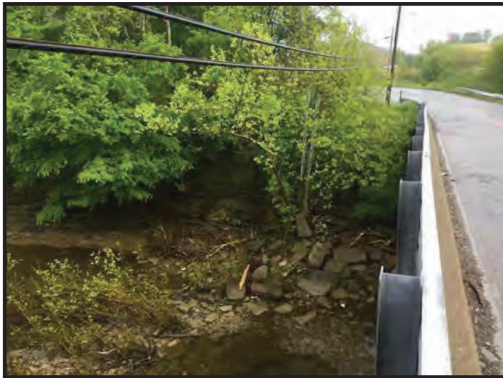
31. View of north bank of Silver Creek from Floyd County Bridge No. 51, looking northwest. (Taken 5/14/2020)
