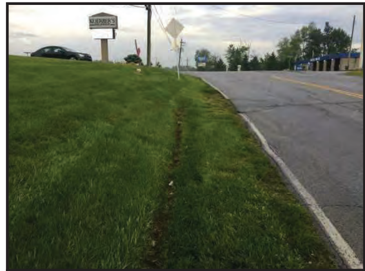
66. View of Blackiston Mill Rd ROW from CV 7 inlet, looking northwest. (Taken 5/14/2020)
