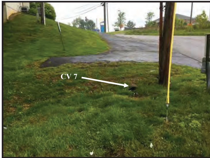
67. View of CV 7 outlet and Blackiston Mill Rd ROW, looking northwest. (Taken 5/14/2020)
