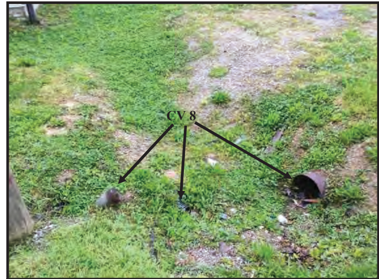
100. View of CV 8 (comprised of two metal pipes and one HDPE pipe), looking southwest. (Taken 5/14/2020)
