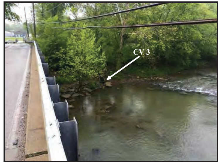
34. View of south bank of Silver Creek from Floyd County Bridge No. 51 and CV 3, looking southwest. (Taken 5/14/2020)
