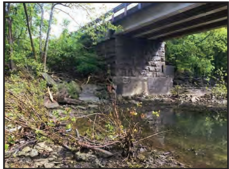
46. View of northern bank of Silver Creek from western PSL, looking northeast. (Taken 5/14/2020)
