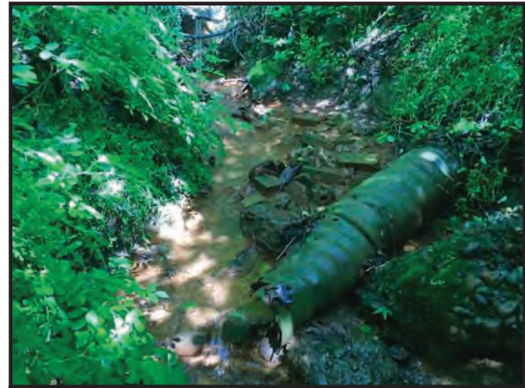
52. View of UNT 1 to Silver Creek and CV 5, looking northwest (upstream). (Taken 5/14/2020)
