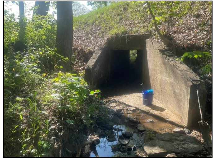
Photo 8. Inlet of culvert (CV 445-28-000.52) and UNT to Beech Creek north of SR 445 facing downstream, viewing southeast, 5/13/2022
