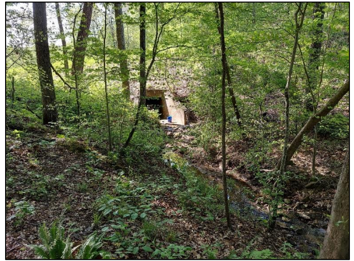
Photo 10. Inlet of culvert (CV 445-28-000.52) and UNT to Beech Creek with surrounding forest facing downstream, viewing southeast, 5/13/2022
