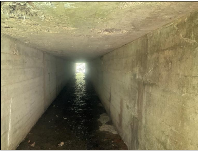
Photo 9. Inside of culvert (CV 445-28-000.52) at inlet and UNT to Beech Creek facing downstream, viewing southeast, 5/13/2022
