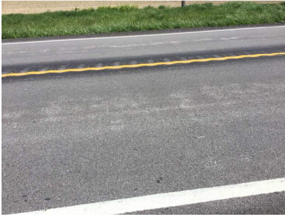
PHOTO 3 Condition Description Pavement condition above culvert
