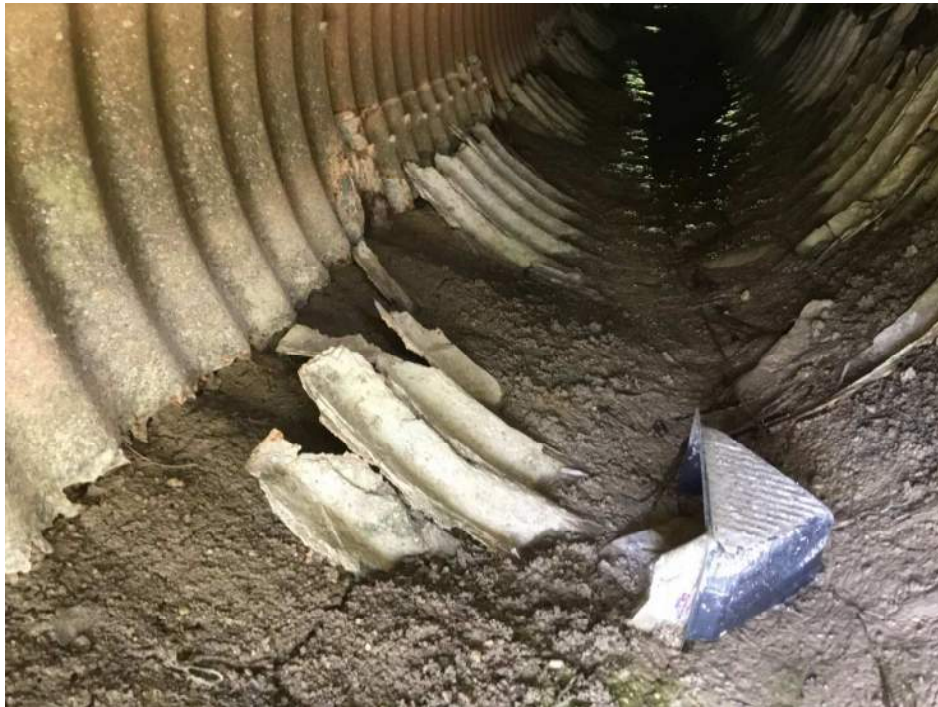
PHOTO 6 Condition Description Looking South through middle pipe showing no bottom
