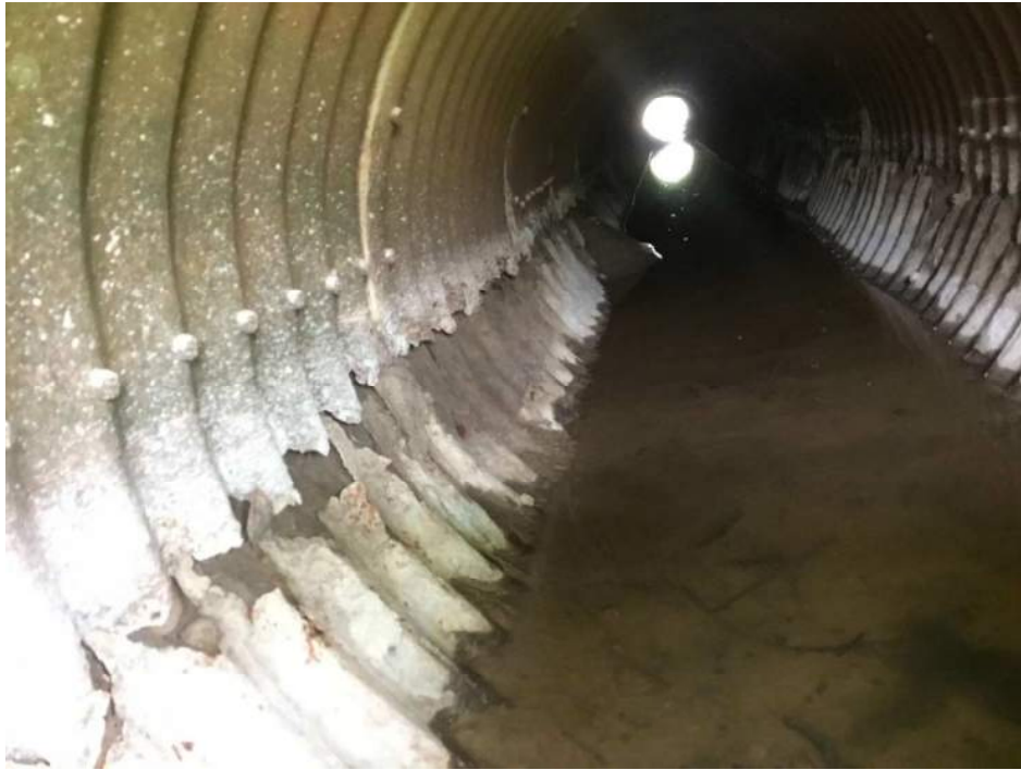
PHOTO 9 Condition Description Looking North through middle pipe showing rusted through areas
