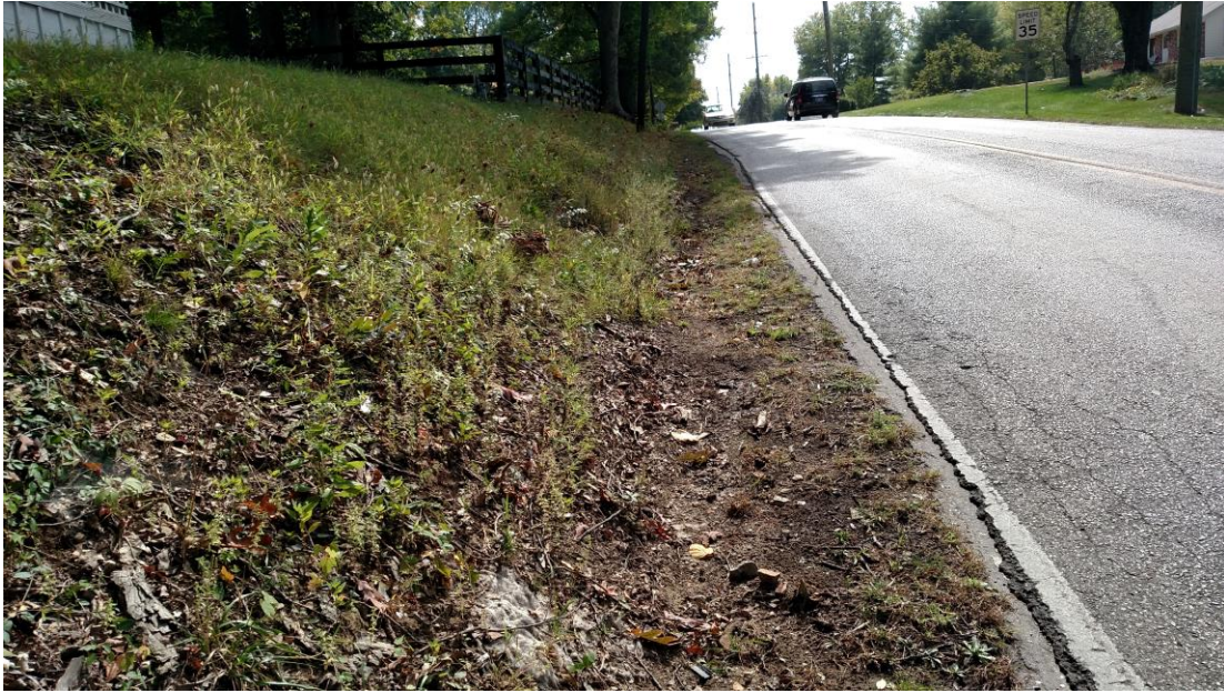
Shallow roadside ditch
