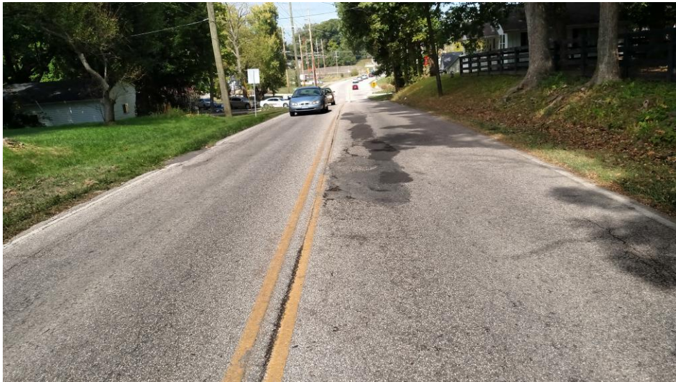
Pavement condition and worn markings
