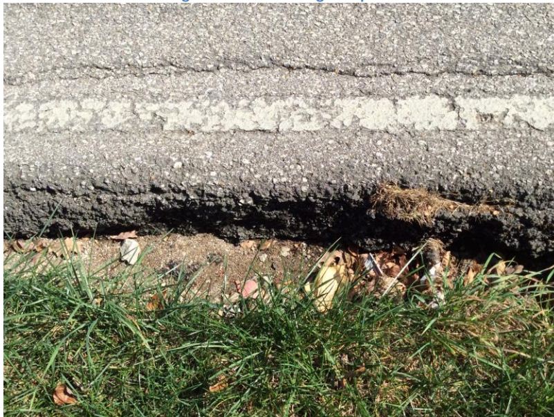
Figure 1: Shoulder edge drop-off
