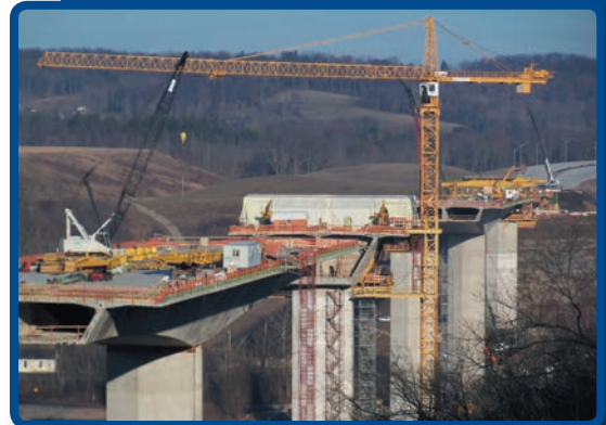
Example from Pennsylvania of the tower cranes to be used on this project.
