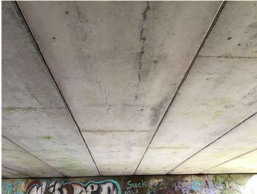
PHOTO 15 Description Beams 4, 5 and 6 longitudinal cracking looking east
