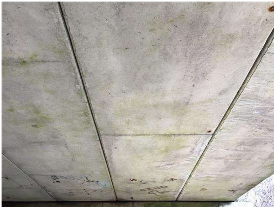
PHOTO 16 Description Beams 7 and 9 longitudinal cracking looking east
