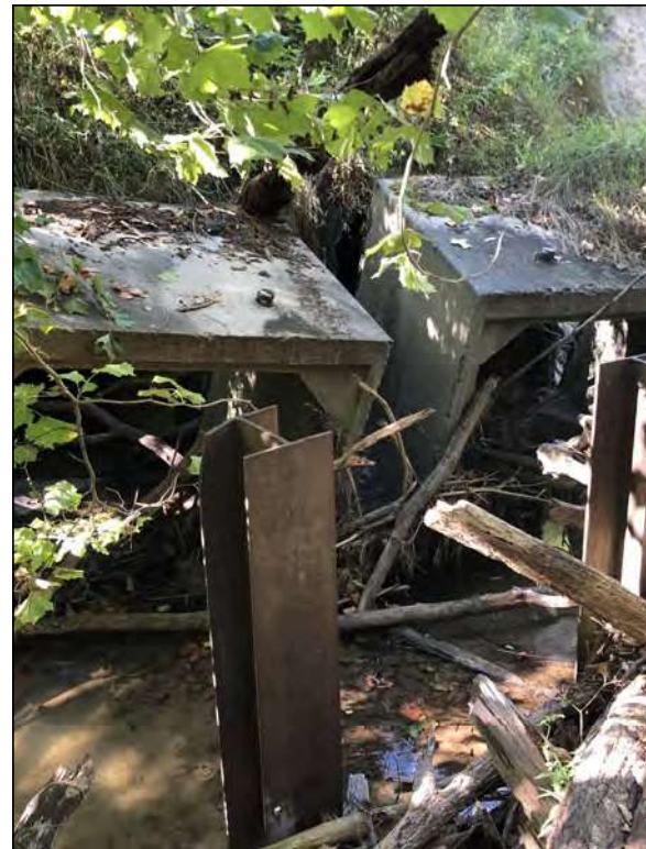
Picture 12—Goose Creek structure CV 026-079-28.10 inlet; southwest view; 1 SEP 2021. Note that culvert end pieces have detached.
