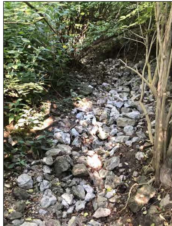
Picture 36—UNT 3 to Goose Creek end of bed and bank structure—note riprap; west view; 1 SEP 2021.
