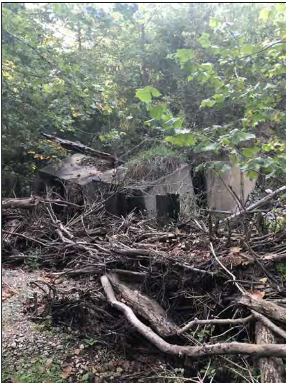
Picture 11—Goose Creek debris north of structure CV 026-079-28.10 inlet; southeast view; 14 SEP 2021. Note that steel beams have collected debris.
