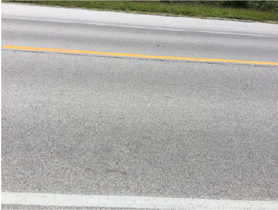
PHOTO 3 Condition Description Pavement condition above culvert
