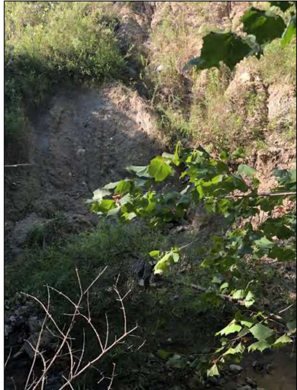
Picture 50—Eroded area west of the Goose Creek structure CV 026-079-28.10 inlet. Erosion is extensive upslope to SR 26; southwest view; 1 SEP 2021.
