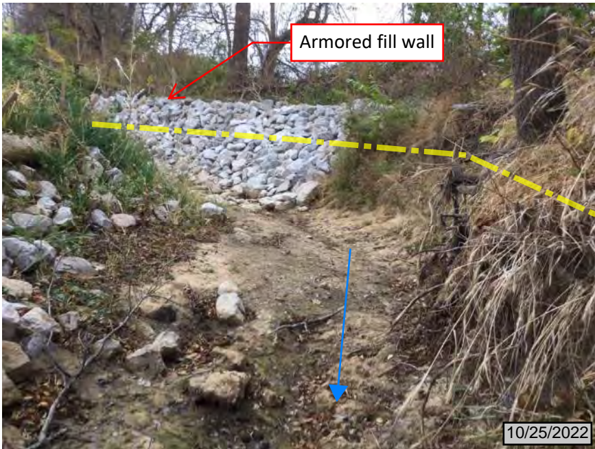
9. Looking west, upstream along Lost Creek, at riprap on north side of SR 64
