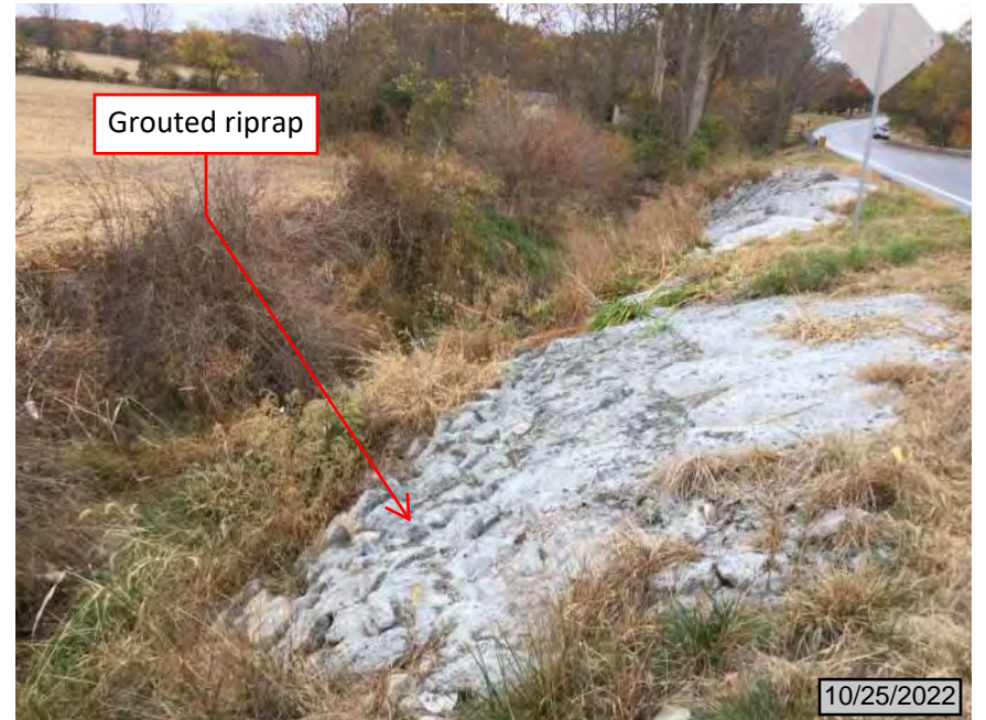
28. Looking east at roadside slope and UNT 1 to Lost Creek on north side of SR 64
