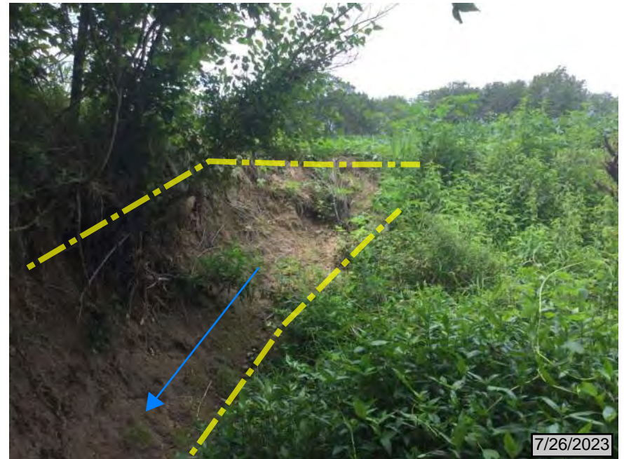
42. North of SR 64, looking north, upstream, to eroded bank of UNT 2 to Lost Creek
