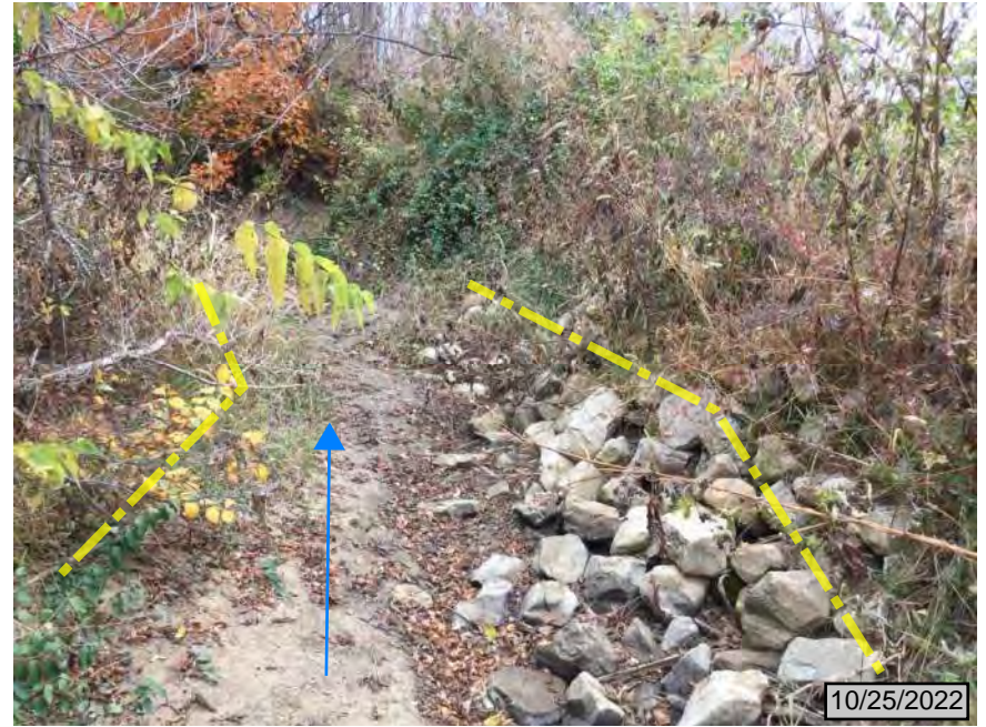
18. Looking east, downstream, toward bend of Lost Creek on north side of SR 64
