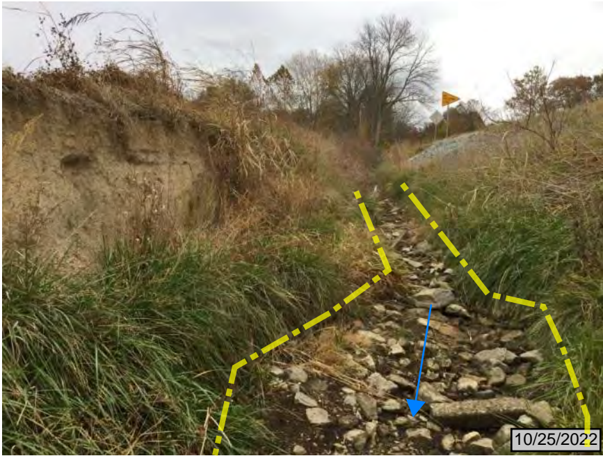
25. On the north side of SR 64, looking southeast, upstream, at UNT 1 to Lost Creek
