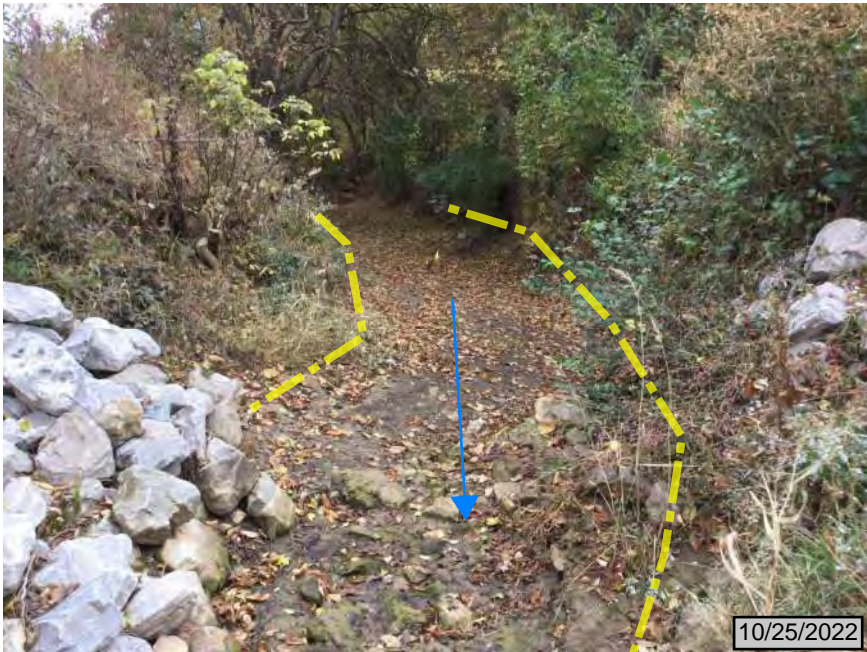
3. Facing south side of SR 64 from structure, looking upstream along Lost Creek Des No. 2100263
