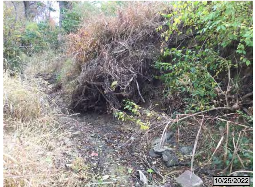
14. North of SR 64, facing southeast toward scoured roadside slope
