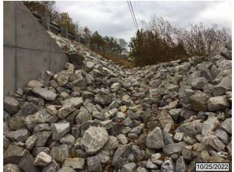
4. On south side of SR 64 facing northeast toward riprap armor at headwall
