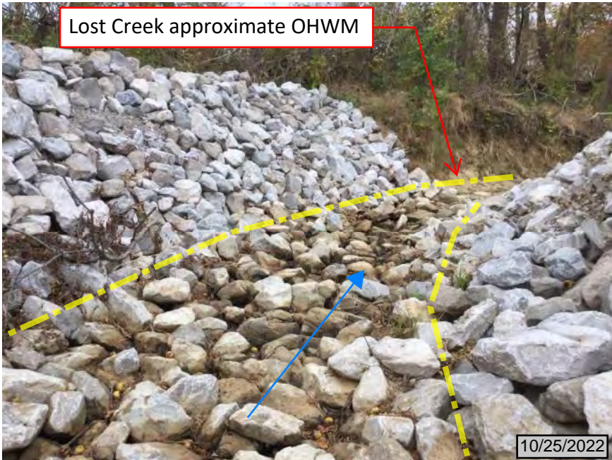
7. Facing northeast, looking downstream along Lost Creek, toward riprap at structure outlet on north side of SR 64 Des No. 2100263
