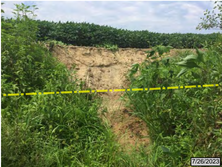
43. North of SR 64, looking west to eroded bank of UNT 2 to Lost Creek Des No. 2100263
