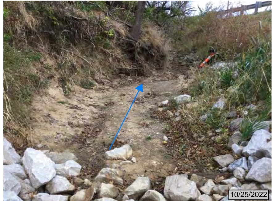
8. Facing southeast, downstream, at end of riprap on north side of SR 64
