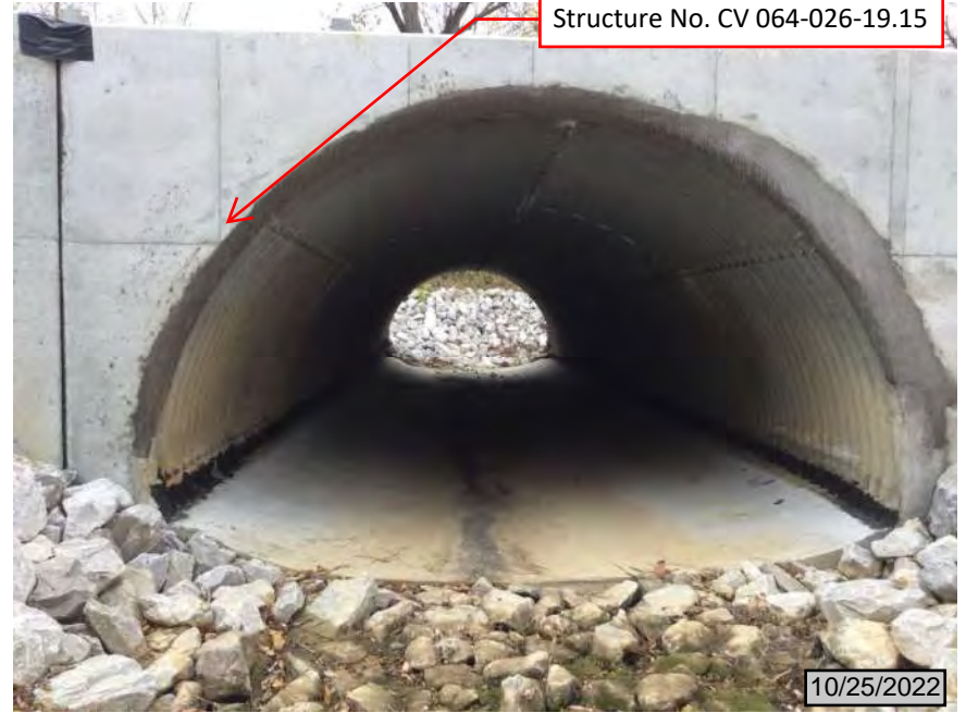
6. Facing northeast toward culvert on south side of SR 64, looking downstream along Lost Creek through culvert
