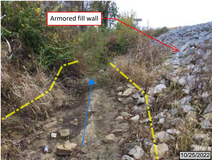
11. Facing southwest on the north side of SR 64, looking downstream at roadside slope and Lost Creek Des No. 2100263
