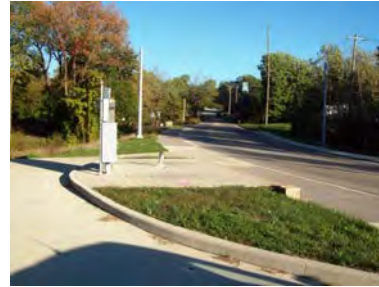
Figure 4.2-26: CBU Lift Station on Vernal Pike
