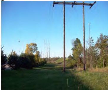
Figure 4.2-25: Duke Energy Transmission Line
