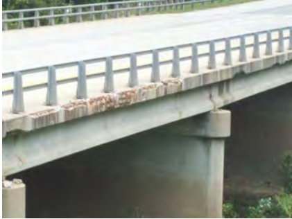
Figure 4.2-18: Spalling of Concrete on Bridge Deck
