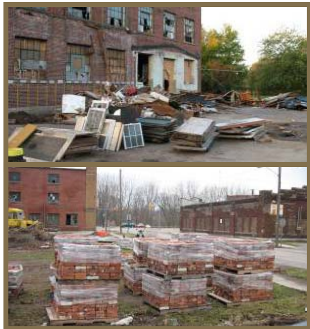
Building materials from the former Essex Wire site in Ligonier in the process of being recycled.
