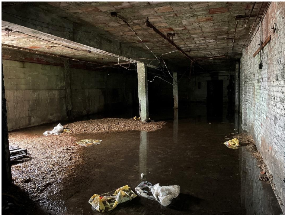
DATE: May 16, 2024 LOCATION: Former Dodge Manufacturing Company / Former RMG Foundry SUBJECT: View of room in northern portion of the complex
