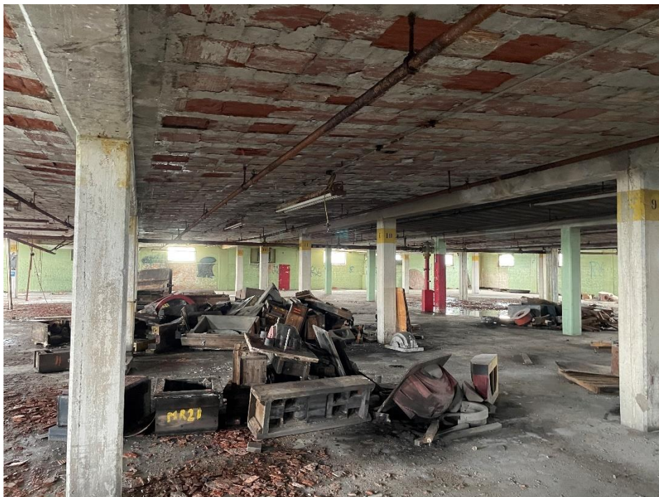
DATE: May 16, 2024 LOCATION: Former Dodge Manufacturing Company / Former RMG Foundry SUBJECT: View of machinery parts in southeastern portion of the complex PHOTOGRAPHER: Robert R. Raduchel (Heartland) PHOTO: 35
