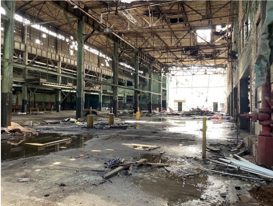
DATE: May 16, 2024 LOCATION: Former Dodge Manufacturing Company / Former RMG Foundry SUBJECT: View of the western portion of the foundry PHOTOGRAPHER: Robert R. Raduchel (Heartland) PHOTO: 15
