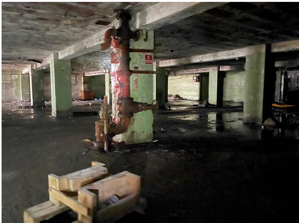
DATE: May 16, 2024 LOCATION: Former Dodge Manufacturing Company / Former RMG Foundry SUBJECT: View of the fire suppression system in southeastern basement PHOTOGRAPHER: Robert R. Raduchel (Heartland) PHOTO: 29
