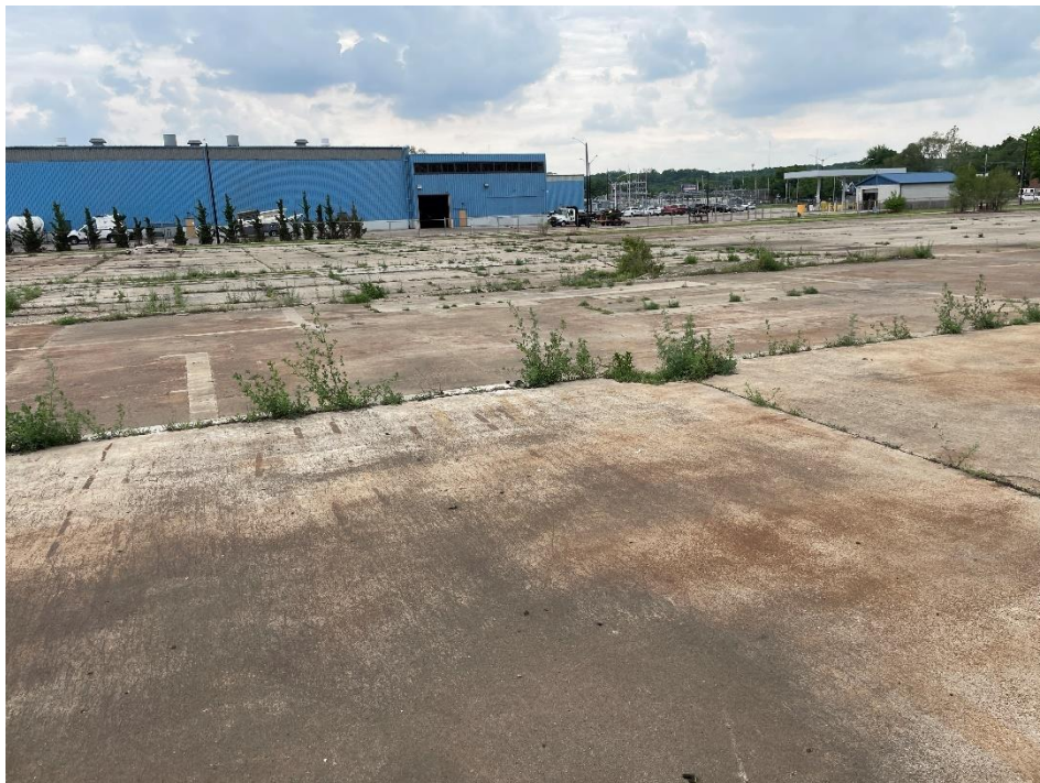
DATE: May 16, 2024 LOCATION: Former Dodge Manufacturing Company / Former RMG Foundry SUBJECT: Additional view of the foundation of the burned southeastern portion of the complex, looking south-southeast PHOTOGRAPHER: Robert R. Raduchel (Heartland) PHOTO: 75
