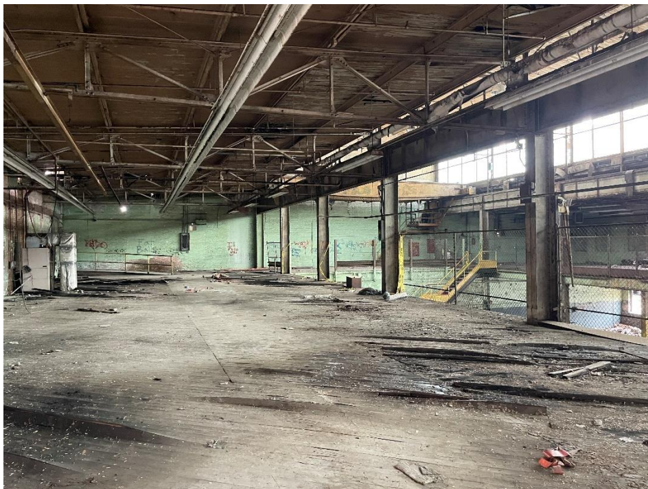
DATE: May 16, 2024 LOCATION: Former Dodge Manufacturing Company / Former RMG Foundry SUBJECT: additional view of the second floor of the western portion of the complex PHOTOGRAPHER: Robert R. Raduchel (Heartland) PHOTO: 31
