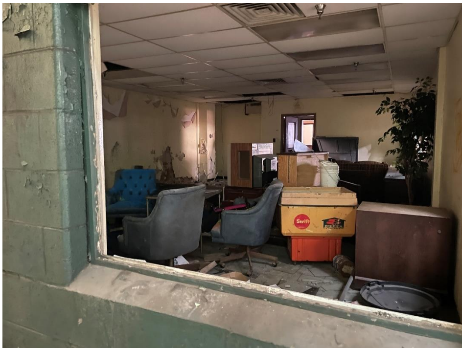
DATE: May 16, 2024 LOCATION: Former Dodge Manufacturing Company / Former RMG Foundry SUBJECT: View of the office in southern portion of the complex PHOTOGRAPHER: Robert R. Raduchel (Heartland) PHOTO: 19
