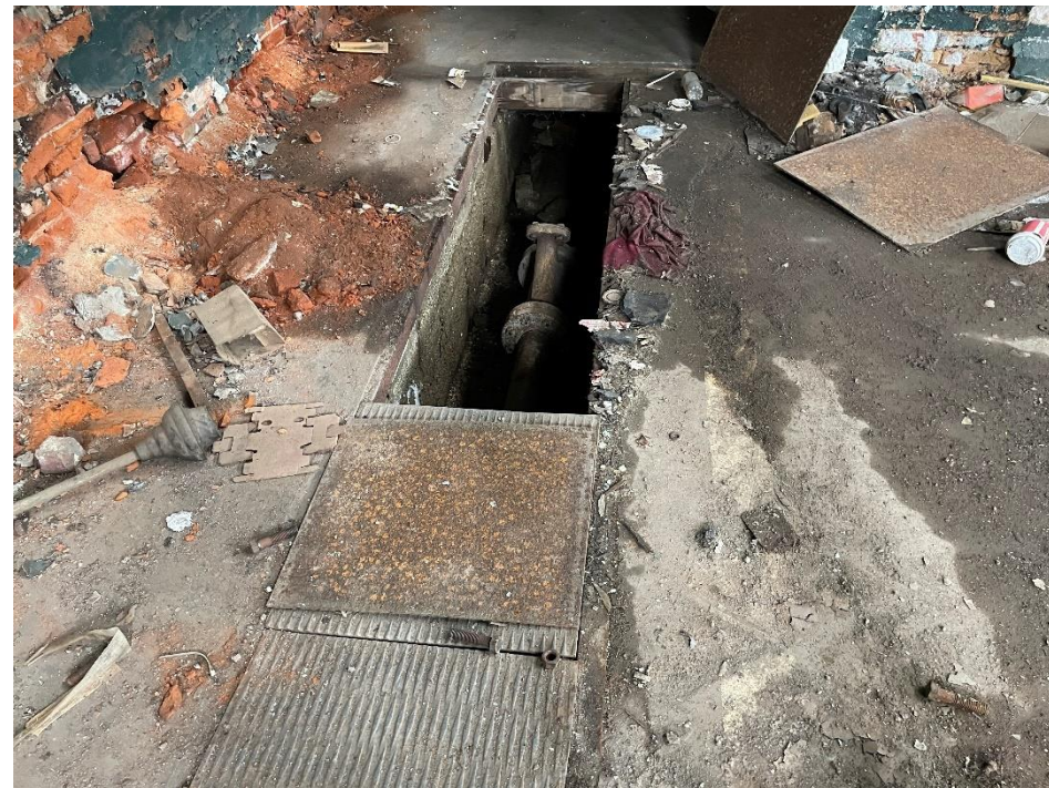
DATE: May 16, 2024 LOCATION: Former Dodge Manufacturing Company / Former RMG Foundry SUBJECT: View of pipe chase in floor of the power house PHOTOGRAPHER: Robert R. Raduchel (Heartland) PHOTO: 84
