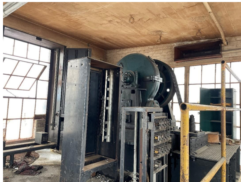
DATE: May 16, 2024 LOCATION: Former Dodge Manufacturing Company / Former RMG Foundry SUBJECT: View of additional hoist in southeastern portion of the complex PHOTOGRAPHER: Robert R. Raduchel (Heartland) PHOTO: 38
