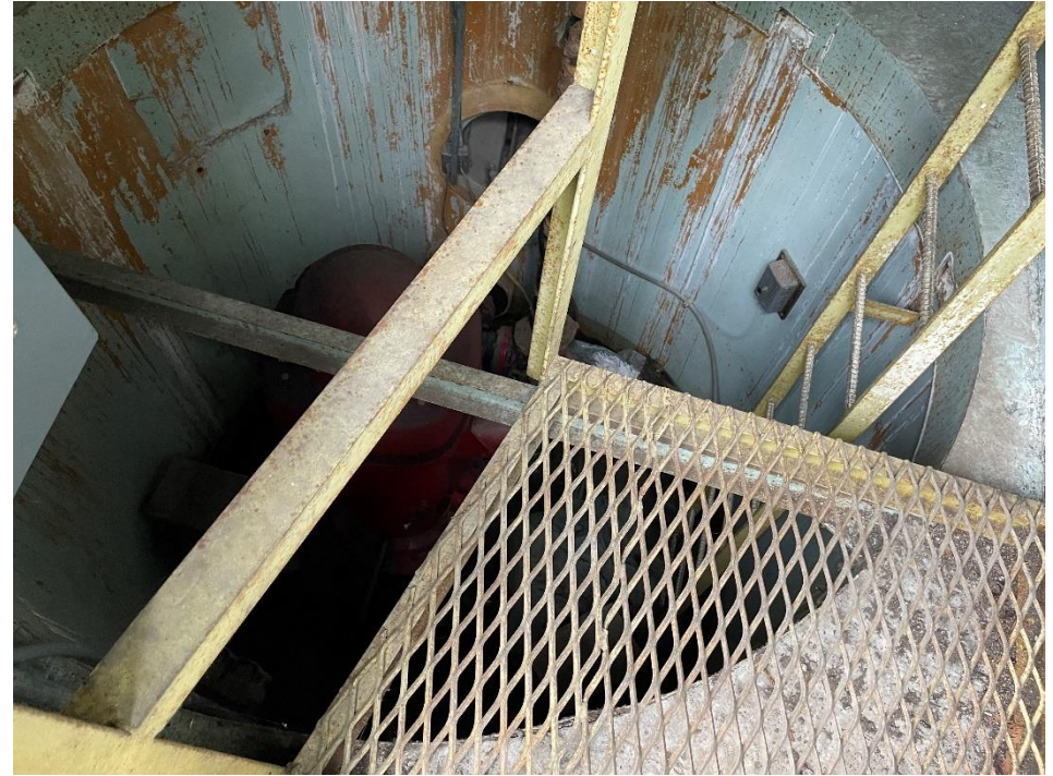
DATE: May 16, 2024 LOCATION: Former Dodge Manufacturing Company / Former RMG Foundry SUBJECT: View of the fire suppression building interior PHOTOGRAPHER: Robert R. Raduchel (Heartland) PHOTO: 78
