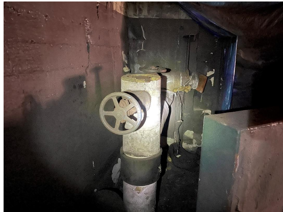
DATE: May 16, 2024 LOCATION: Former Dodge Manufacturing Company / Former RMG Foundry SUBJECT: View of the secondary water main on eastern portion of the complex
