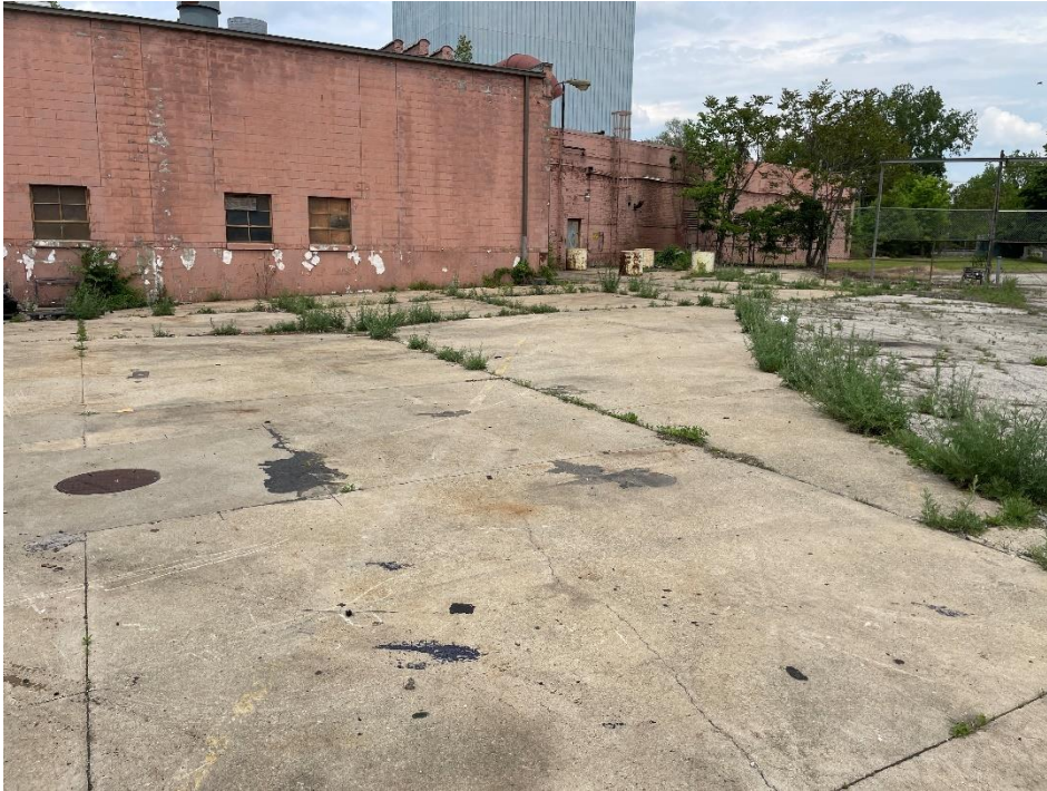
DATE: May 16, 2024 LOCATION: Former Dodge Manufacturing Company / Former RMG Foundry SUBJECT: View of the eastern portion of the complex, looking northeast PHOTOGRAPHER: Robert R. Raduchel (Heartland) PHOTO: 63
