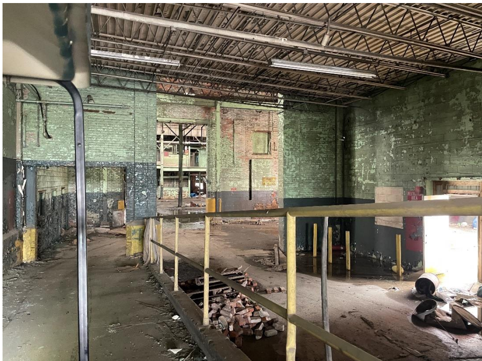
DATE: May 16, 2024 LOCATION: Former Dodge Manufacturing Company / Former RMG Foundry SUBJECT: View of the southeastern portion of the complex PHOTOGRAPHER: Robert R. Raduchel (Heartland) PHOTO: 43
