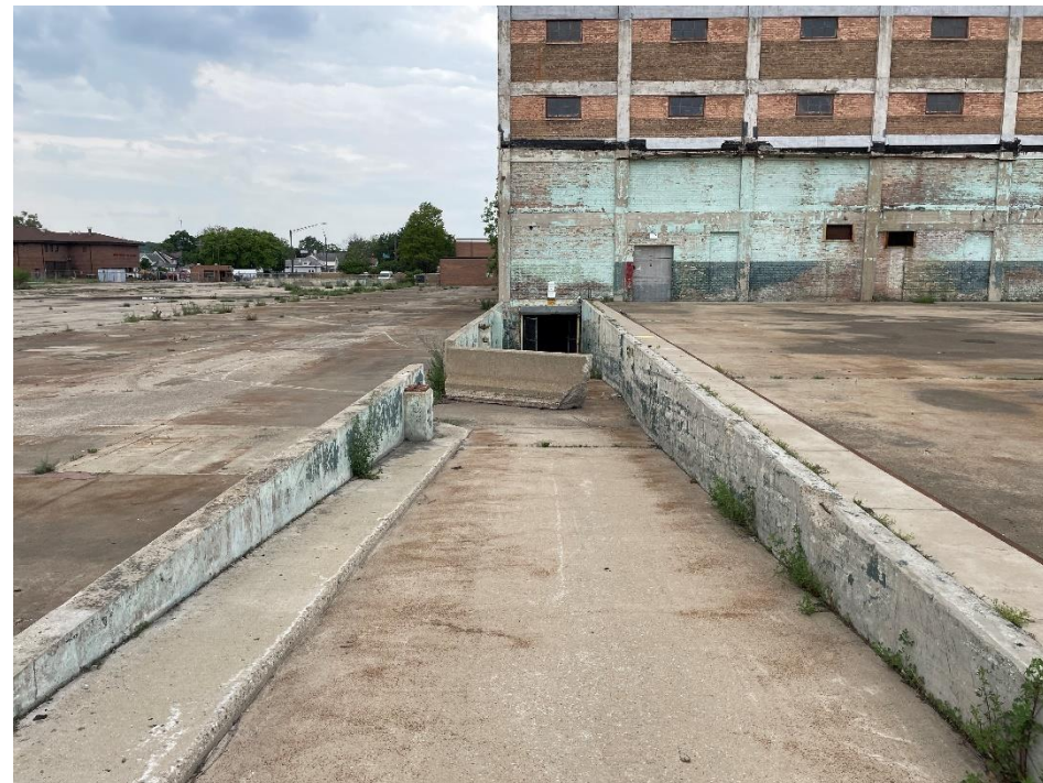
DATE: May 16, 2024 LOCATION: Former Dodge Manufacturing Company / Former RMG Foundry SUBJECT: View of the southeast basement entrance PHOTOGRAPHER: Robert R. Raduchel (Heartland) PHOTO: 76
