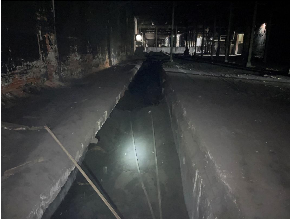
DATE: May 16, 2024 LOCATION: Former Dodge Manufacturing Company / Former RMG Foundry SUBJECT: View of sand conveyor in northern portion of the complex PHOTOGRAPHER: Robert R. Raduchel (Heartland) PHOTO: 53
