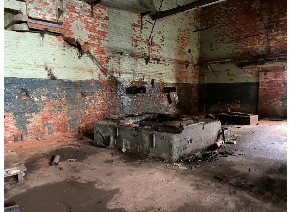
DATE: May 16, 2024 LOCATION: Former Dodge Manufacturing Company / Former RMG Foundry SUBJECT: View of additional compressor pads PHOTOGRAPHER: Robert R. Raduchel (Heartland) PHOTO: 86
