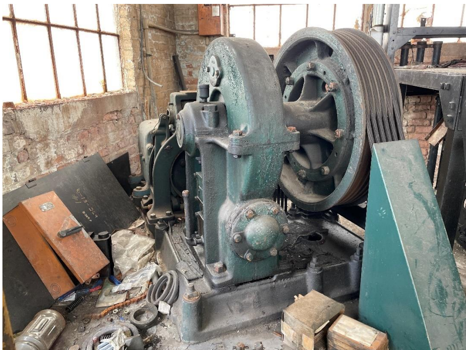
DATE: May 16, 2024 LOCATION: Former Dodge Manufacturing Company / Former RMG Foundry SUBJECT: View of hoist in southeastern portion of the complex PHOTOGRAPHER: Robert R. Raduchel (Heartland) PHOTO: 37
