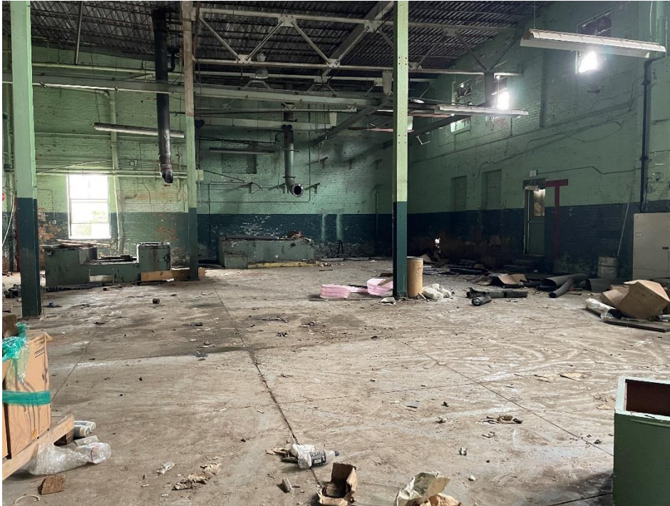
DATE: May 16, 2024 LOCATION: Former Dodge Manufacturing Company / Former RMG Foundry SUBJECT: View of the powerhouse room and compressor pads PHOTOGRAPHER: Robert R. Raduchel (Heartland) PHOTO: 85
