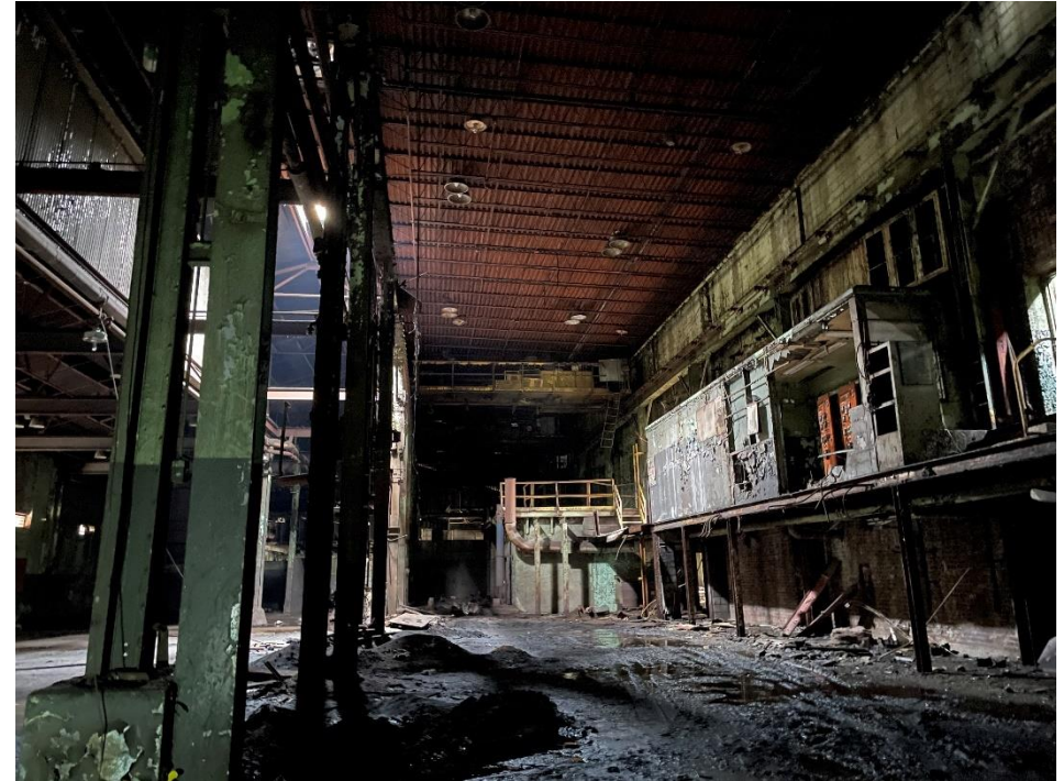
DATE: May 16, 2024 LOCATION: Former Dodge Manufacturing Company / Former RMG Foundry SUBJECT: View of former furnace area in northern portion of the complex PHOTOGRAPHER: Robert R. Raduchel (Heartland) PHOTO: 54
