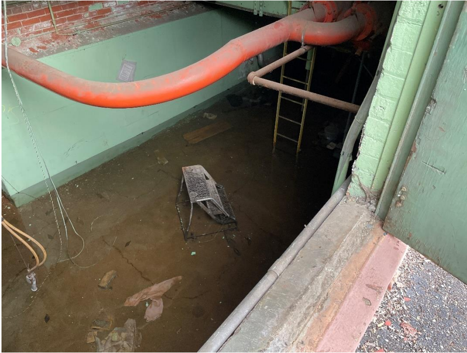
DATE: May 16, 2024 LOCATION: Former Dodge Manufacturing Company / Former RMG Foundry SUBJECT: View of the flooded powerhouse basement PHOTOGRAPHER: Robert R. Raduchel (Heartland) PHOTO: 77
