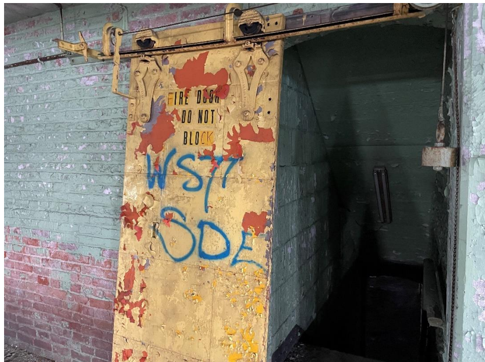
DATE: May 16, 2024 LOCATION: Former Dodge Manufacturing Company / Former RMG Foundry SUBJECT: View of fire door in southeastern portion of the complex
