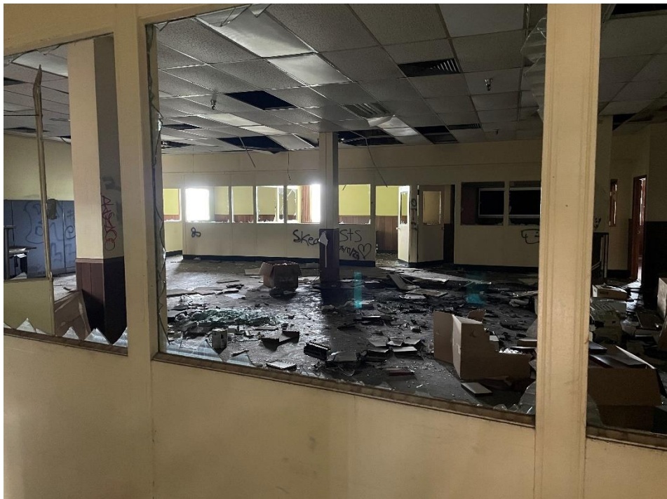
DATE: May 16, 2024 LOCATION: Former Dodge Manufacturing Company / Former RMG Foundry SUBJECT: View of the second floor offices in northwestern corner of the complex PHOTOGRAPHER: Robert R. Raduchel (Heartland) PHOTO: 45
