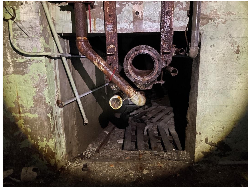
DATE: May 16, 2024 LOCATION: Former Dodge Manufacturing Company / Former RMG Foundry SUBJECT: View of steam and air pipes leading to the western power house PHOTOGRAPHER: Robert R. Raduchel (Heartland) PHOTO: 28
