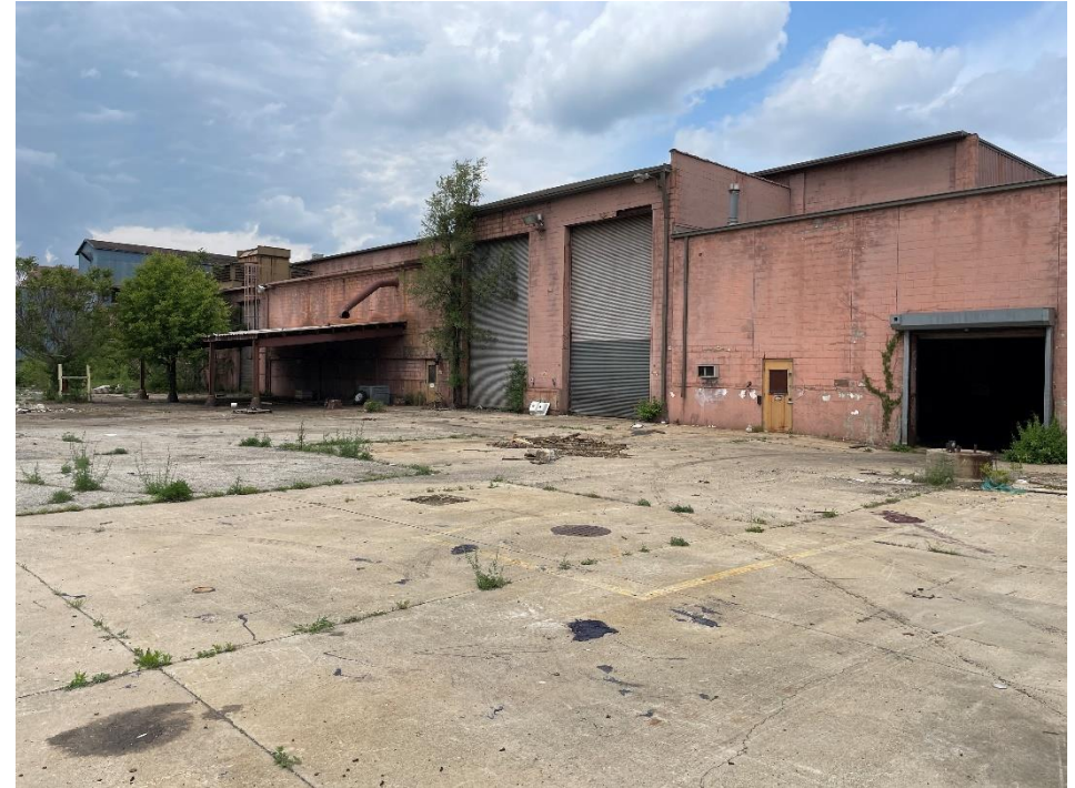
DATE: May 16, 2024 LOCATION: Former Dodge Manufacturing Company / Former RMG Foundry SUBJECT: View of the lean-to against eastern portion of the complex PHOTOGRAPHER: Robert R. Raduchel (Heartland) PHOTO: 64
