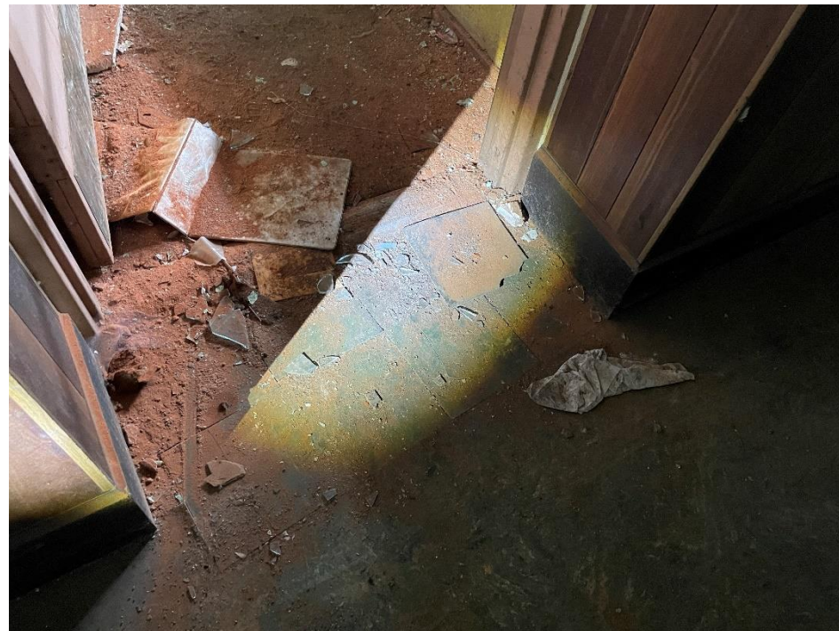
DATE: May 16, 2024 LOCATION: Former Dodge Manufacturing Company / Former RMG Foundry SUBJECT: View of the linoleum tile in second floor office area PHOTOGRAPHER: Robert R. Raduchel (Heartland) PHOTO: 46
