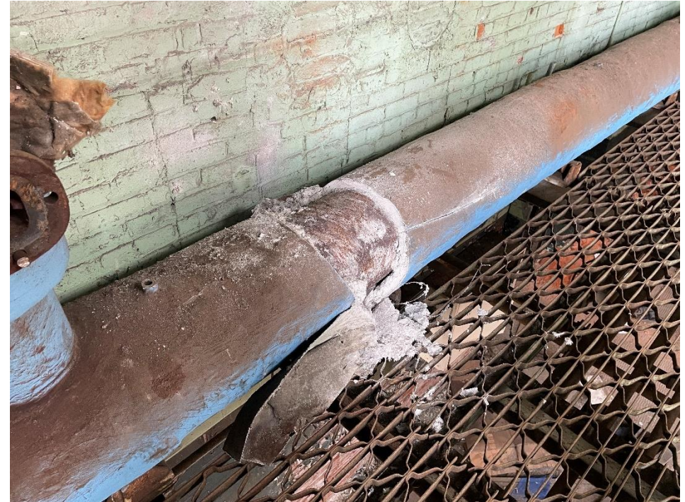
DATE: May 16, 2024 LOCATION: Former Dodge Manufacturing Company / Former RMG Foundry SUBJECT: View of insulated pipe in power house PHOTOGRAPHER: Robert R. Raduchel (Heartland) PHOTO: 88
