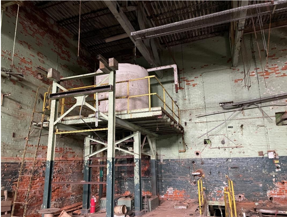
DATE: May 16, 2024 LOCATION: Former Dodge Manufacturing Company / Former RMG Foundry SUBJECT: View of water softening tank in power house PHOTOGRAPHER: Robert R. Raduchel (Heartland) PHOTO: 87
