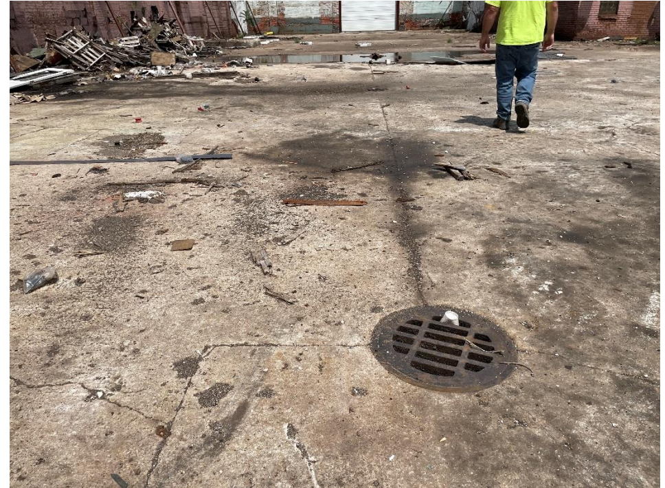
DATE: May 16, 2024 LOCATION: Former Dodge Manufacturing Company / Former RMG Foundry SUBJECT: View of staining around drain PHOTOGRAPHER: Robert R. Raduchel (Heartland) PHOTO: 10
