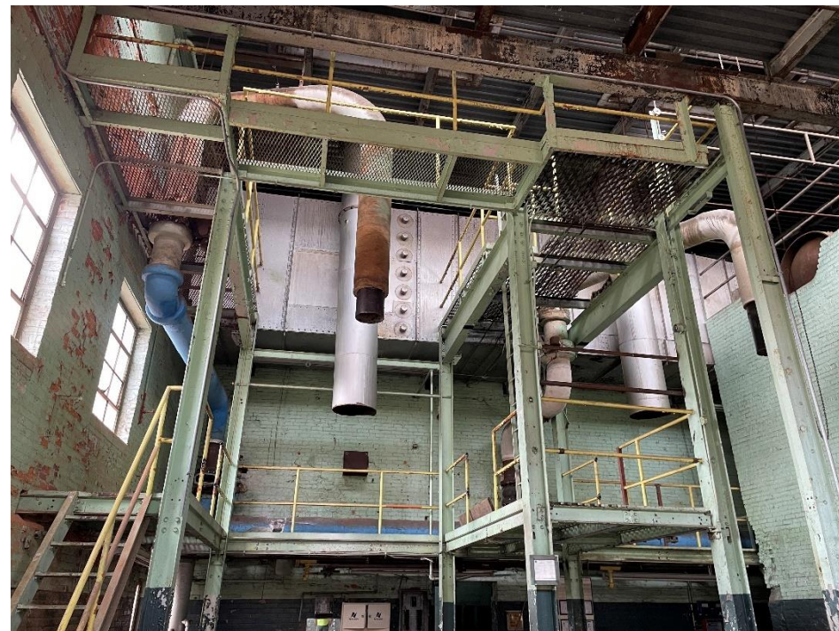
DATE: May 16, 2024 LOCATION: Former Dodge Manufacturing Company / Former RMG Foundry SUBJECT: View of the boiler vents and water lines in power house PHOTOGRAPHER: Robert R. Raduchel (Heartland) PHOTO: 82
