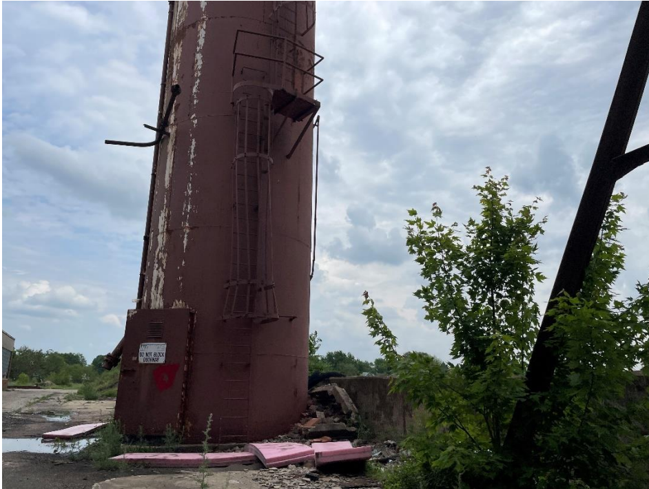
DATE: May 16, 2024 LOCATION: Former Dodge Manufacturing Company / Former RMG Foundry SUBJECT: View of the base of the foundry sand silo (AST)
