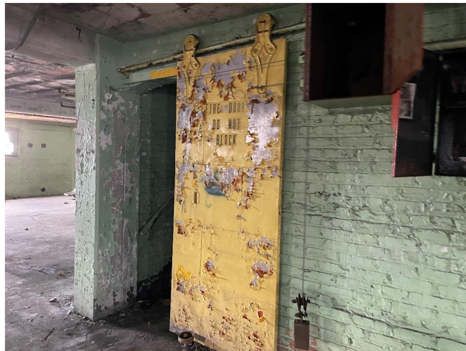
DATE: May 16, 2024 LOCATION: Former Dodge Manufacturing Company / Former RMG Foundry SUBJECT: View of additional fire door in southeastern portion of the complex
