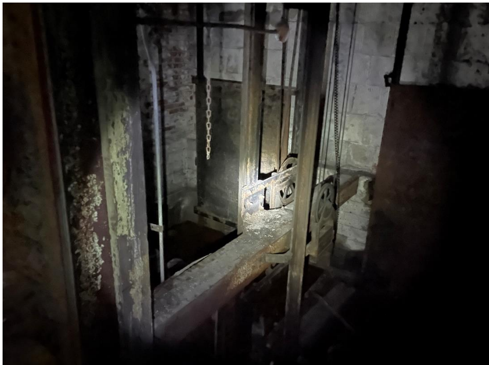
DATE: May 16, 2024 LOCATION: Former Dodge Manufacturing Company / Former RMG Foundry SUBJECT: View of the freight elevator pulleys
