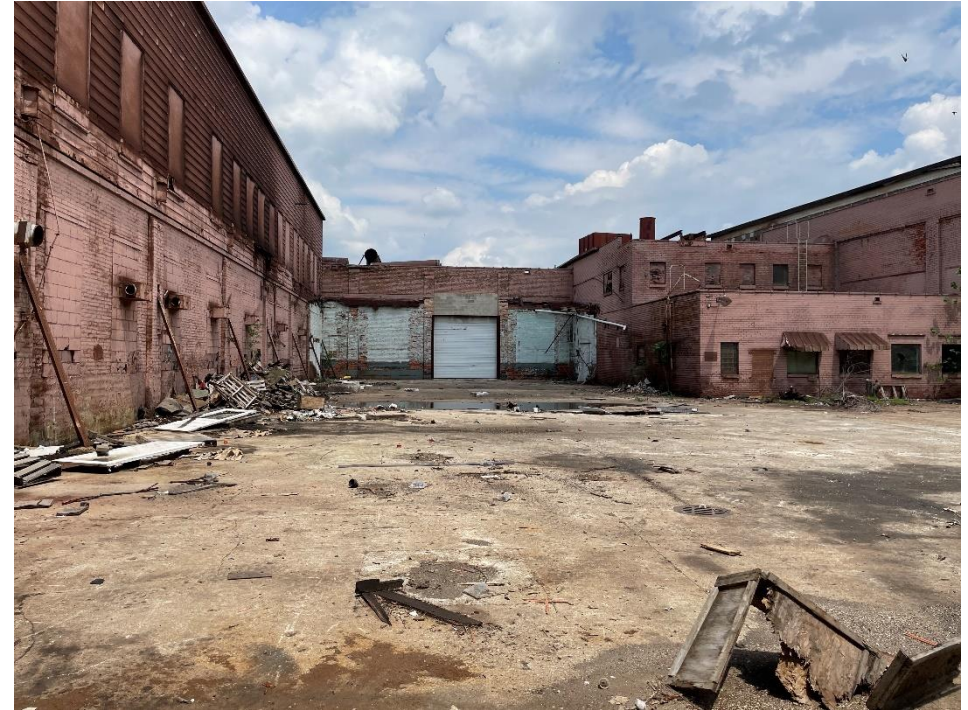
DATE: May 16, 2024 LOCATION: Former Dodge Manufacturing Company / Former RMG Foundry SUBJECT: View of the Former Dodge Manufacturing Company / Former RMG Foundry additions, looking north PHOTOGRAPHER: Robert R. Raduchel (Heartland) PHOTO: 6
