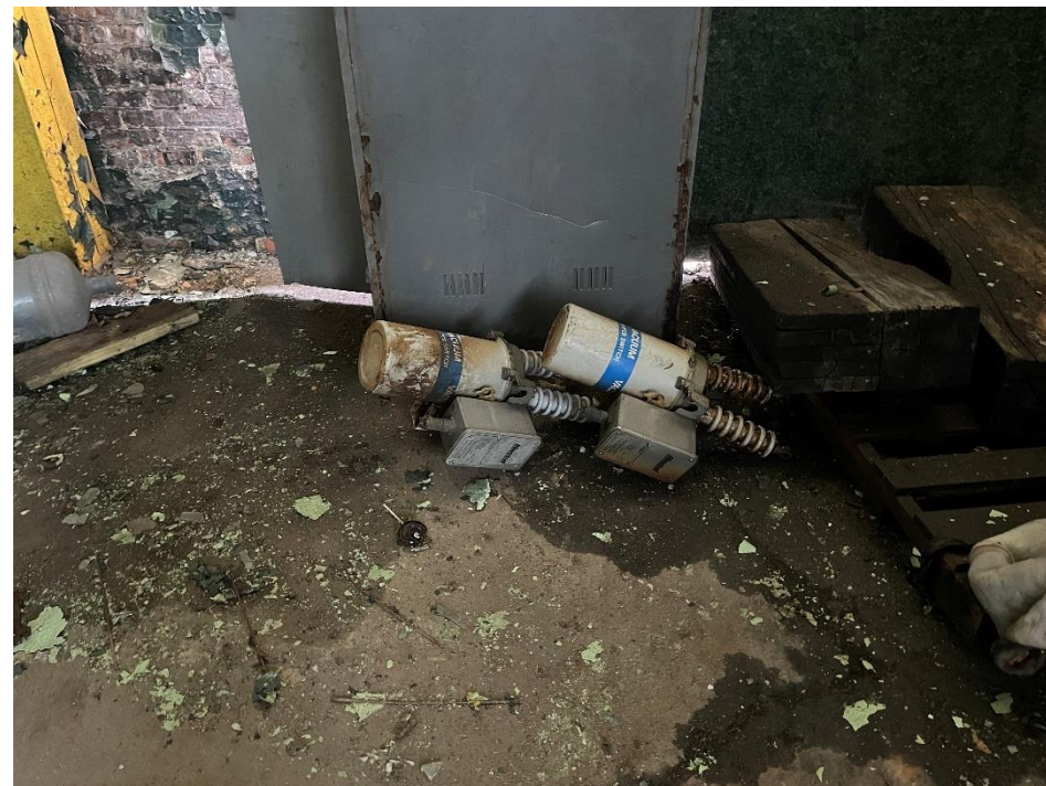
DATE: May 16, 2024 LOCATION: Former Dodge Manufacturing Company / Former RMG Foundry SUBJECT: View of non-PCB switches PHOTOGRAPHER: Robert R. Raduchel (Heartland) PHOTO: 20
