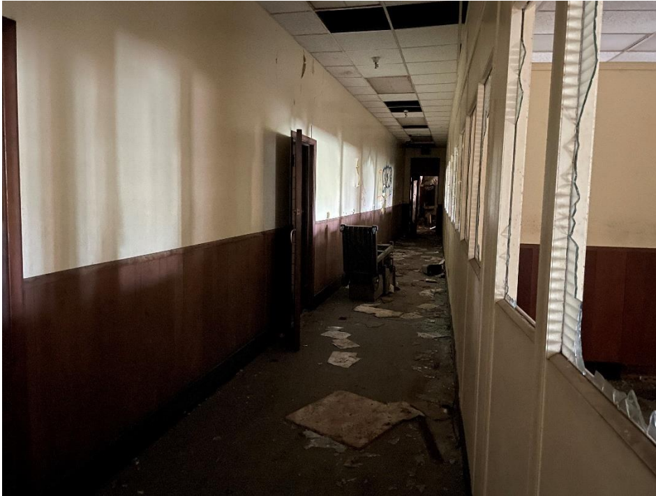
DATE: May 16, 2024 LOCATION: Former Dodge Manufacturing Company / Former RMG Foundry SUBJECT: Additional view of the second floor offices PHOTOGRAPHER: Robert R. Raduchel (Heartland) PHOTO: 49
