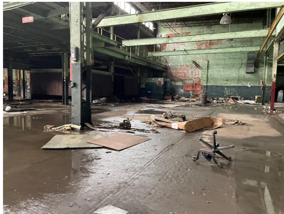
DATE: May 16, 2024 LOCATION: Former Dodge Manufacturing Company / Former RMG Foundry SUBJECT: View of the northwestern portion of the complex PHOTOGRAPHER: Robert R. Raduchel (Heartland) PHOTO: 44
