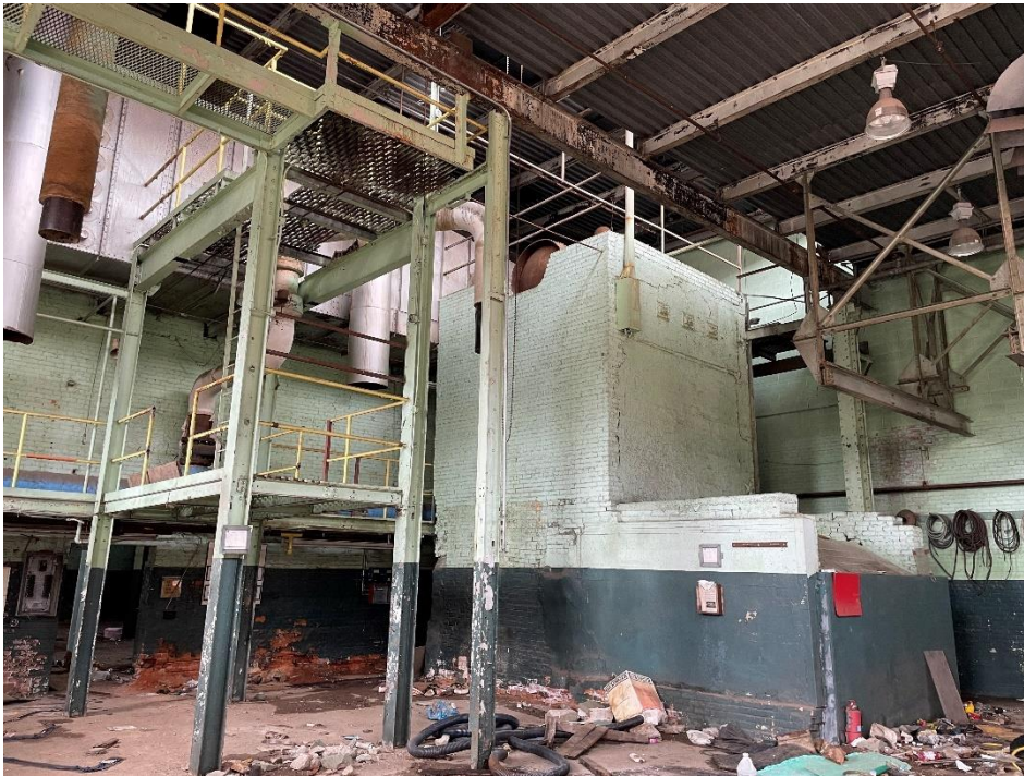
DATE: May 16, 2024 LOCATION: Former Dodge Manufacturing Company / Former RMG Foundry SUBJECT: View of bricked boiler in power house
