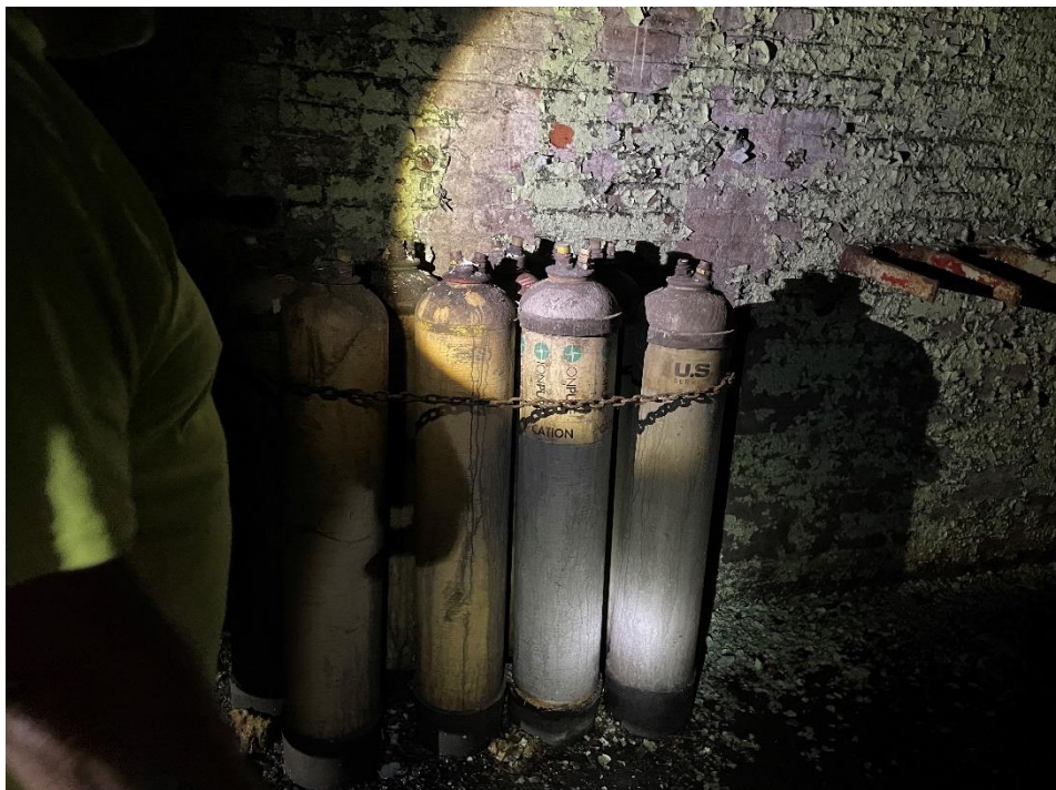
DATE: May 16, 2024 LOCATION: Former Dodge Manufacturing Company / Former RMG Foundry SUBJECT: View of water softening cartridges
