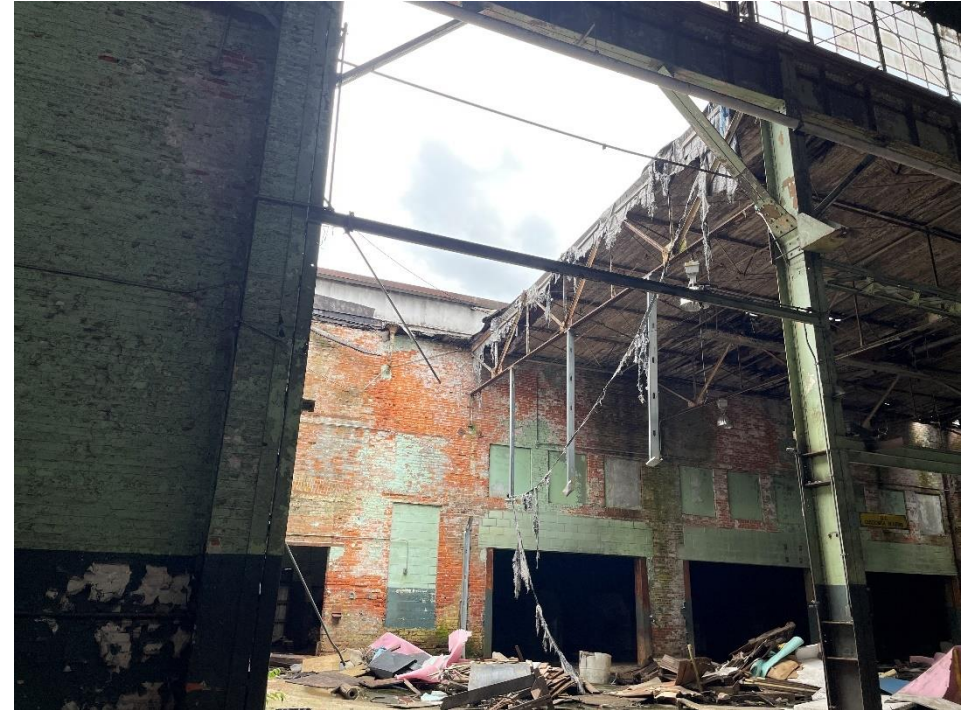
DATE: May 16, 2024 LOCATION: Former Dodge Manufacturing Company / Former RMG Foundry SUBJECT: View of missing roof section in western portion of the complex PHOTOGRAPHER: Robert R. Raduchel (Heartland) PHOTO: 50
