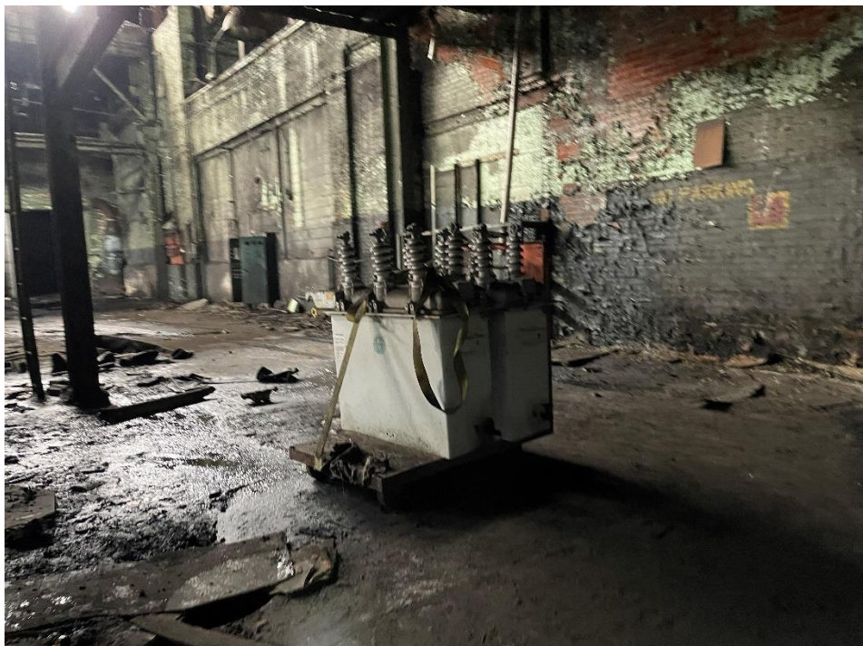
DATE: May 16, 2024 LOCATION: Former Dodge Manufacturing Company / Former RMG Foundry SUBJECT: View of additional electrical infrastructure equipment
