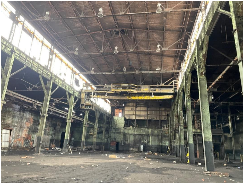
DATE: May 16, 2024 LOCATION: Former Dodge Manufacturing Company / Former RMG Foundry SUBJECT: View of the gantry crane on northern portion of the complex PHOTOGRAPHER: Robert R. Raduchel (Heartland) PHOTO: 71
