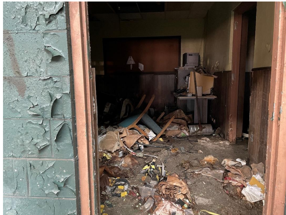
DATE: May 16, 2024 LOCATION: Former Dodge Manufacturing Company / Former RMG Foundry SUBJECT: View of the office and mold in southern portion of the complex PHOTOGRAPHER: Robert R. Raduchel (Heartland) PHOTO: 18
