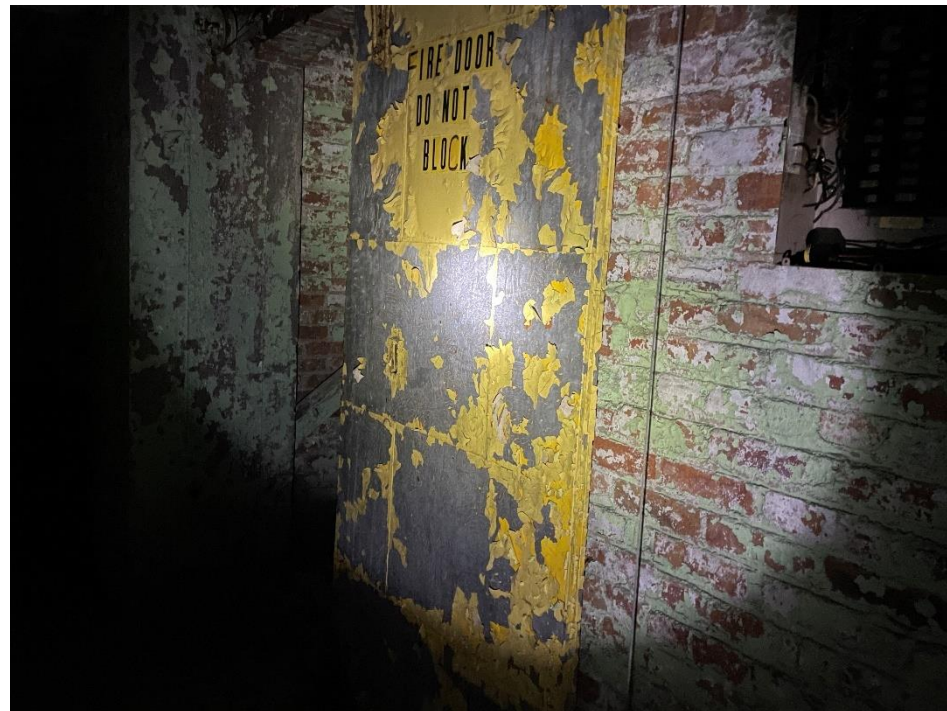
DATE: May 16, 2024 LOCATION: Former Dodge Manufacturing Company / Former RMG Foundry SUBJECT: View of fire door in basement of the southeastern portion of the complex
