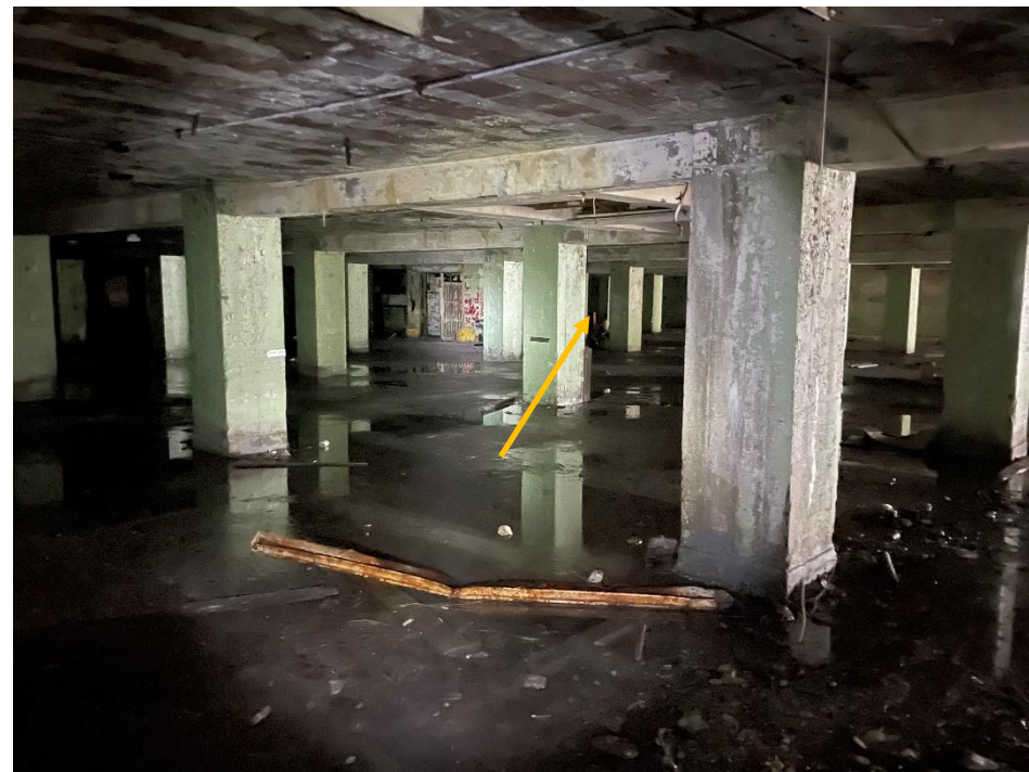
DATE: May 16, 2024 LOCATION: Former Dodge Manufacturing Company / Former RMG Foundry SUBJECT: View of the basement under southeastern portion of the complex PHOTOGRAPHER: Robert R. Raduchel (Heartland) PHOTO: 22
