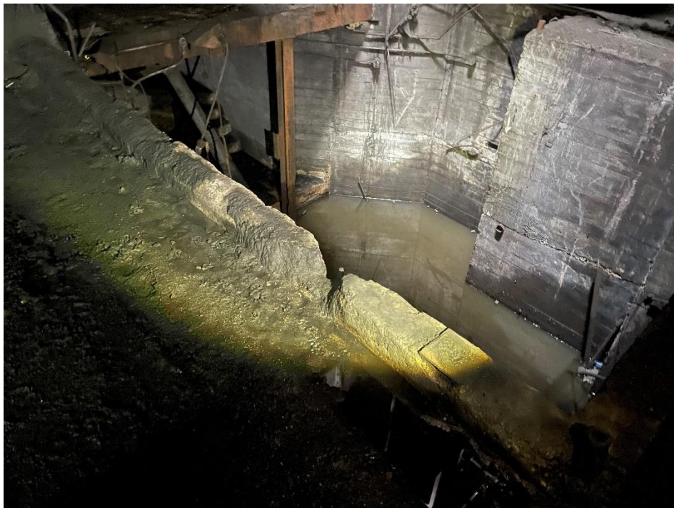
DATE: May 16, 2024 LOCATION: Former Dodge Manufacturing Company / Former RMG Foundry SUBJECT: View of former sand pit in northern portion of the complex PHOTOGRAPHER: Robert R. Raduchel (Heartland) PHOTO: 51
