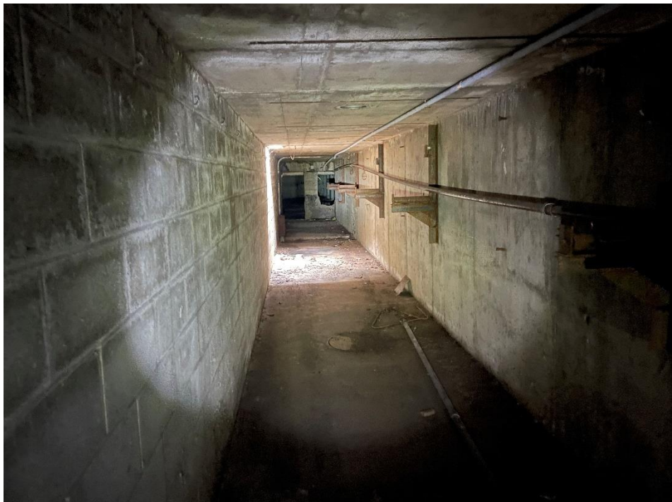
DATE: May 16, 2024 LOCATION: Former Dodge Manufacturing Company / Former RMG Foundry SUBJECT: View of pipe chase leading east from the southeastern basement PHOTOGRAPHER: Robert R. Raduchel (Heartland) PHOTO: 25
