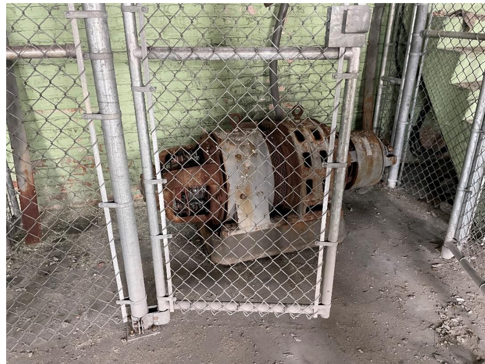
DATE: May 16, 2024 LOCATION: Former Dodge Manufacturing Company / Former RMG Foundry SUBJECT: View of DC motor in southeastern portion of the complex PHOTOGRAPHER: Robert R. Raduchel (Heartland) PHOTO: 36
