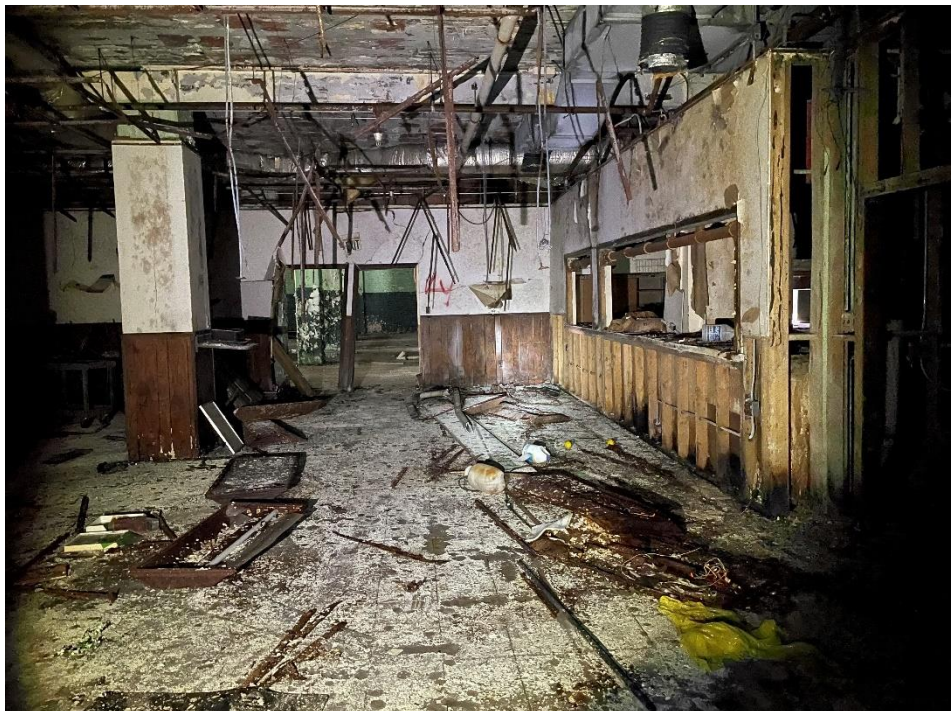
DATE: May 16, 2024 LOCATION: Former Dodge Manufacturing Company / Former RMG Foundry SUBJECT: View of the cafeteria in southeastern portion of the complex PHOTOGRAPHER: Robert R. Raduchel (Heartland) PHOTO: 27
