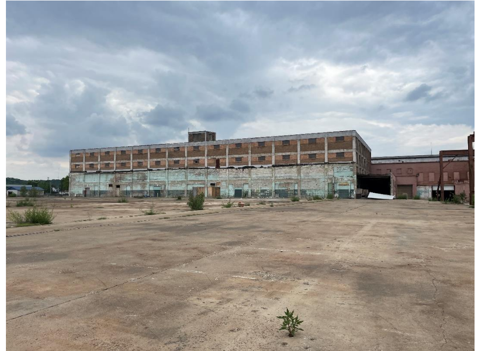
DATE: May 16, 2024 LOCATION: Former Dodge Manufacturing Company / Former RMG Foundry SUBJECT: View of the foundation of the burned southeastern portion of the complex, looking east
