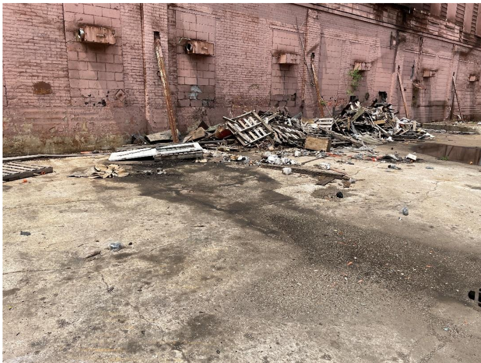
DATE: May 16, 2024 LOCATION: Former Dodge Manufacturing Company / Former RMG Foundry SUBJECT: View of stained concrete west of the foundry sand silo (AST) PHOTOGRAPHER: Robert R. Raduchel (Heartland) PHOTO: 11
