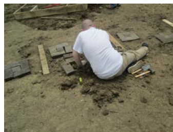
Students helped design and install the pathway for the students, staff, volunteers, and visitors to enjoy.
