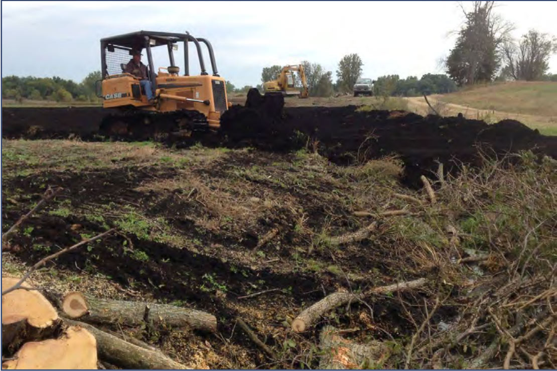
Ditch closure using a wide-tracked bulldozer to push muck soil. Felled ditch-side trees and brush served as a more stable foundation upon which the bulldozer could operate without sinking.
