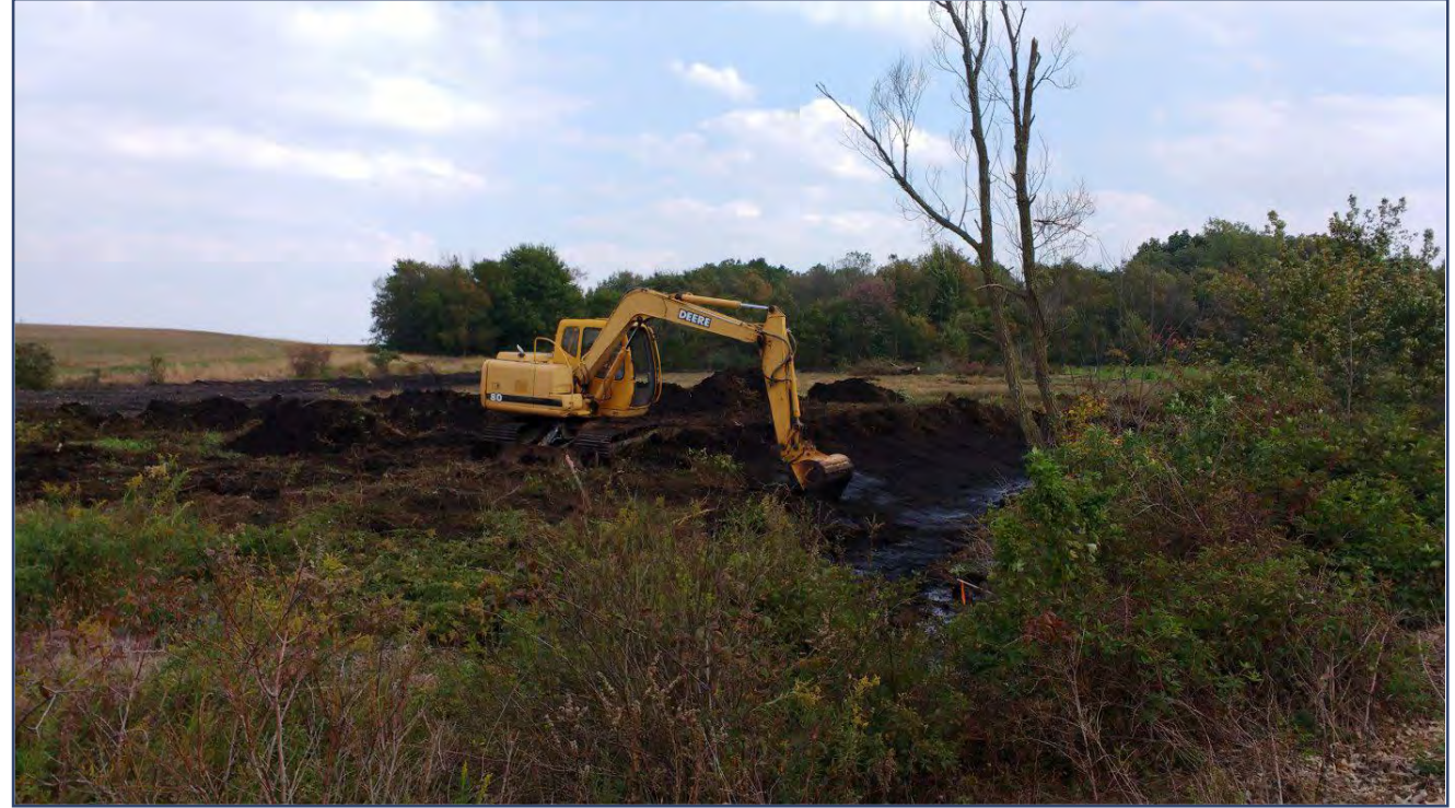
Stream meander creation using a tracked excavator. The steep-sided ditch banks were pulled back and the channel bottom was reconfigured with pools and riffles to create a natural stream course.
