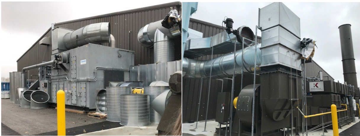
VOC concentrators with natural gas-fired thermal oxidizers
