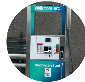
Hydrogen refueling station
