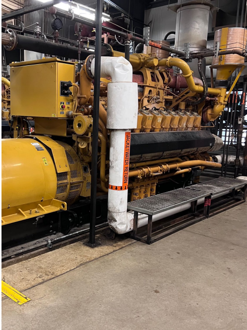
Existing 1600KW LFG Generator Source for Heat Recovery Skids.
