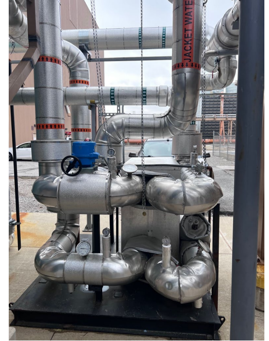
New Jacket Water (225F) Heat Recovery Skids – 650 GPM
