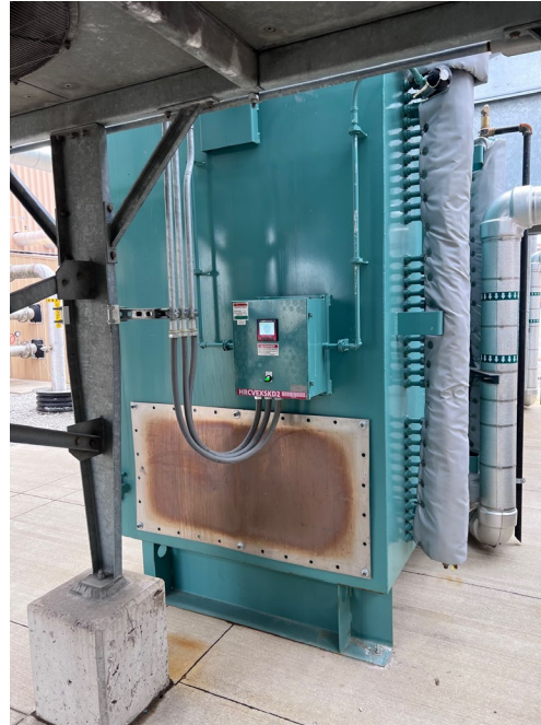
New Exhaust Heat Recovery Skids Exhaust (1000F) to water (220F) heat exchanger – 650 GPM
