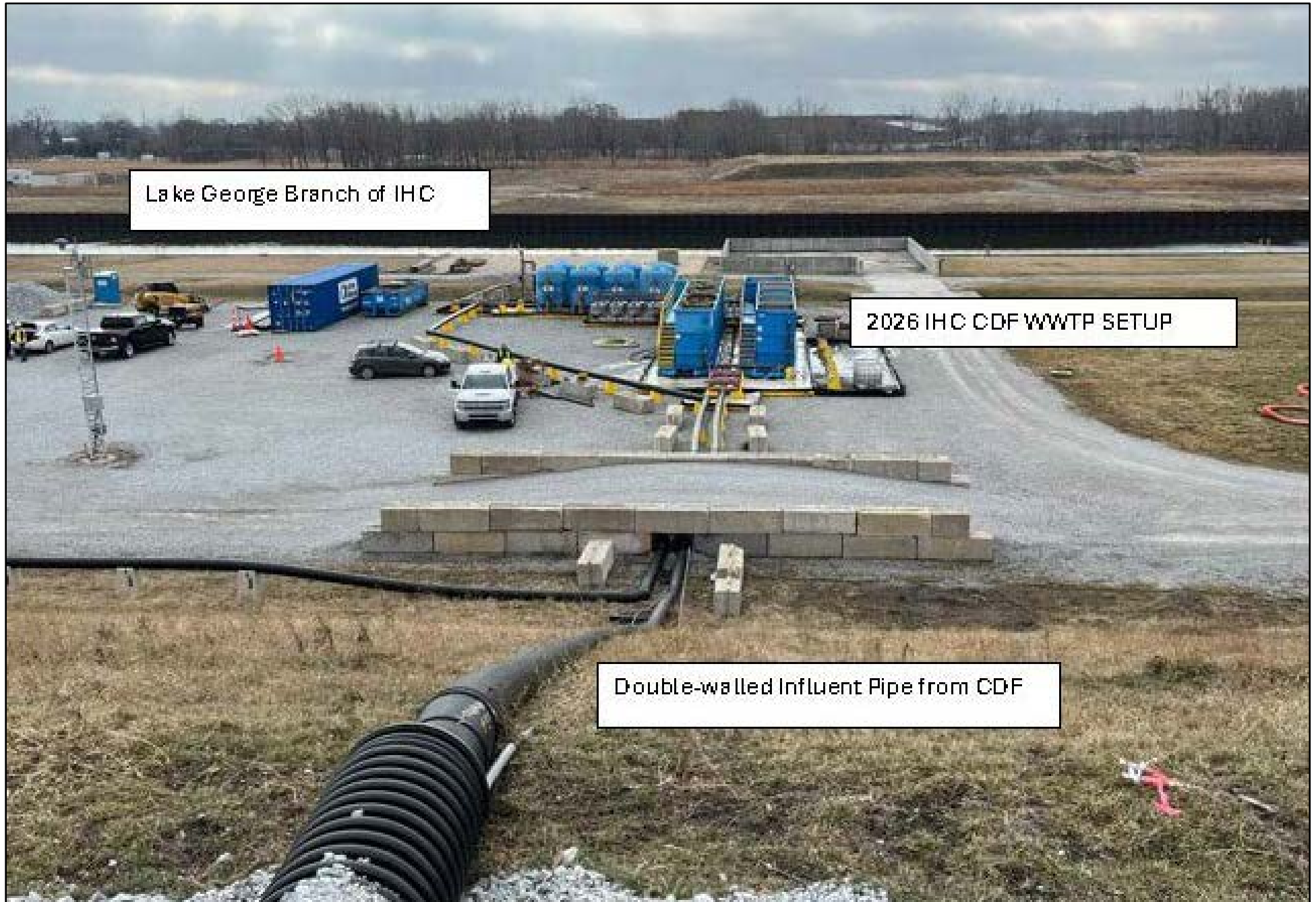
Figure 5 – Package Wastewater Treatment Plant
