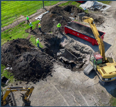
Regulated tanks that do not meet requirements must be properly closed or upgraded.
