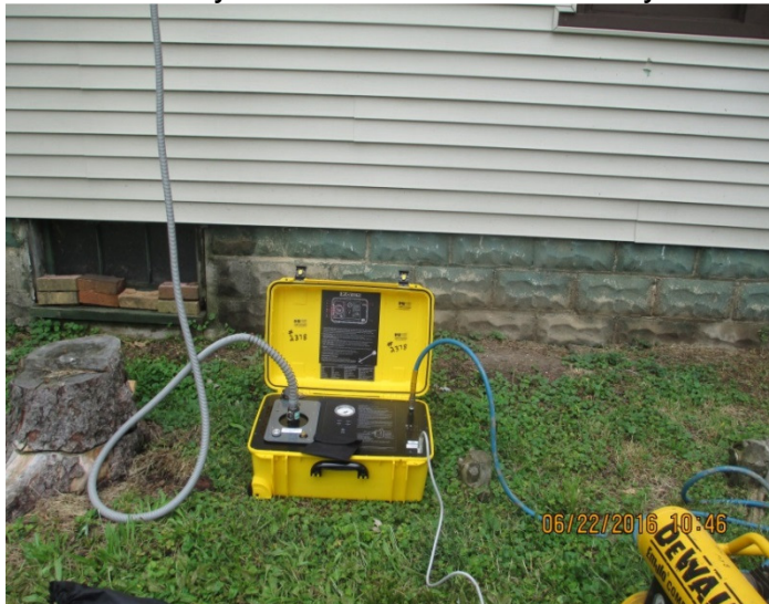
Figure 1. Compressor and smoke generator with attachment going to the roof vent.
