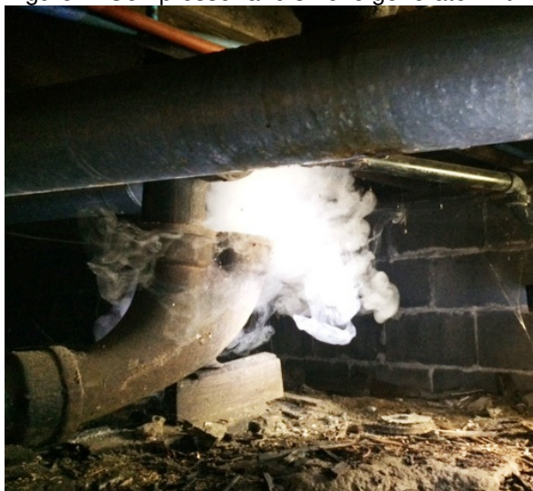
Figure 2. Visual observation of smoke at a potential sewer gas leak.
